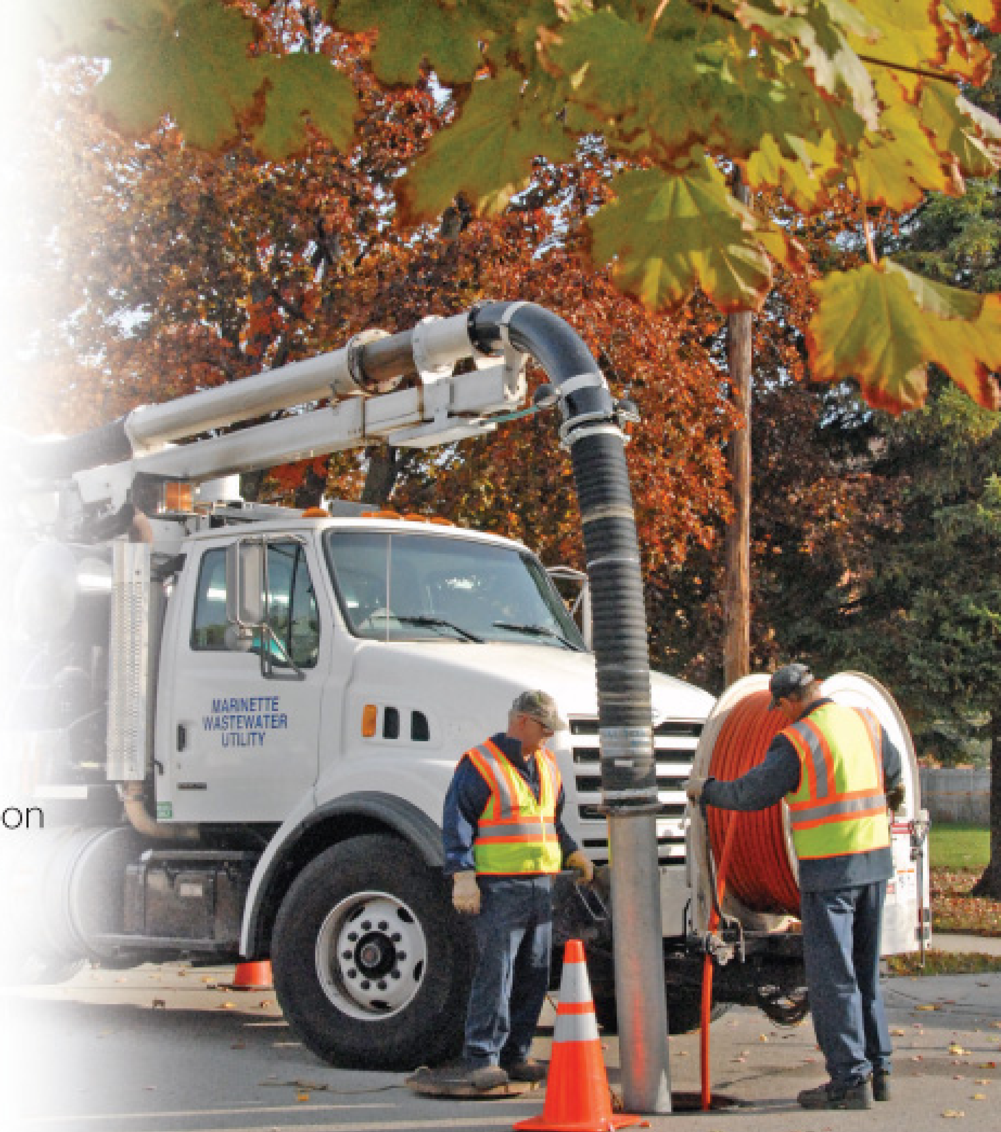
Roger Keller (left) and Gary Kmieciak operate the jetter on Marinette's Vactor 2100 truck in preparation for a video inspection of a sewer. (Photos by Jim Kneiszel)
