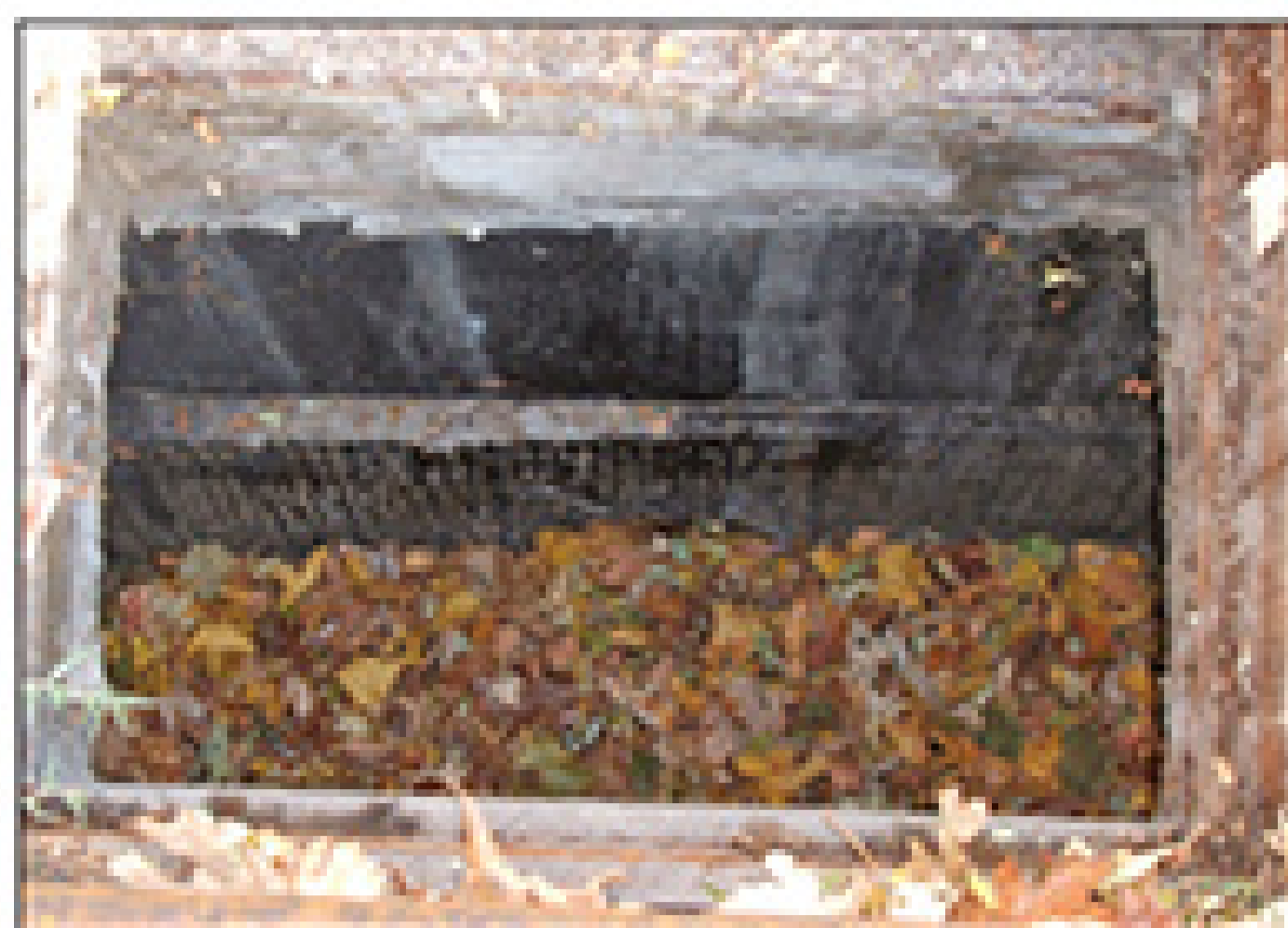
Left, dry leaves fill a catch basin, piled nearly to the top of the entry to the storm sewer pipe that runs under the street. Below, a crew member uses a water hose to loosen debris inside the basin.
