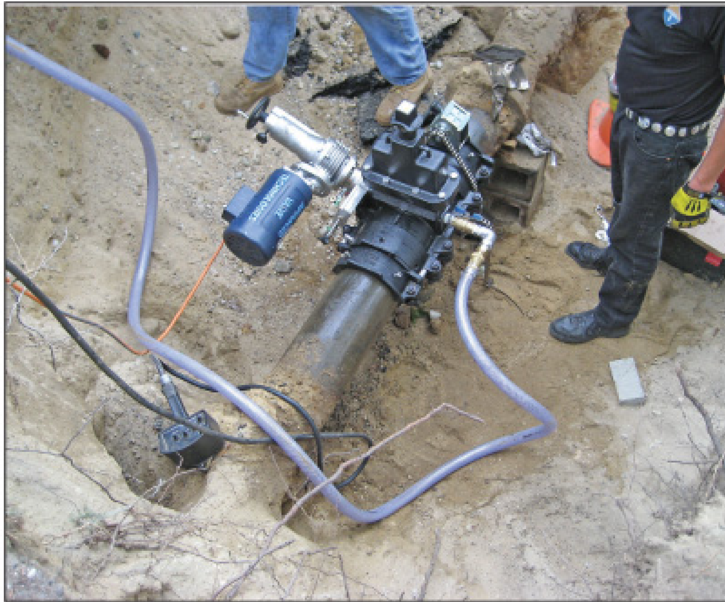
An exit hose removed metal chips during cutting of the valve opening. This keeps chips from traveling downstream and potentially clogging meters and services.
