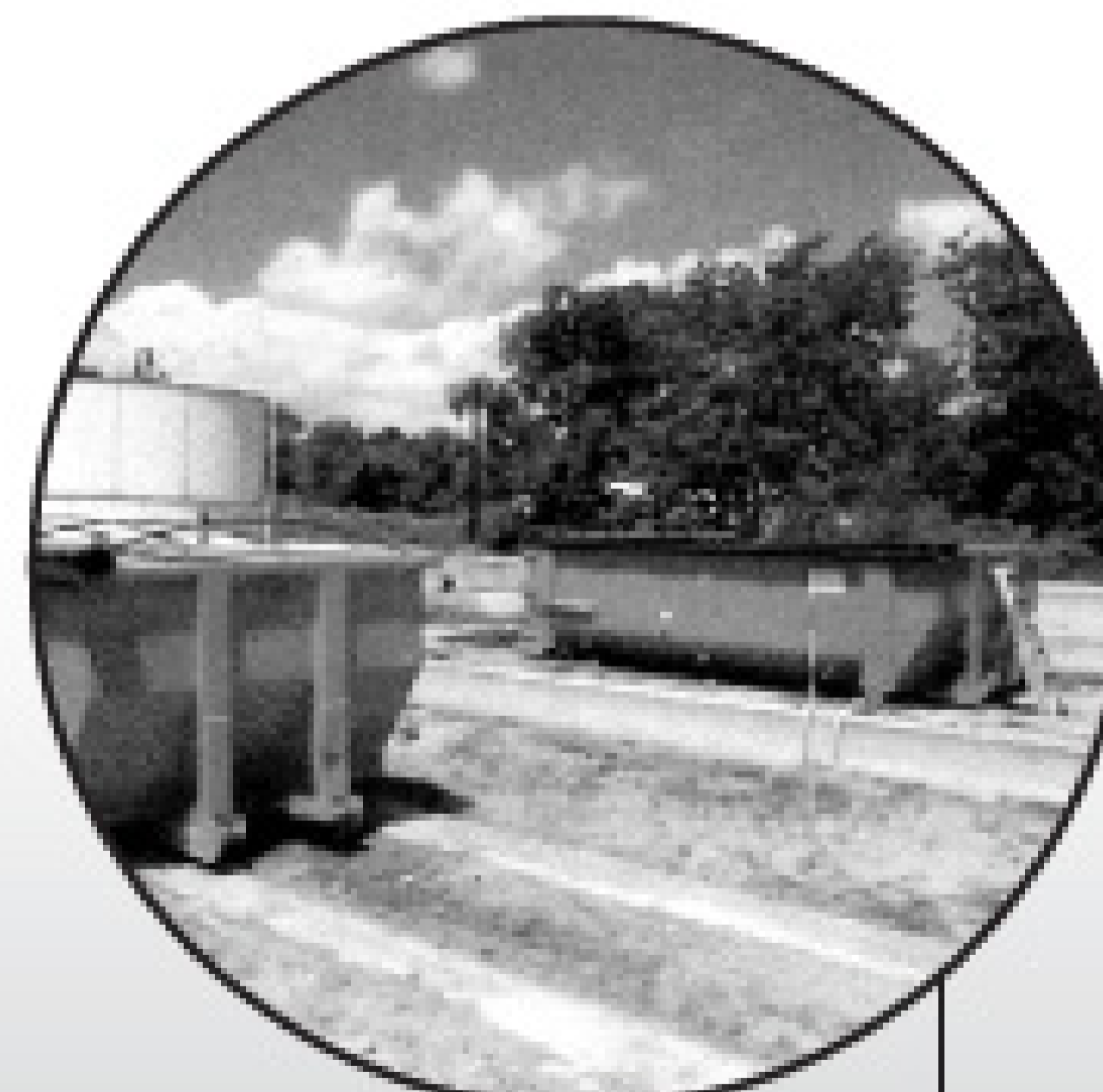
Concrete runners installed in existing drying beds for placement of roll-off dewatering box.
