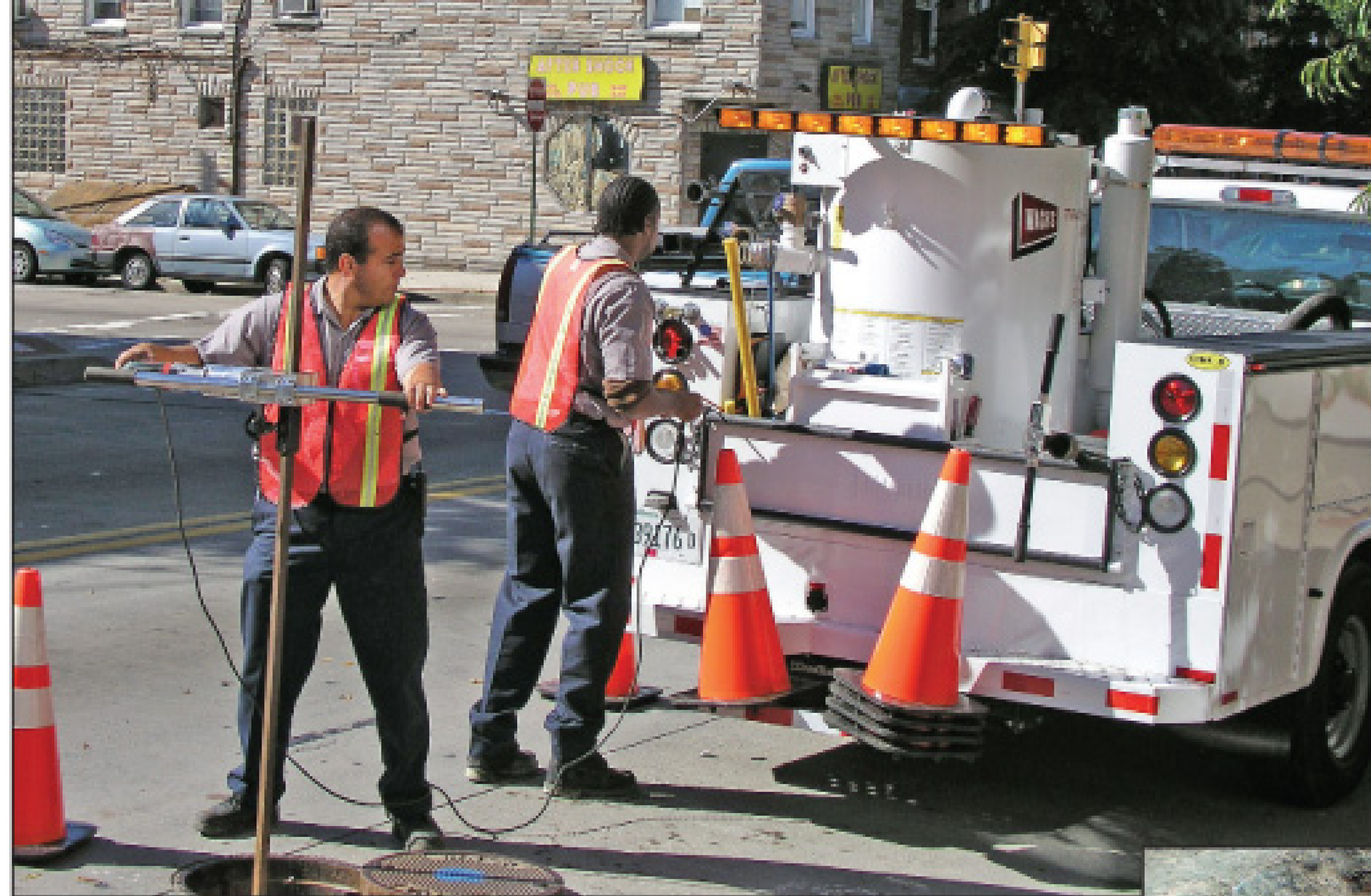
A Wachs Utility Services crew operates a valve with a hand-held electric turner after accessing and cleaning debris out of the valve box with the Wachs Travl-Vac 300.
