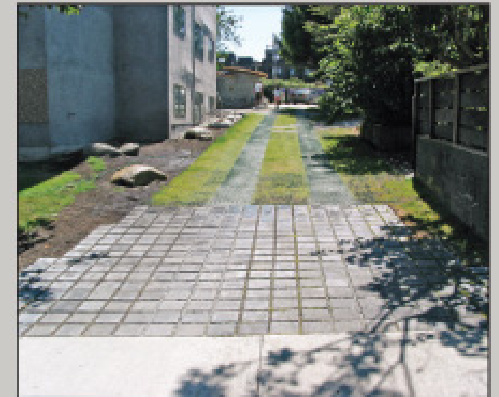
At Farmers Country Lane, designers used interlocking paver blocks for support where driveways entered alleys, or in areas with heavy utility truck traffic.
