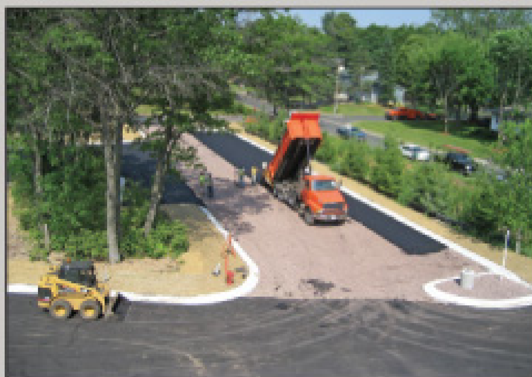
A rooftop view of porous asphalt placement. Soil behind the curb lines is stabilized with erosion control blanketing.
