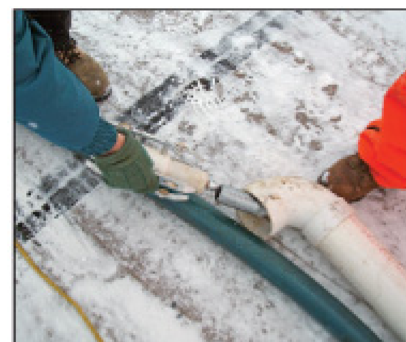
The inspection crew used duct tape to attach the sonde to a camera cable. The sonde is more typically attached to a sewer-cleaning cable.
