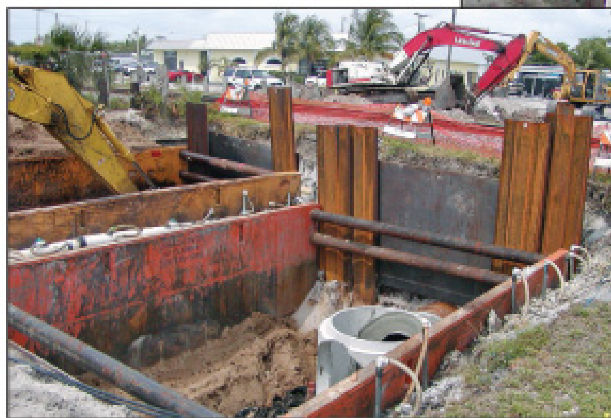
A double jack-and-bore operation: stormwater on the right, water main on the left. (Photo courtesy of City of Boynnton Beach Utilities Department)
