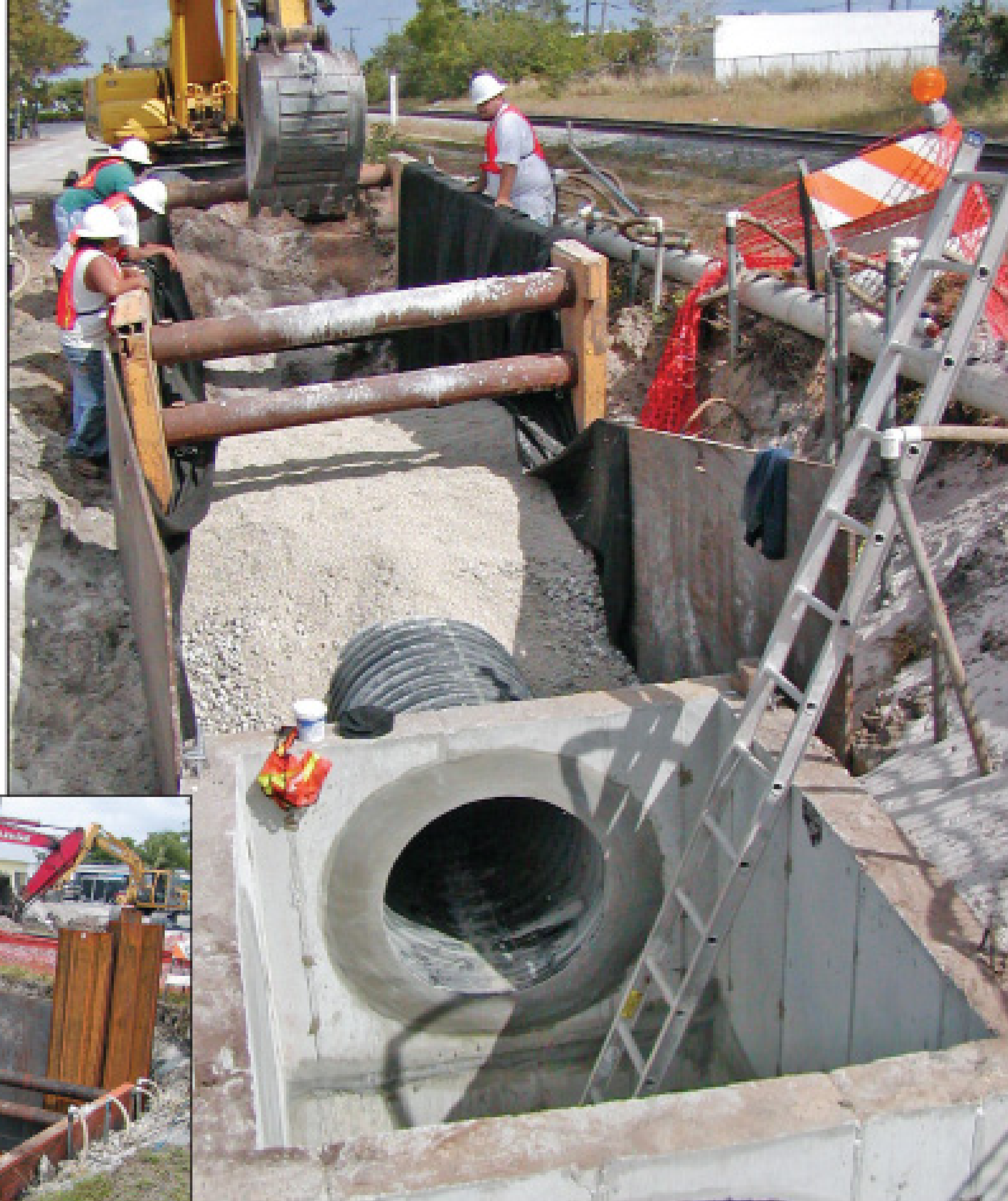
Boynnton Beach workers install a drainage structure and exfiltration trench. (Photo courtesy of City of Boynnton Beach Utilities Department)
