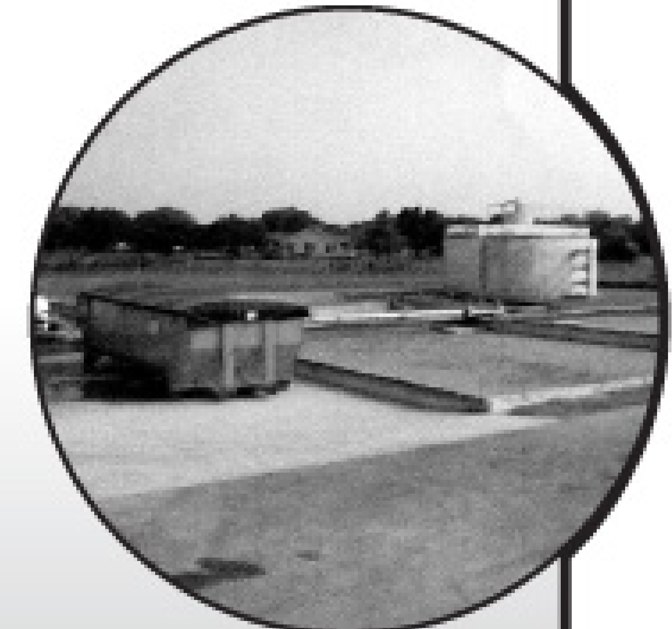
One of six drying beds converted to concrete to accommodate entire dewatering system.
