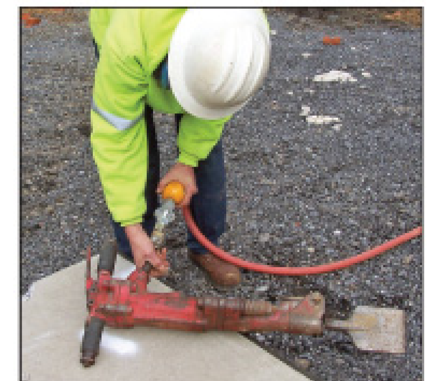
King connects the compressed air system to a jackhammer.
