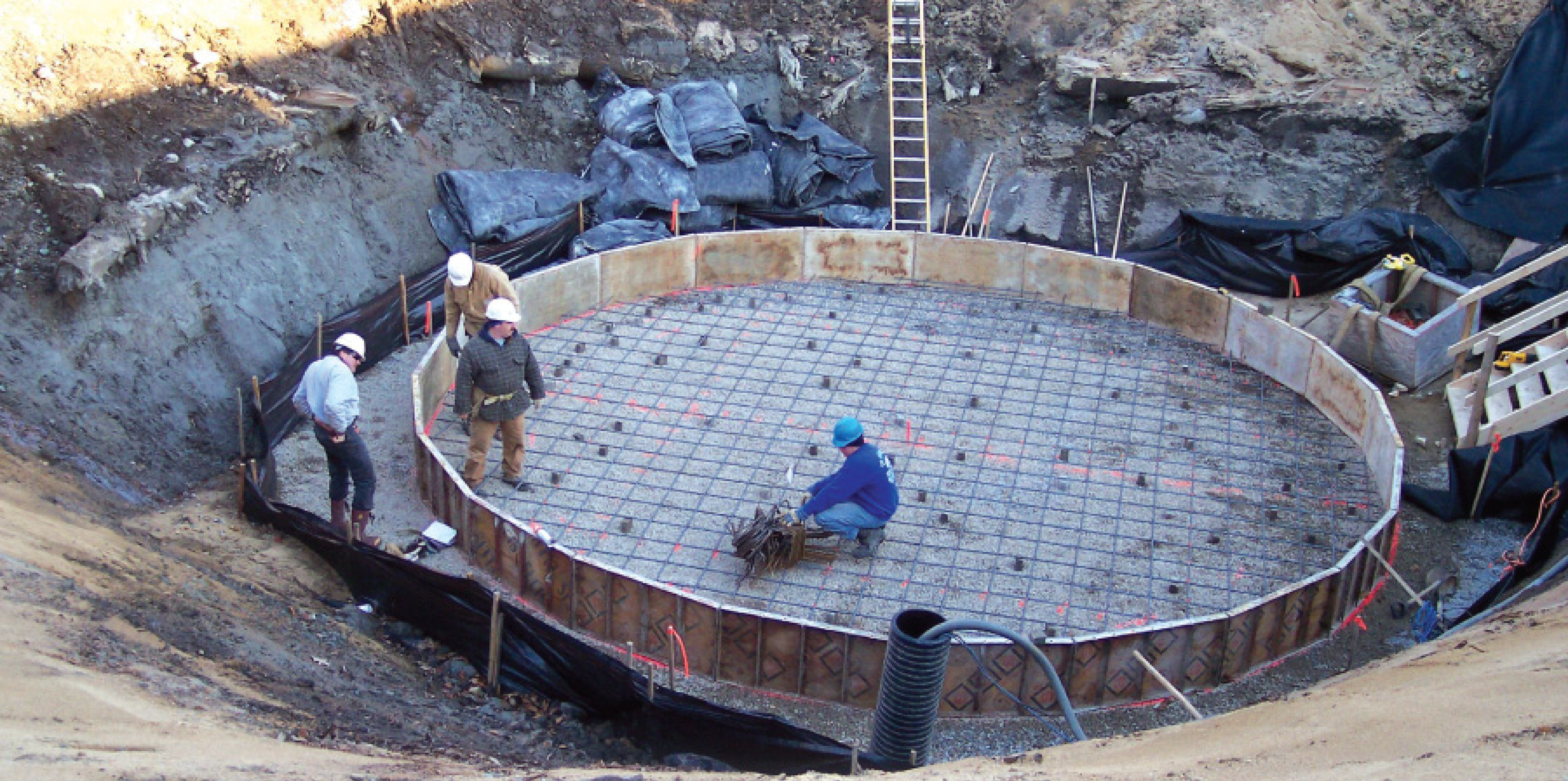
Initial construction of the CSO Storm King. (Photo courtesy of Saco WWTP)
