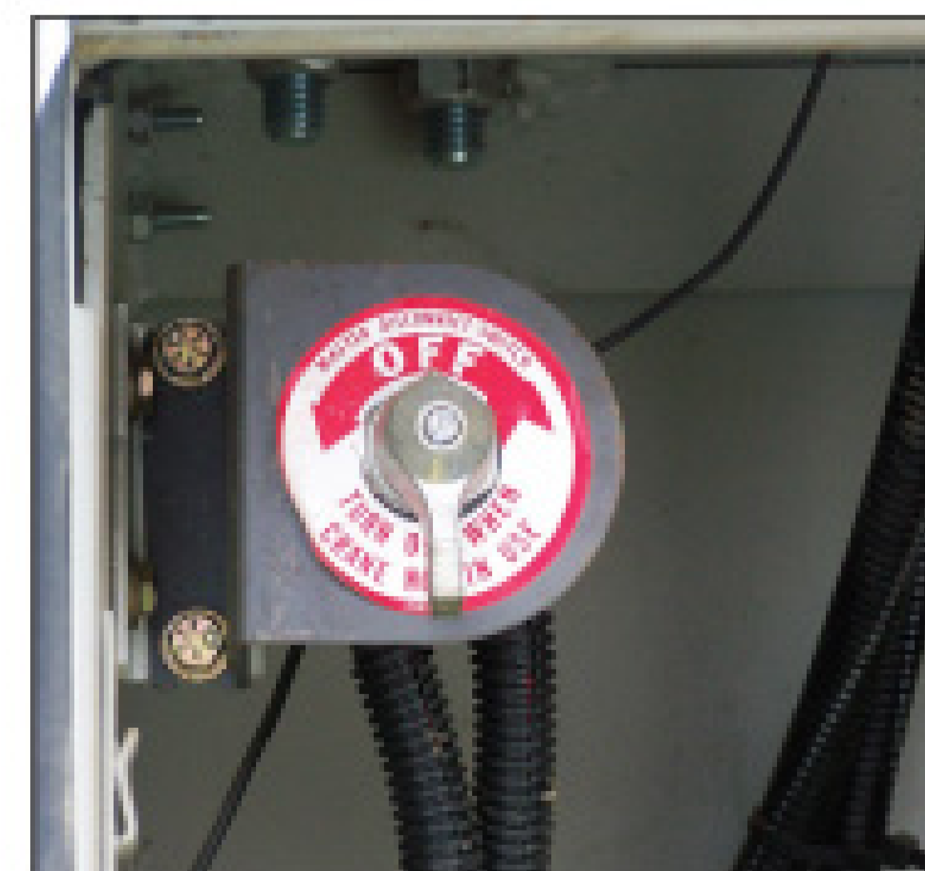
The crane's master disconnect switch protects the equipment from unauthorized use.
