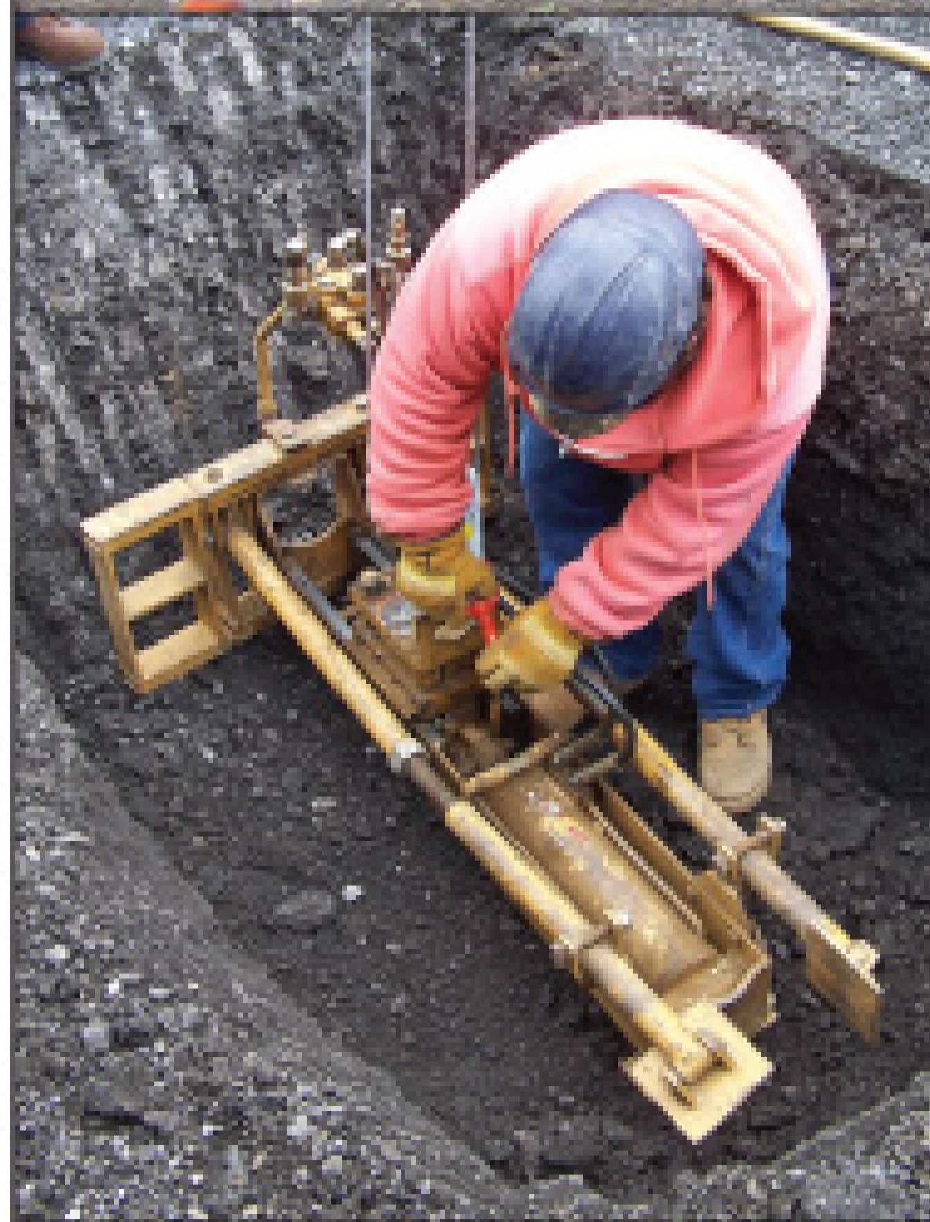
Crew member Tom Haddad readies a McLaughlin hydraulic ram, used to drive a rod under an obstruction (like a road) as part of a replacement pipe insertion project.
