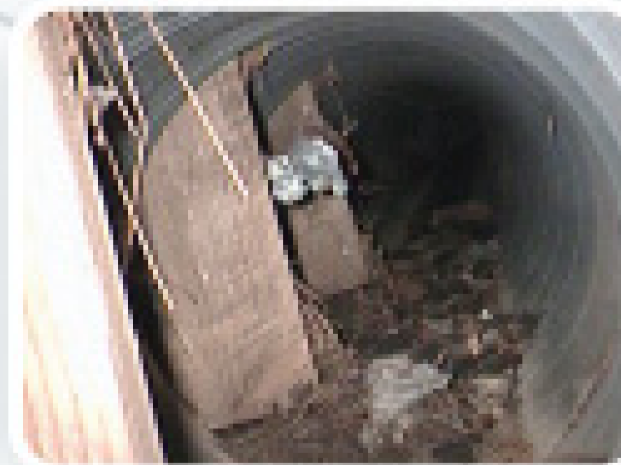
Fence Post Breach
