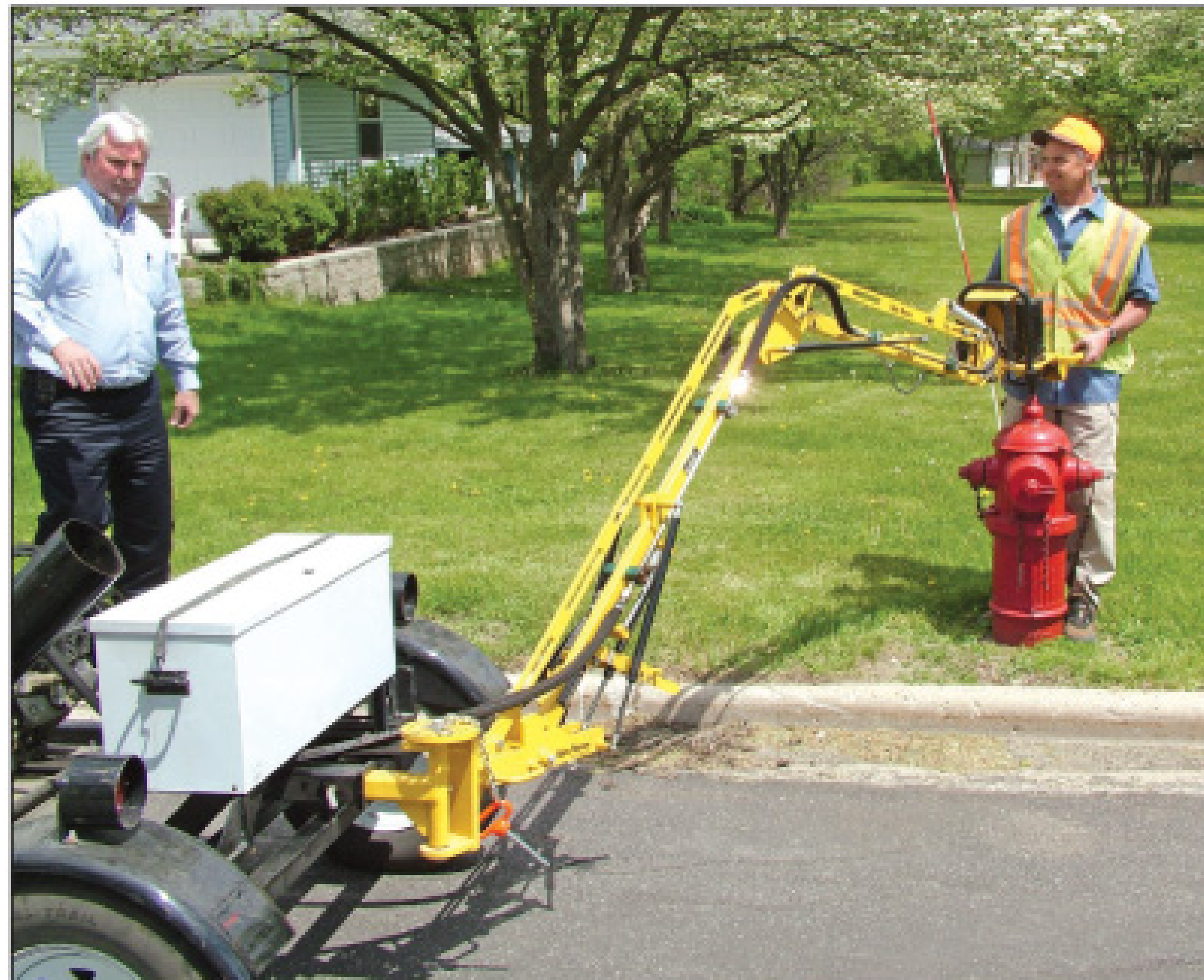
Utility maintenance technician Louie Thon demonstrates how the Spin Doctor unit's jointed arm provides reach that can enable exercising of more than one valve without repositioning the trailer.
