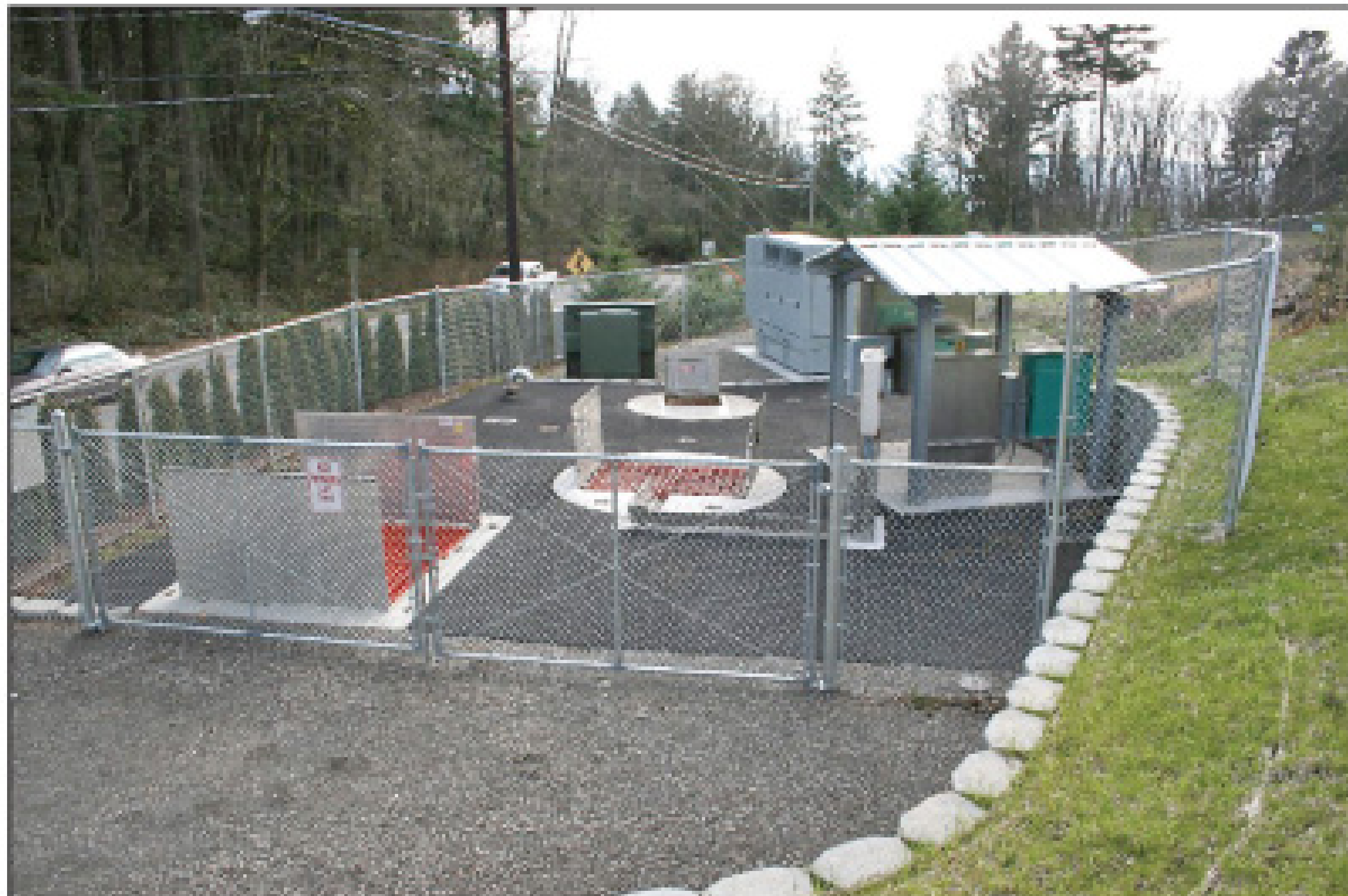
The new Brady Road wastewater lift station uses a complete system design from Romtec Utilities Inc. that has helped the City of Camas standardize its lift station network.
