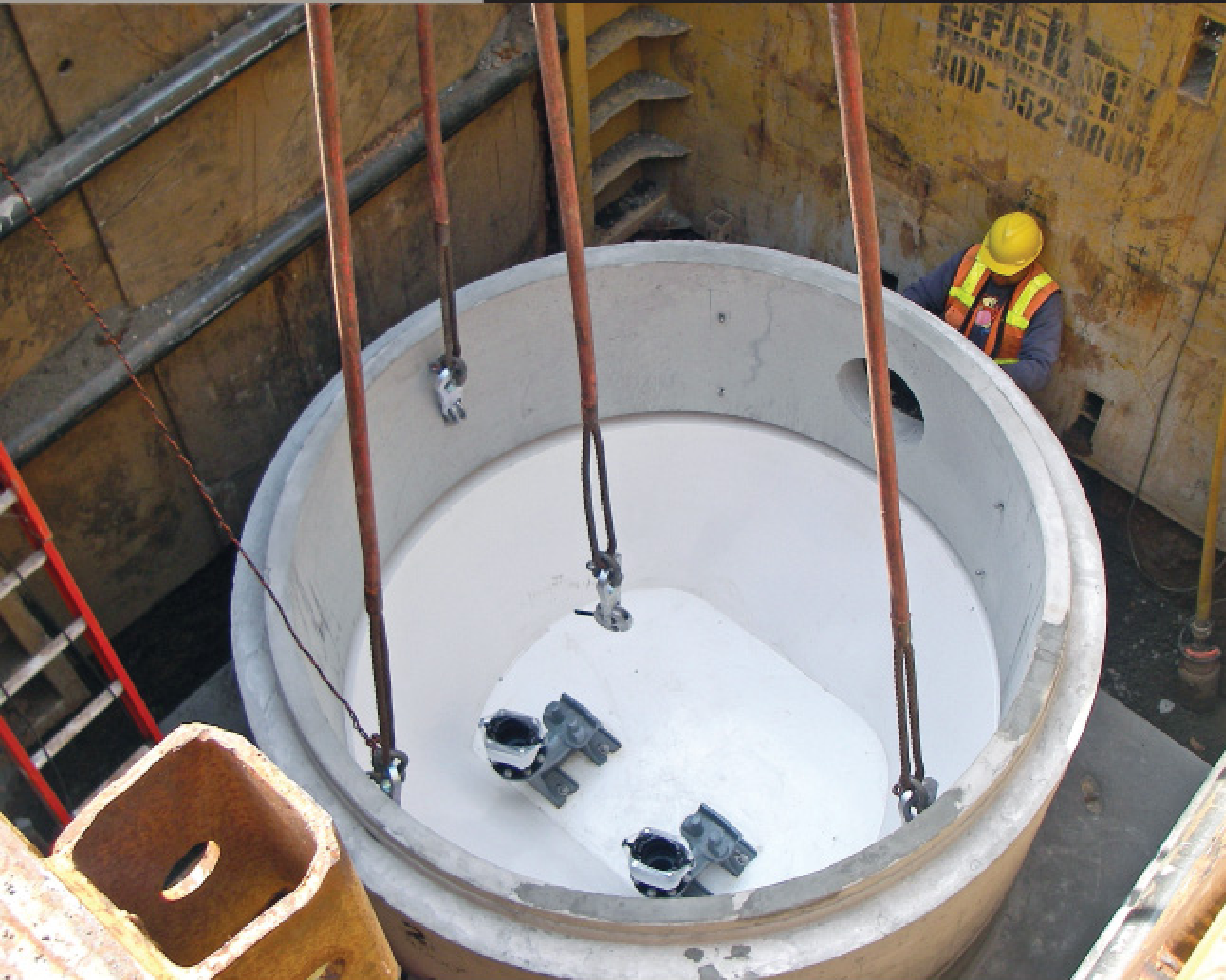
A worker from George Schmid & Sons readies the wet well base for installation.
