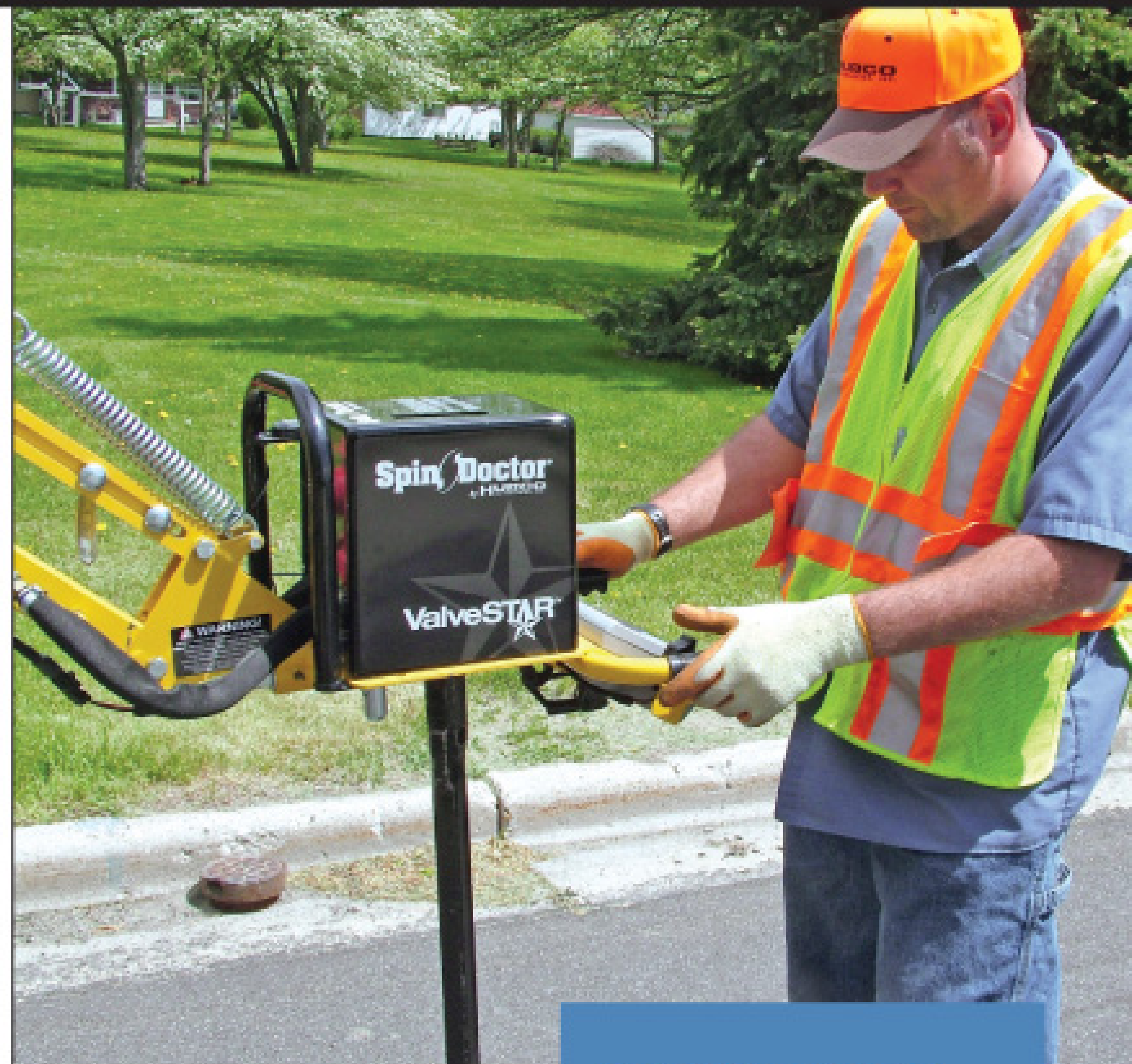
Utility maintenance technician Troy Bacon operates the Spin Doctor unit with Valve Star head. The joystick at his left thumb activates valve closing and opening.
