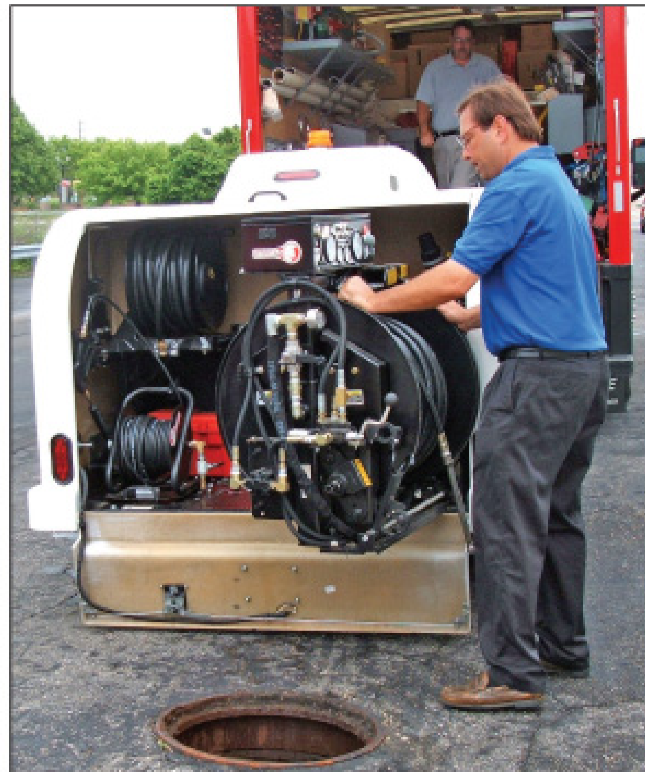
Spartan Tool president Tom Pranka maneuvers the jetter hose reel out from its resting place. Besides the jetting hose, the unit carries an auxiliary hose (lower left) that feeds a wash-down nozzle or can be used to jet in more limited spaces; and a hose for filling the tank (upper left).
