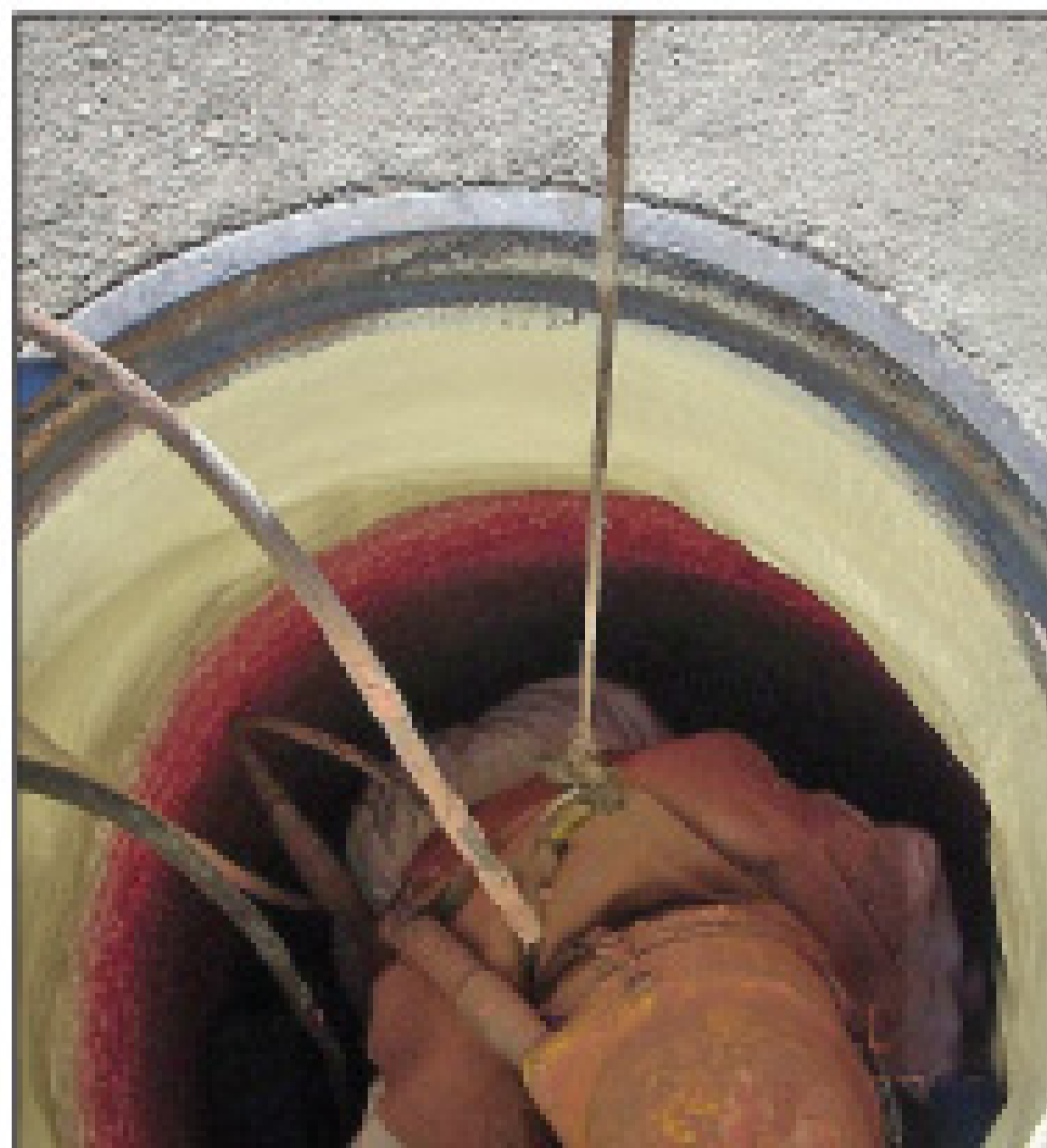
The corrosion barrier was applied by a technician fully equipped for confined-space entry.
