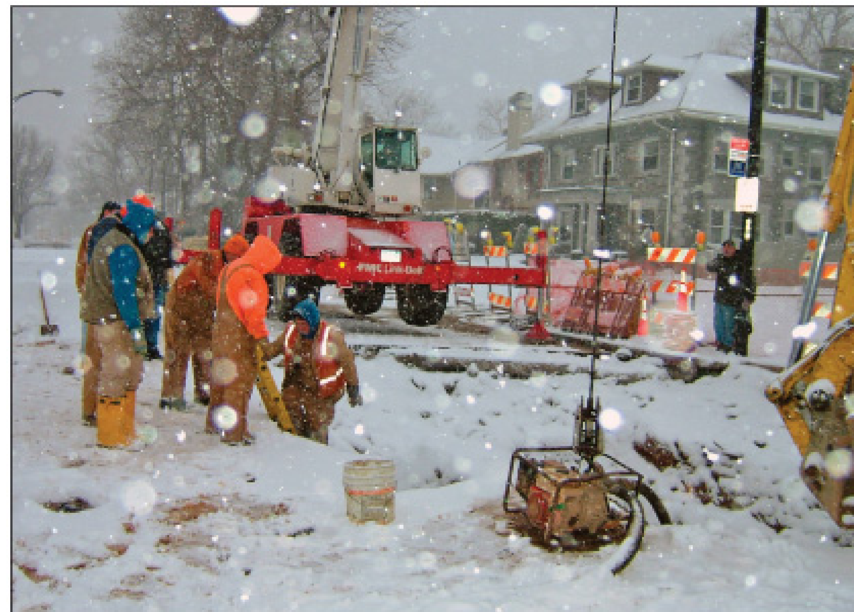
Buffalo's typically heavy snowfall creates an extra level of difficulty in repairing midwinter main breaks. (Photos by Peter Kenter)
