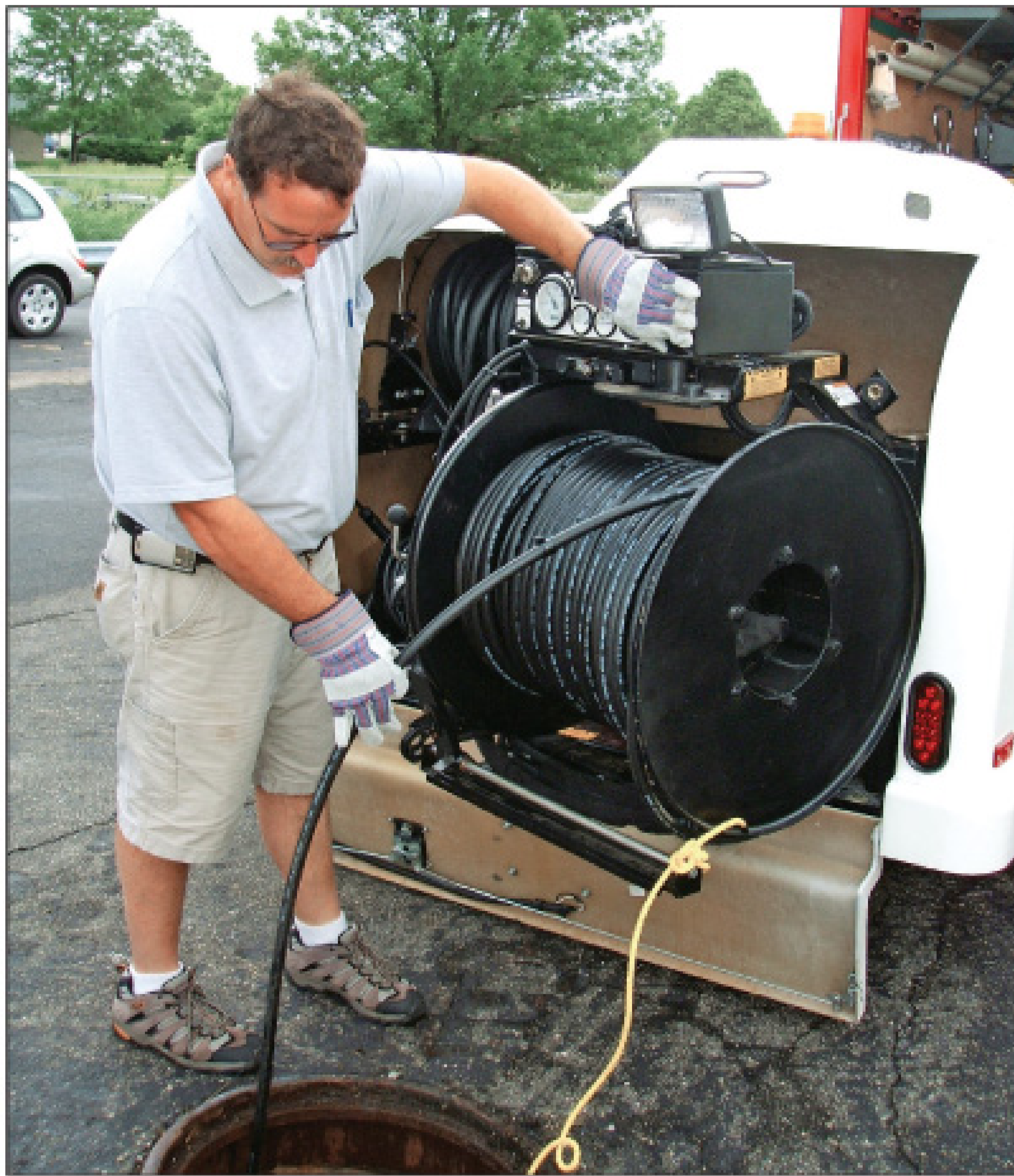
Brian Willis, Spartan Tool territory sales manager, feeds the jetter hose into a manhole.
