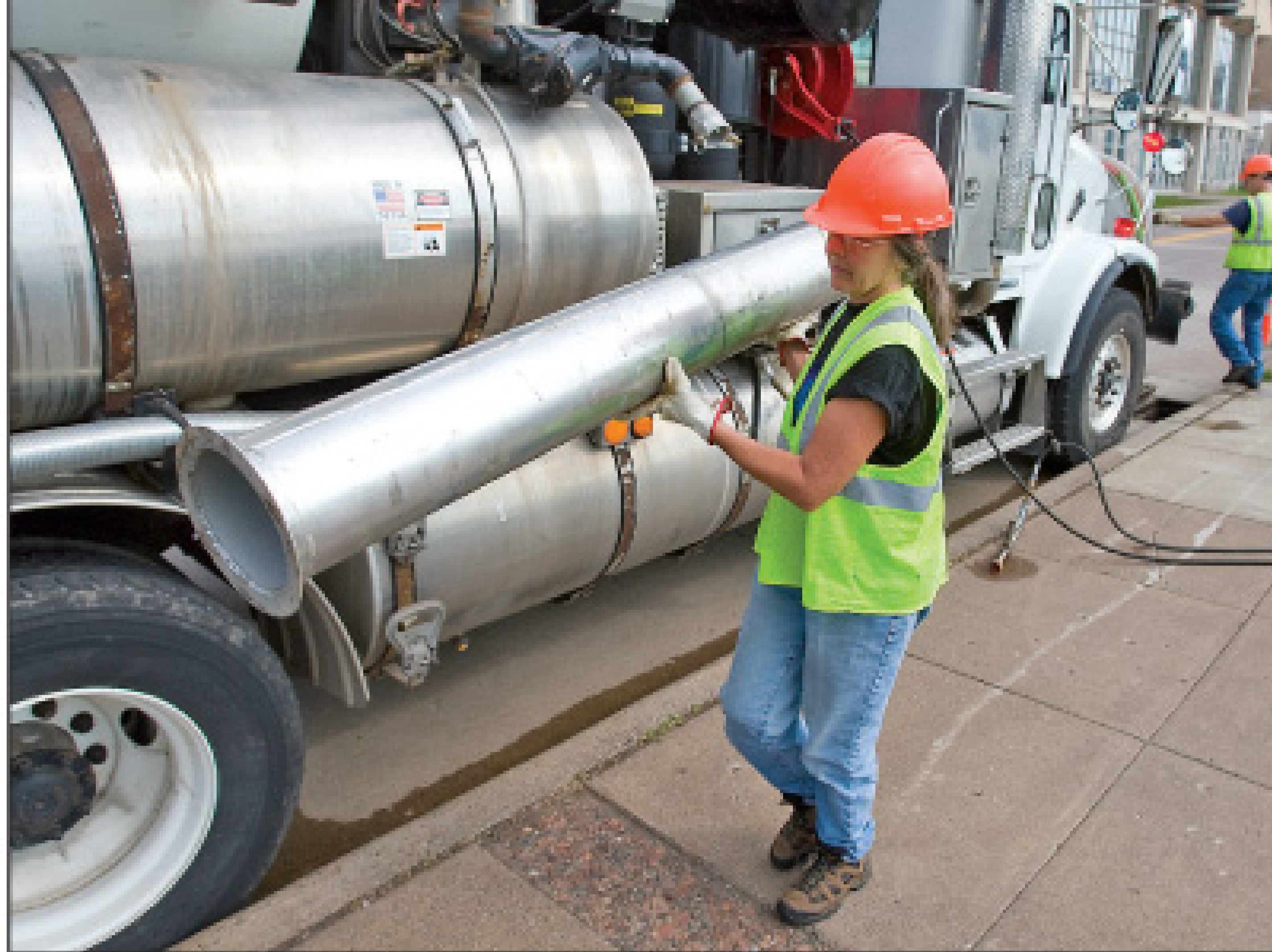
Hutchinson prepares for a job using a Vactor 2100 truck, one of four the city uses to clean storm drains and more than 9,000 catch basins.
