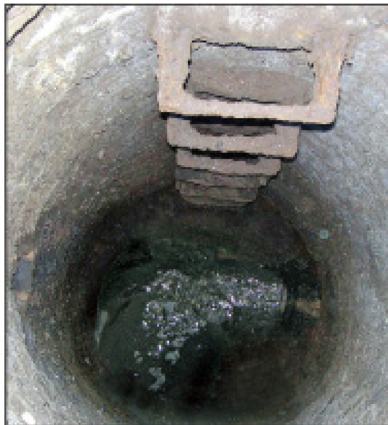
Three manholes had steel stairs so badly corroded that they fell off when hit with a hammer. Note water infiltration.
