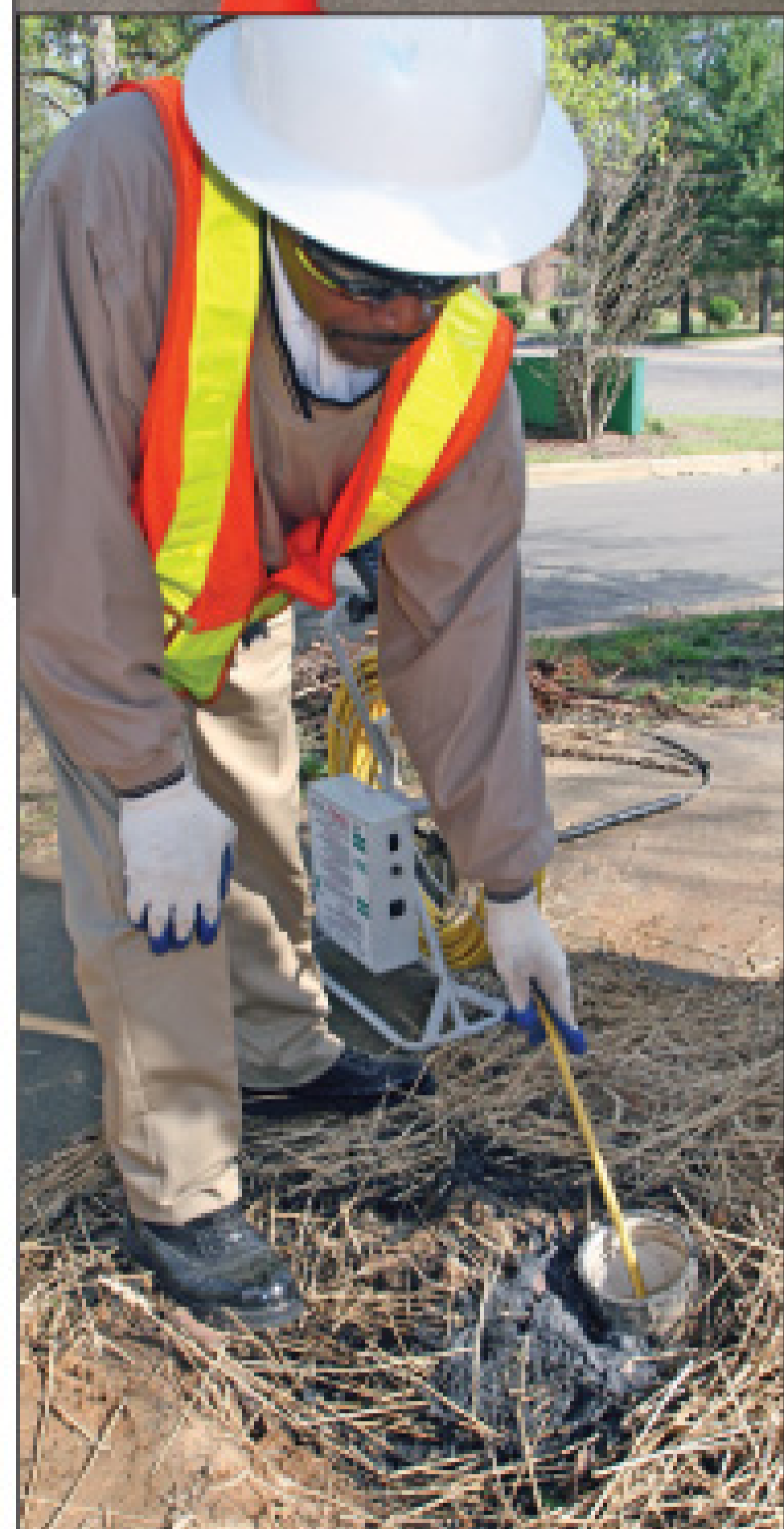
Donald Barnes uses a CCTV rig to inspect a service line along the region's 2,300-mile collection system.
