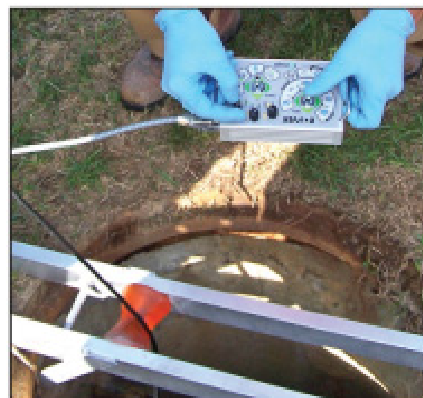
A remote control system helps direct the crawler-mounted side-wall scanning camera through the pipe.
