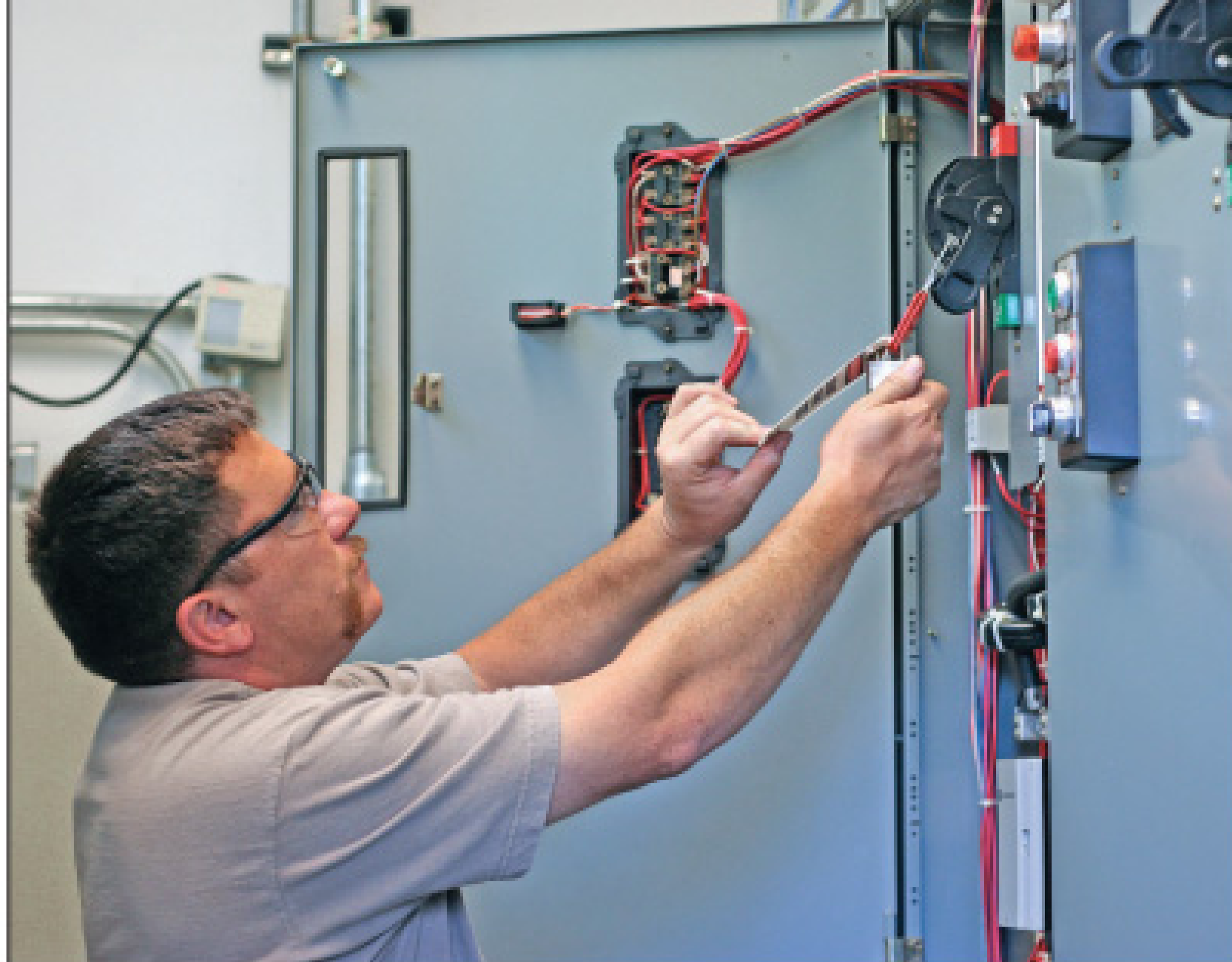
Gerald Arredondo, a 15-year veteran of the Pumps and Controls Group, sets up a power monitor for preventive maintenance. The goal of the group is to avoid breakdowns by maintaining, repairing or replacing equipment before it fails.
