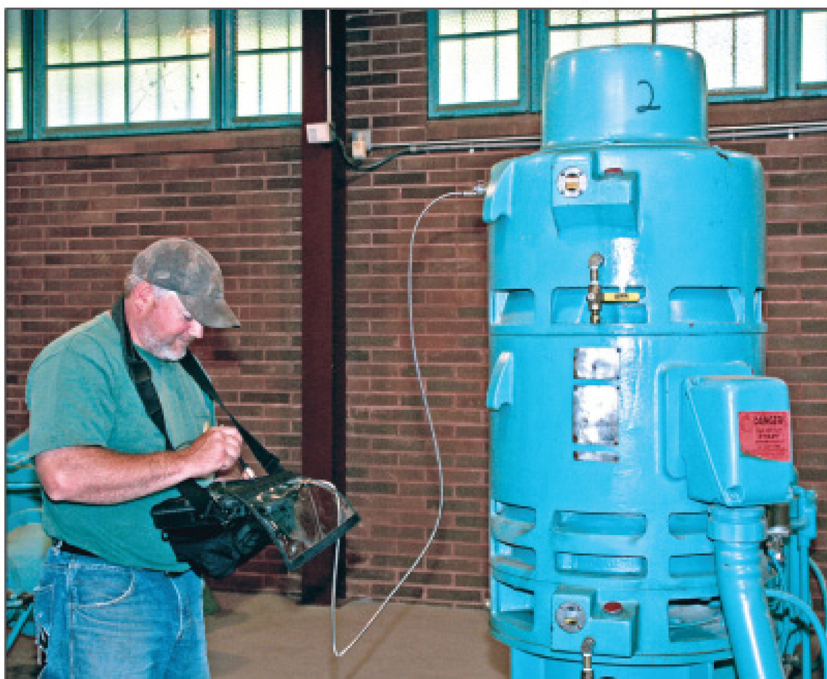
Shane Wallen uses vibration sensing technology for predictive maintenance on motors.
