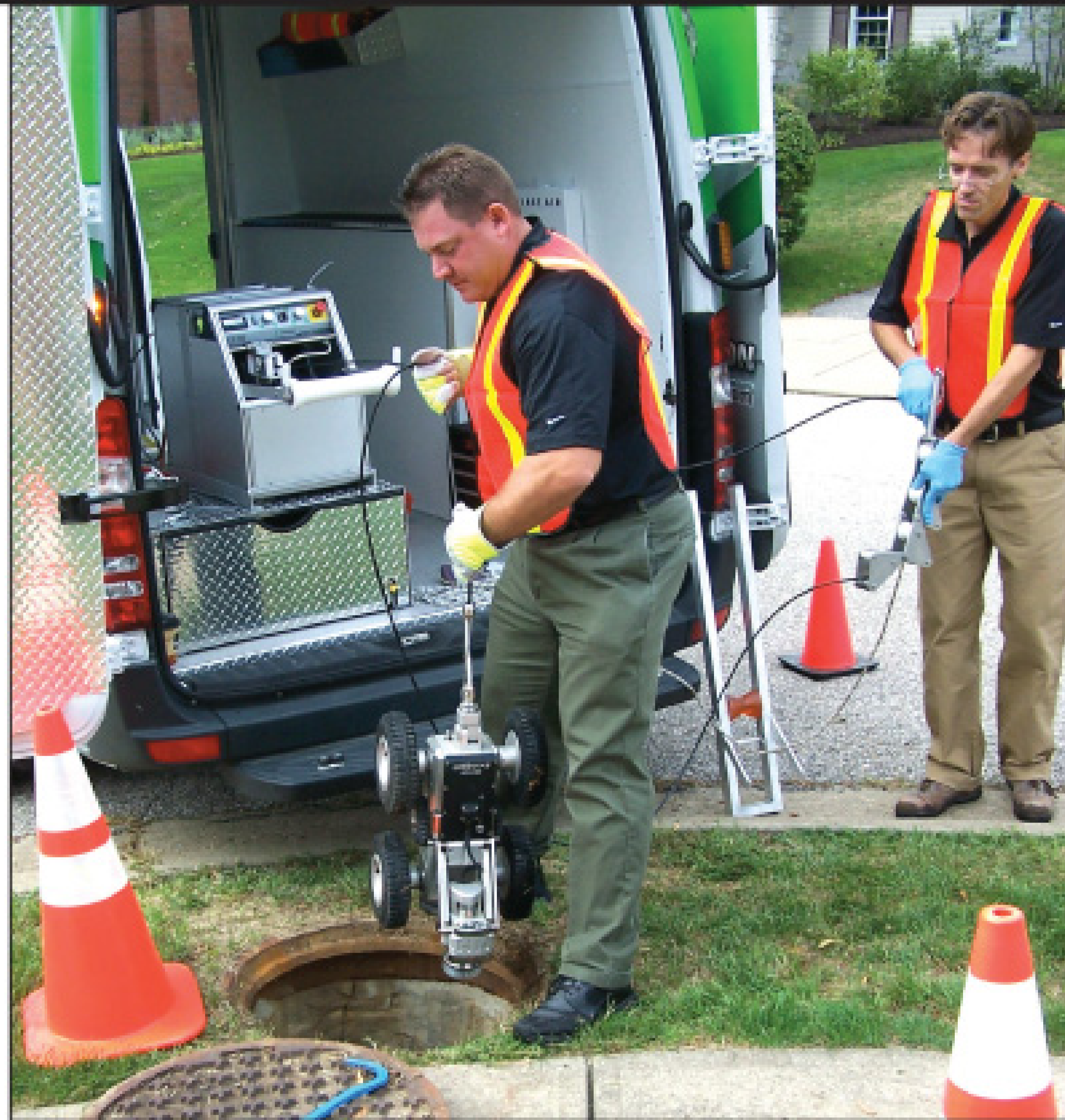
Jason Kelley, left, and Jake Wells of Envirosight prepare the DigiSewer 180° Inspection System.
