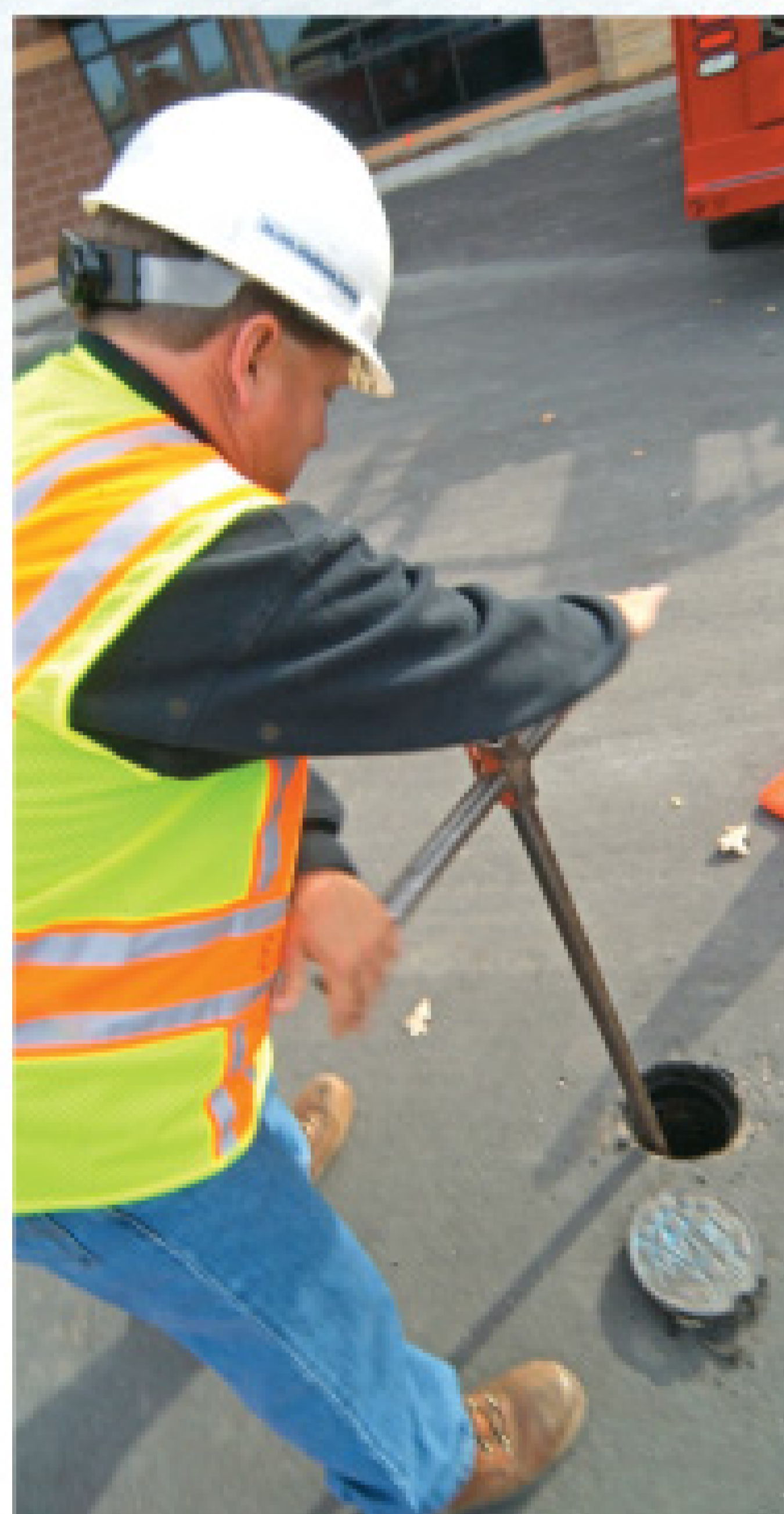
Dan Randolph exercises a water valve.
