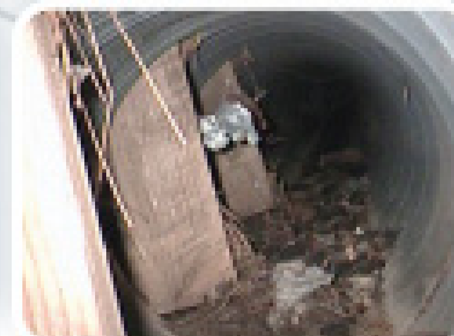
Fence Post Breach
