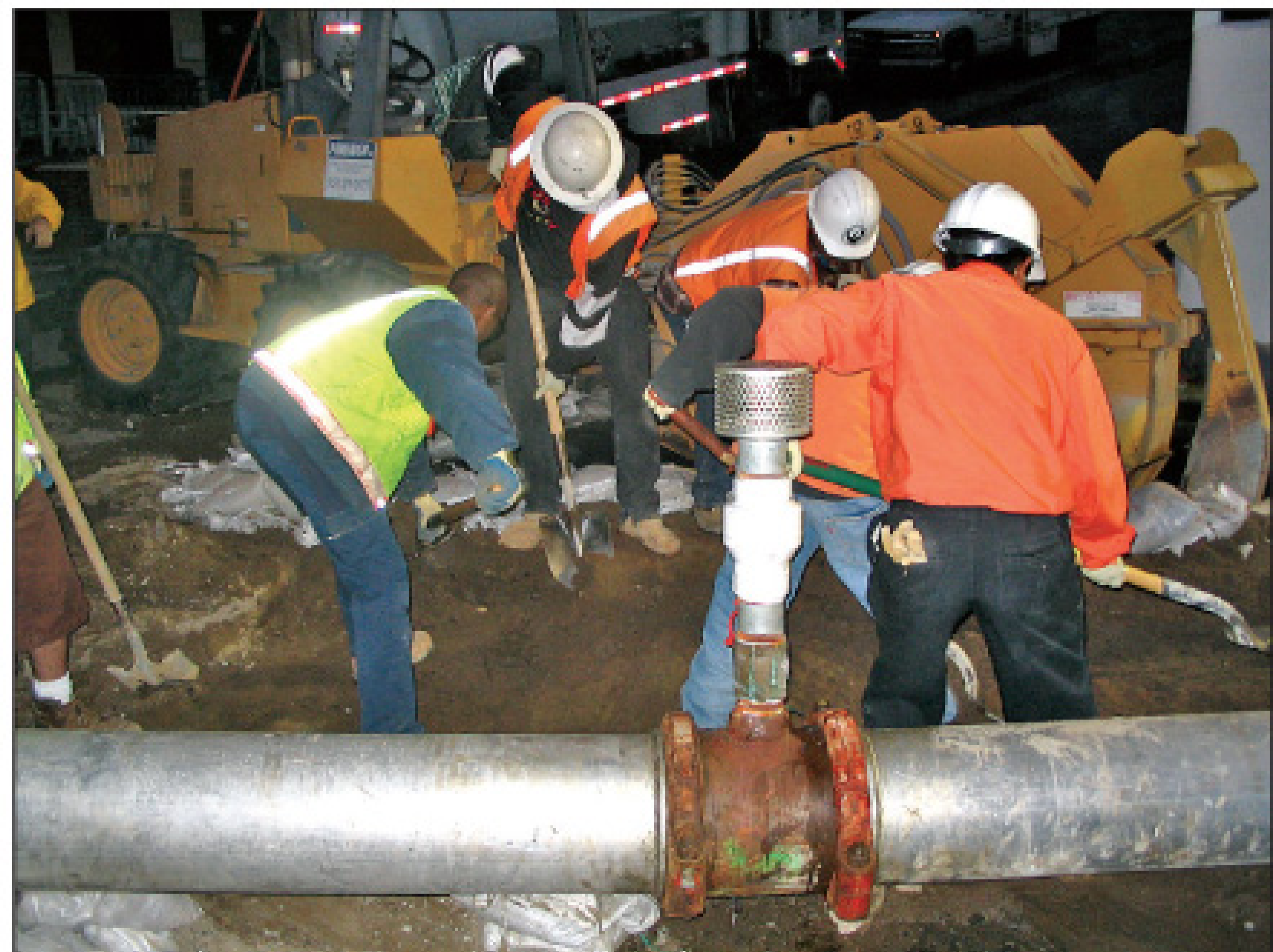
Districts crews construct a temporary above-ground 12-inch aluminum bypass piping system to limit a spill from a damaged force main. Crews also placed sandbags at nearby catch basins in case the overflow breached the containment area.
