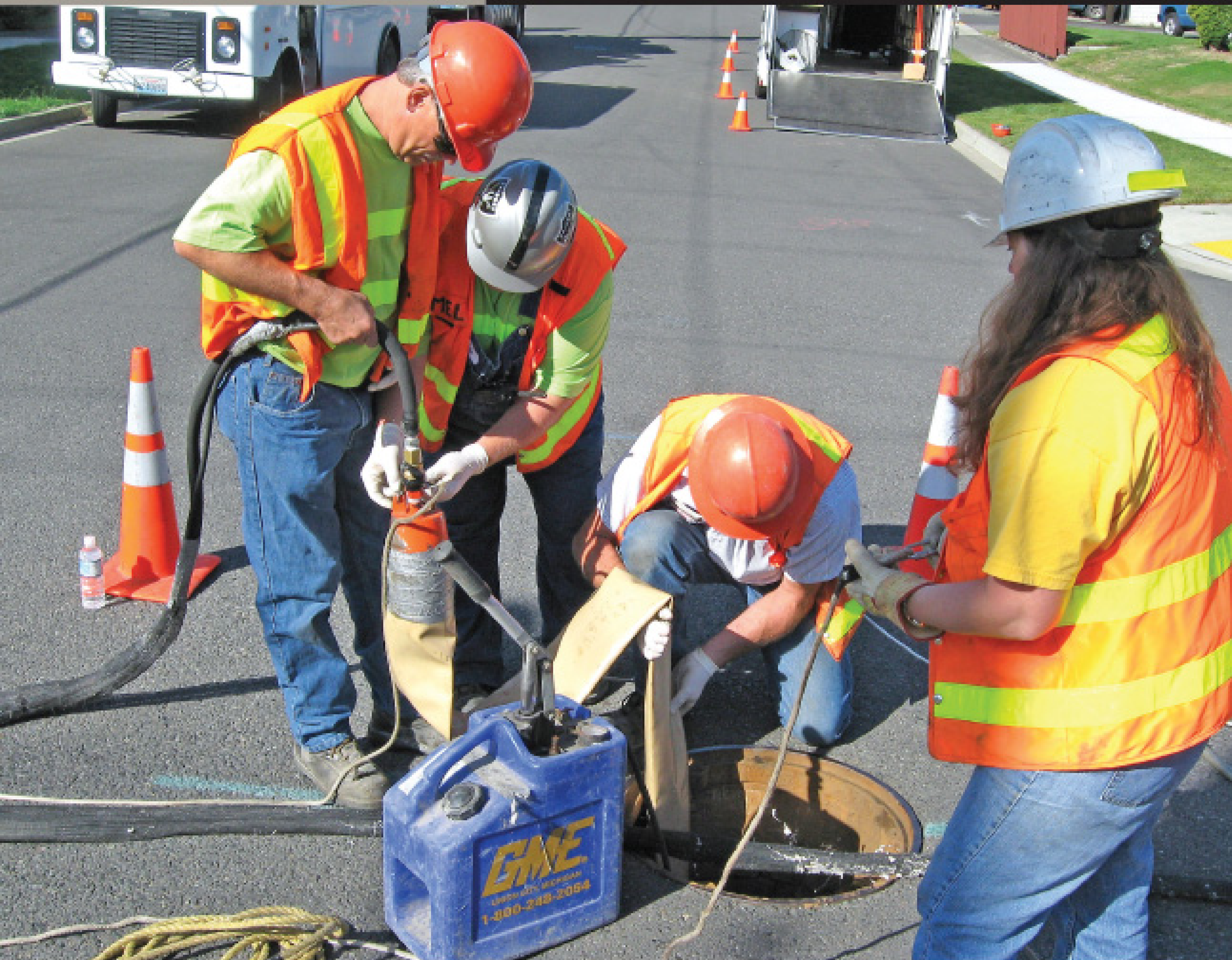
The ESMD crew installs the launching device for an LMK liner to seal a troublesome connection under an electric transmission tower. (Photos courtesy of the Environmental Services/Maintenance Division)
