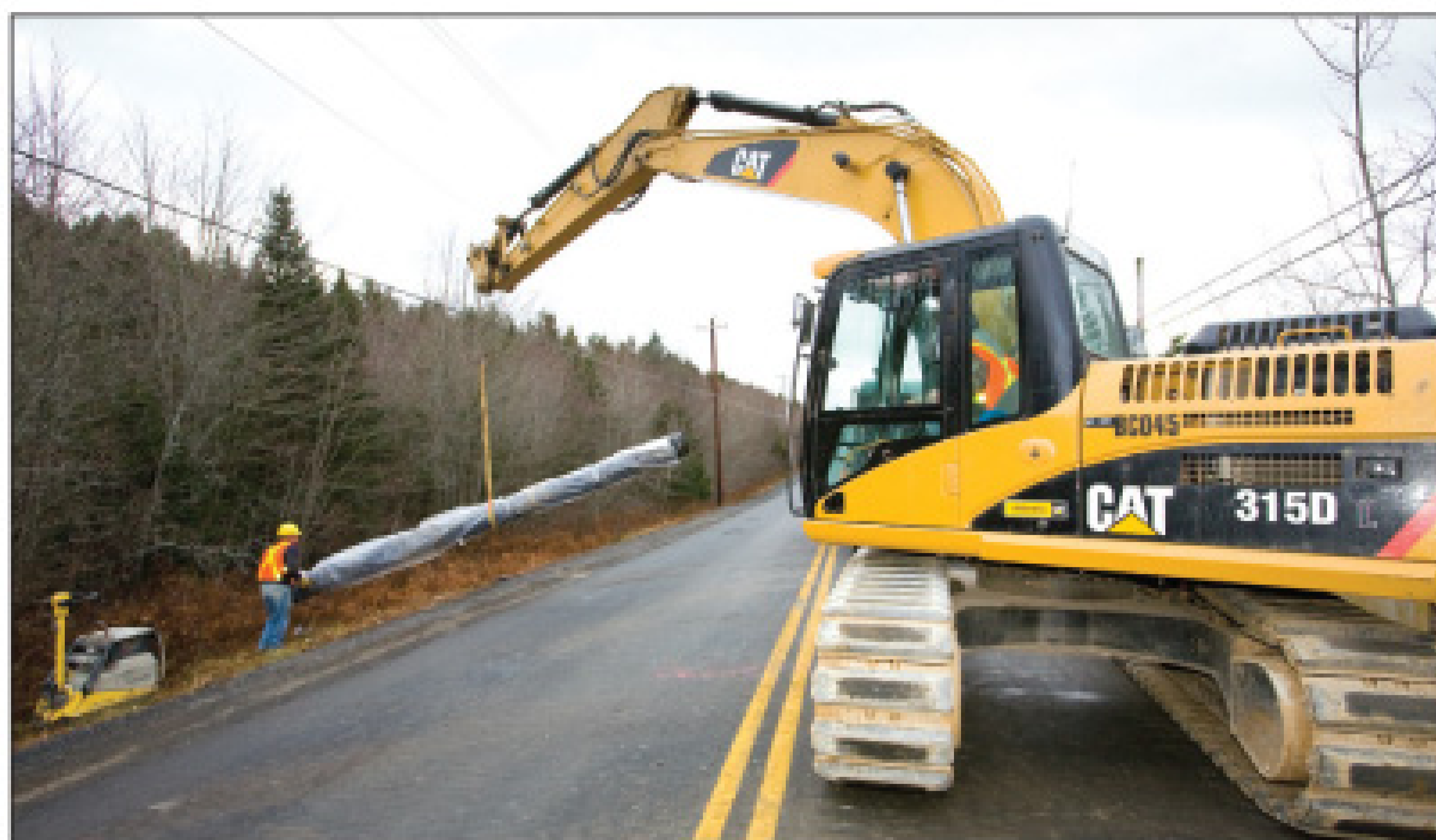
Halifax uses ductile iron pipe for most open-trench replacements. Here, crew member Paul Corbett guides a pipe section.
