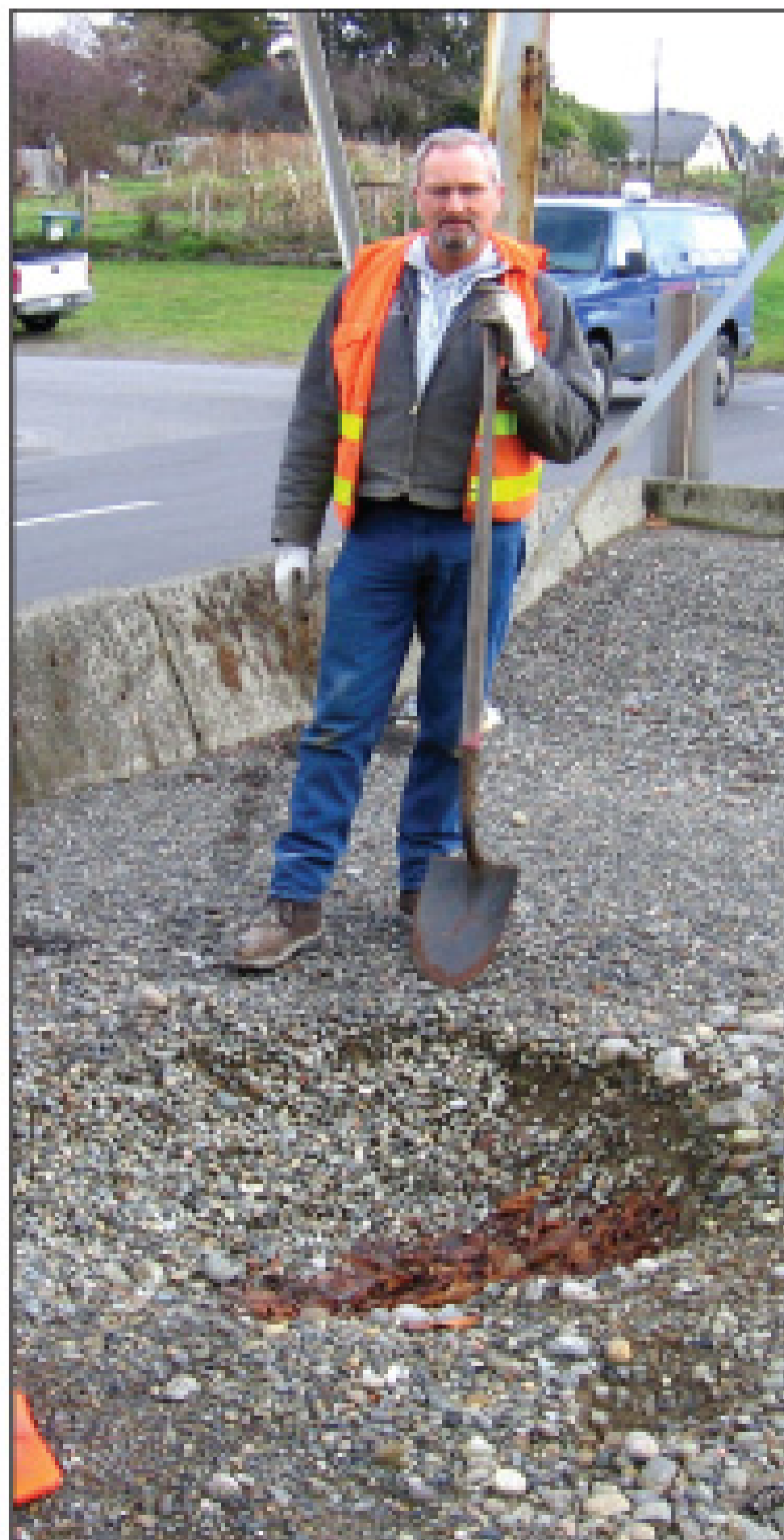
Mike Blake stands behind the sinkhole that formed under the 115-kV transmission tower because of the faulty sewer pipe.
