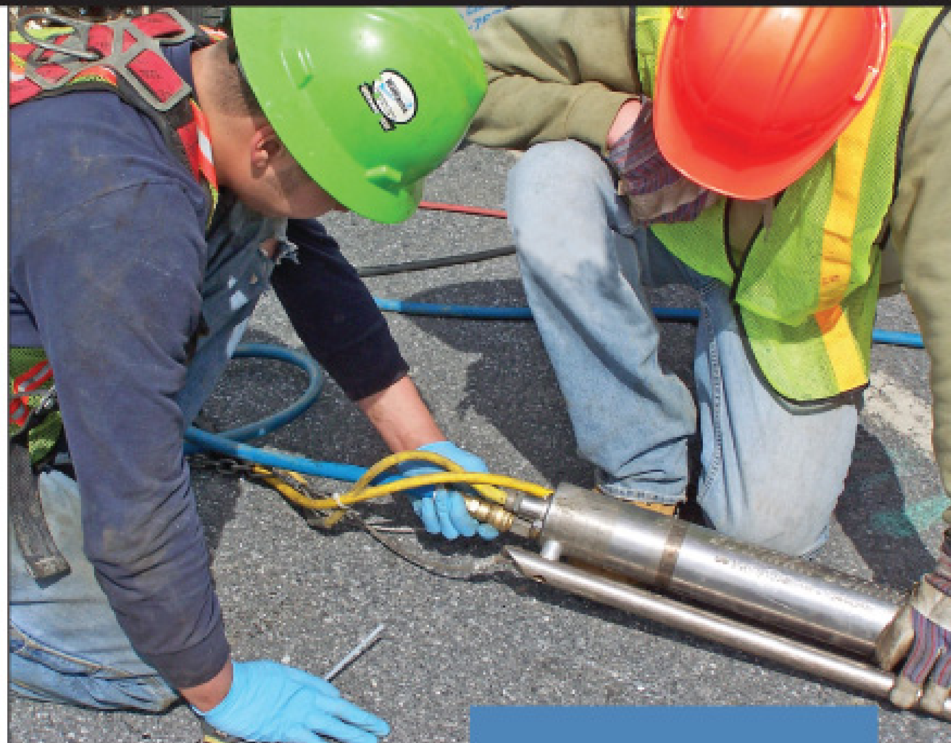
Wesley Logan (left) and Kyle McCarthy connect an air line (blue) and an electrical control cable (yellow) to the Dominator reinstatement cutter. (Photography by Gil Longwell)
