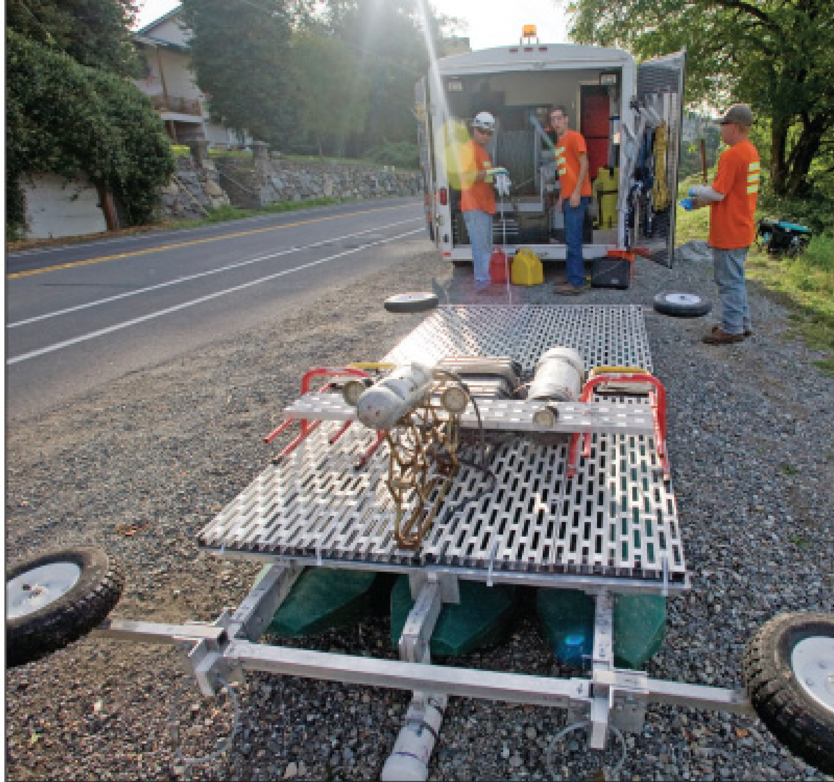
A crew from Pipe Experts Inc. of Tumwater, Wash., prepares a CCTV camera and sonar platform for the inspection of a 96-inch interceptor.
