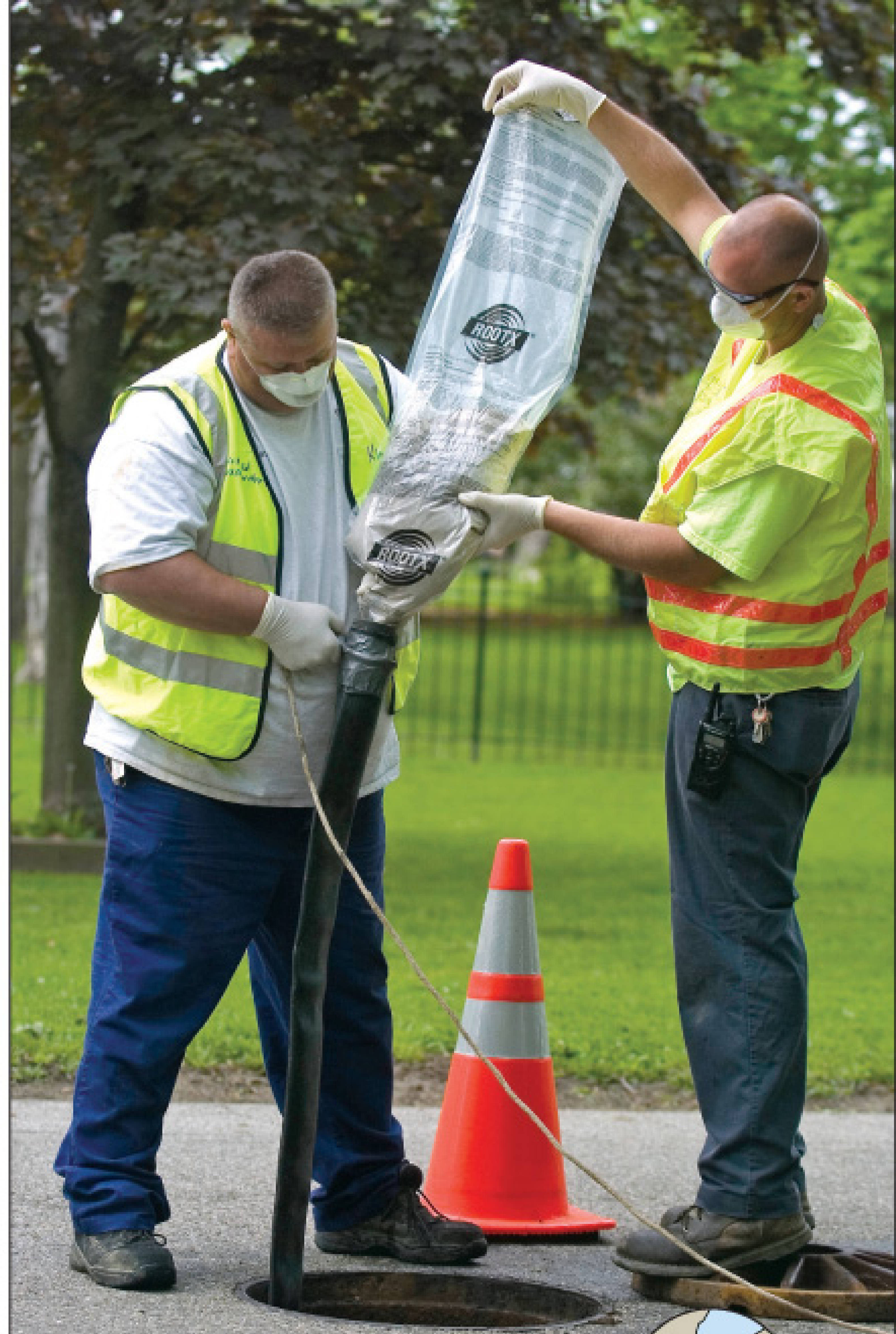
City of Fairfield maintenance operator Kim Campbell, left, and collection laborer Chris Croucher add RootX root treatment to a sewer line. The material, which foams on contact with water, is designed to kill roots in municipal and residential lines. (Photography by Carrie Cochran)
