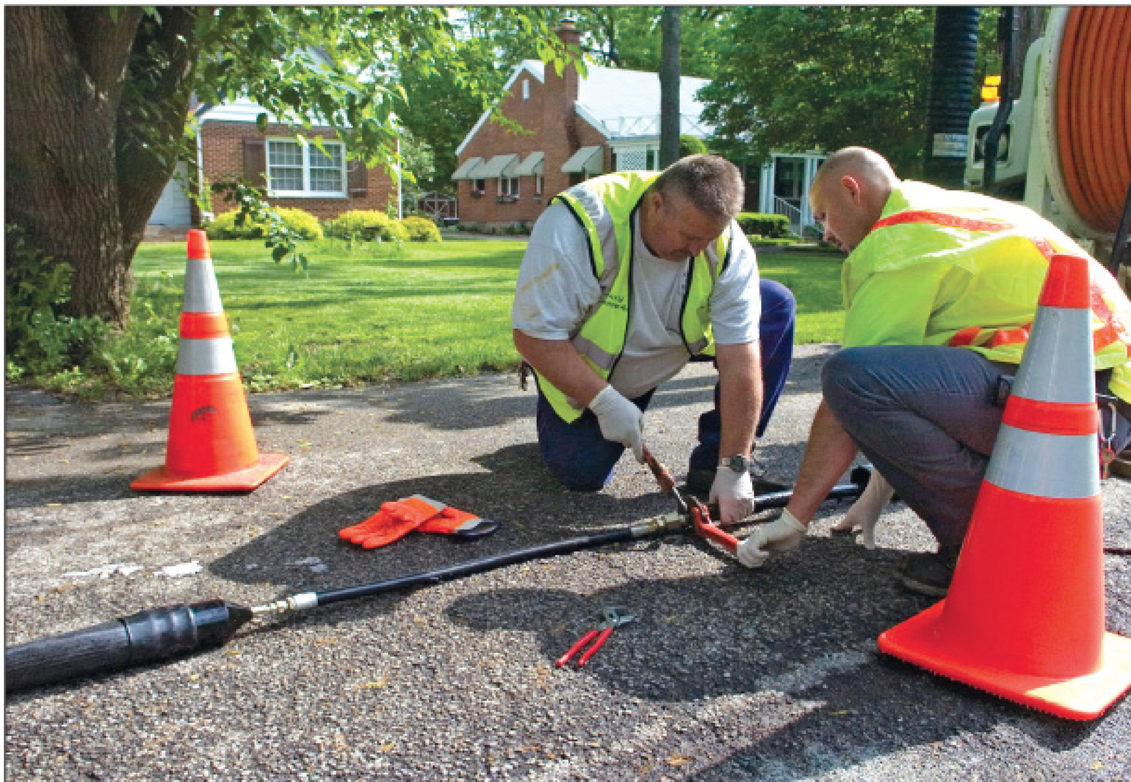
Maintenance operator Kim Campbell, left, and collection laborer Chris Croucher disassemble equipment after applying a root treatment.
