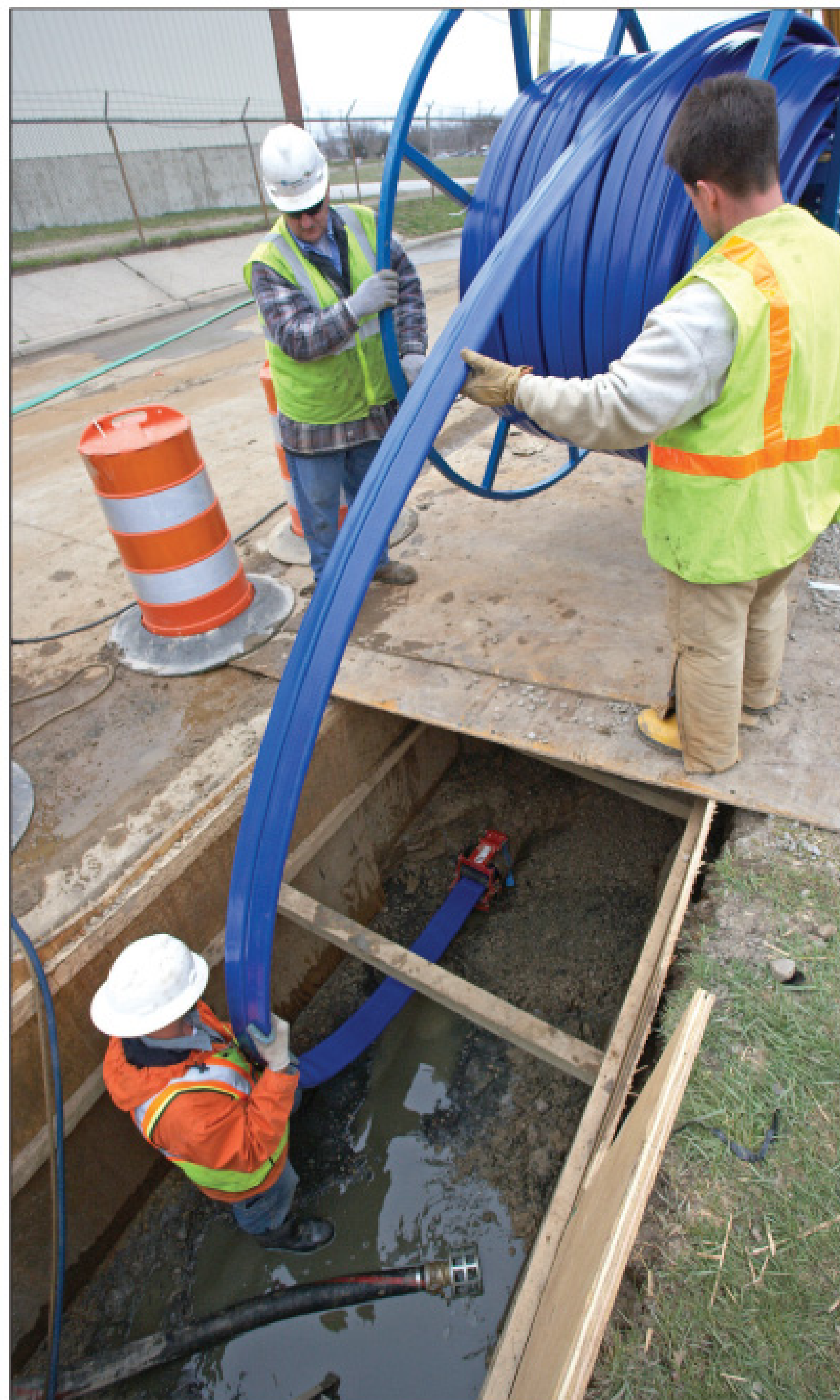
Thermopipe lining has helped the City of Monroe accelerate its water main rehabilitation program.
