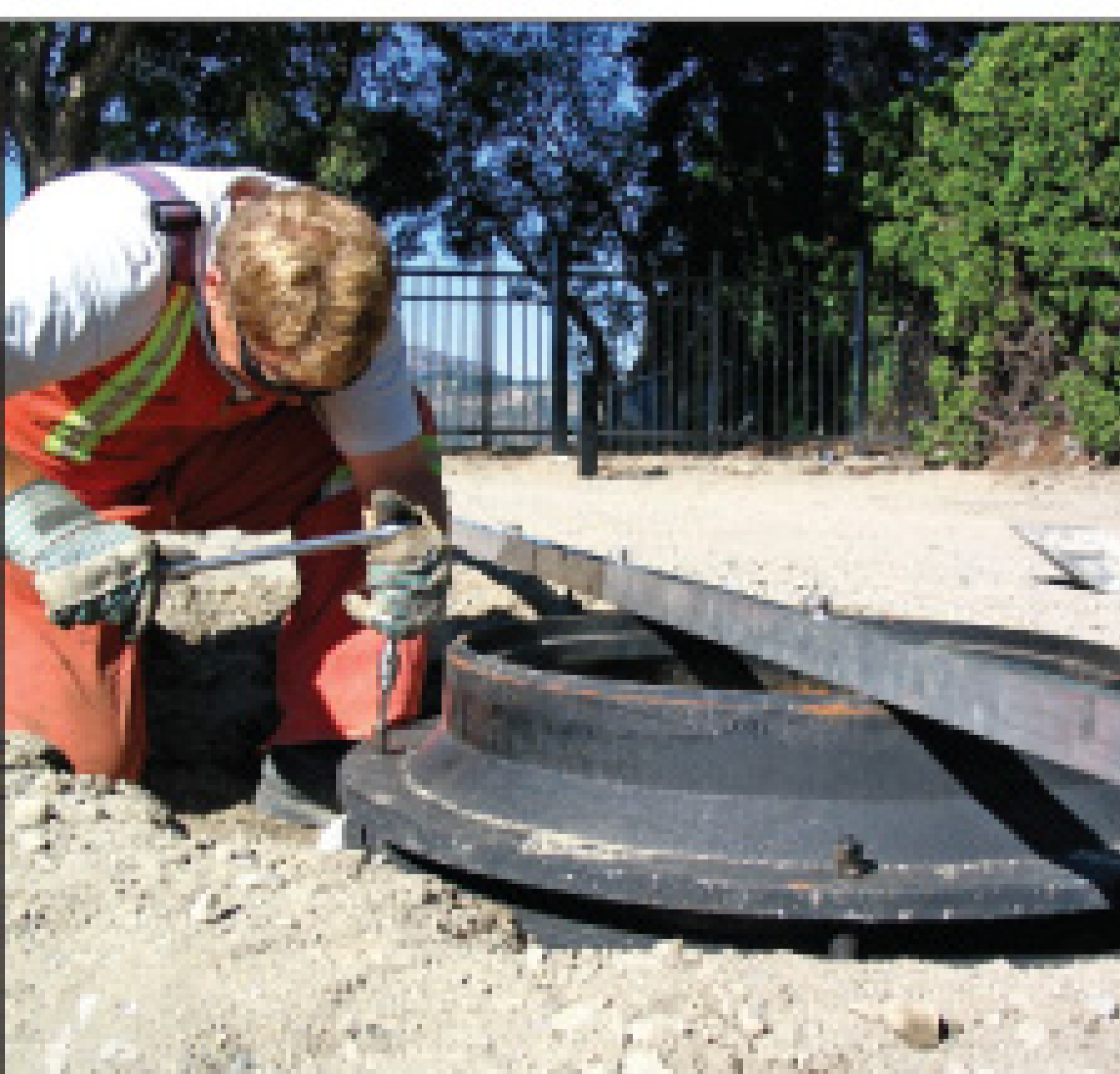
A worker sets an adjustable manhole frame using a bar to check the grade.
