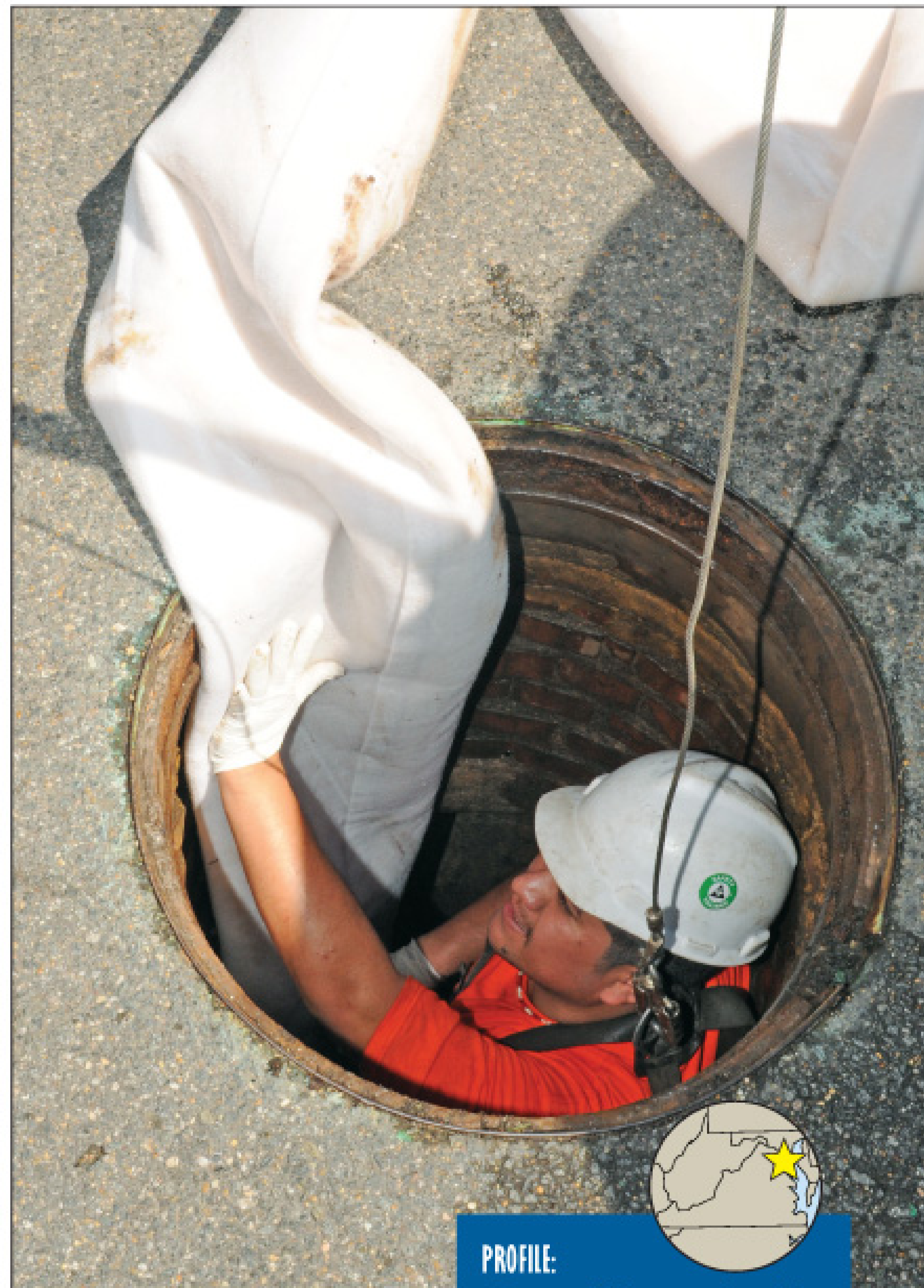
Carlos Satalan with AM-Liner East Inc., of Berryville, Va., enters a manhole to trim the excess liner. (Photography by Alan Lehman)
