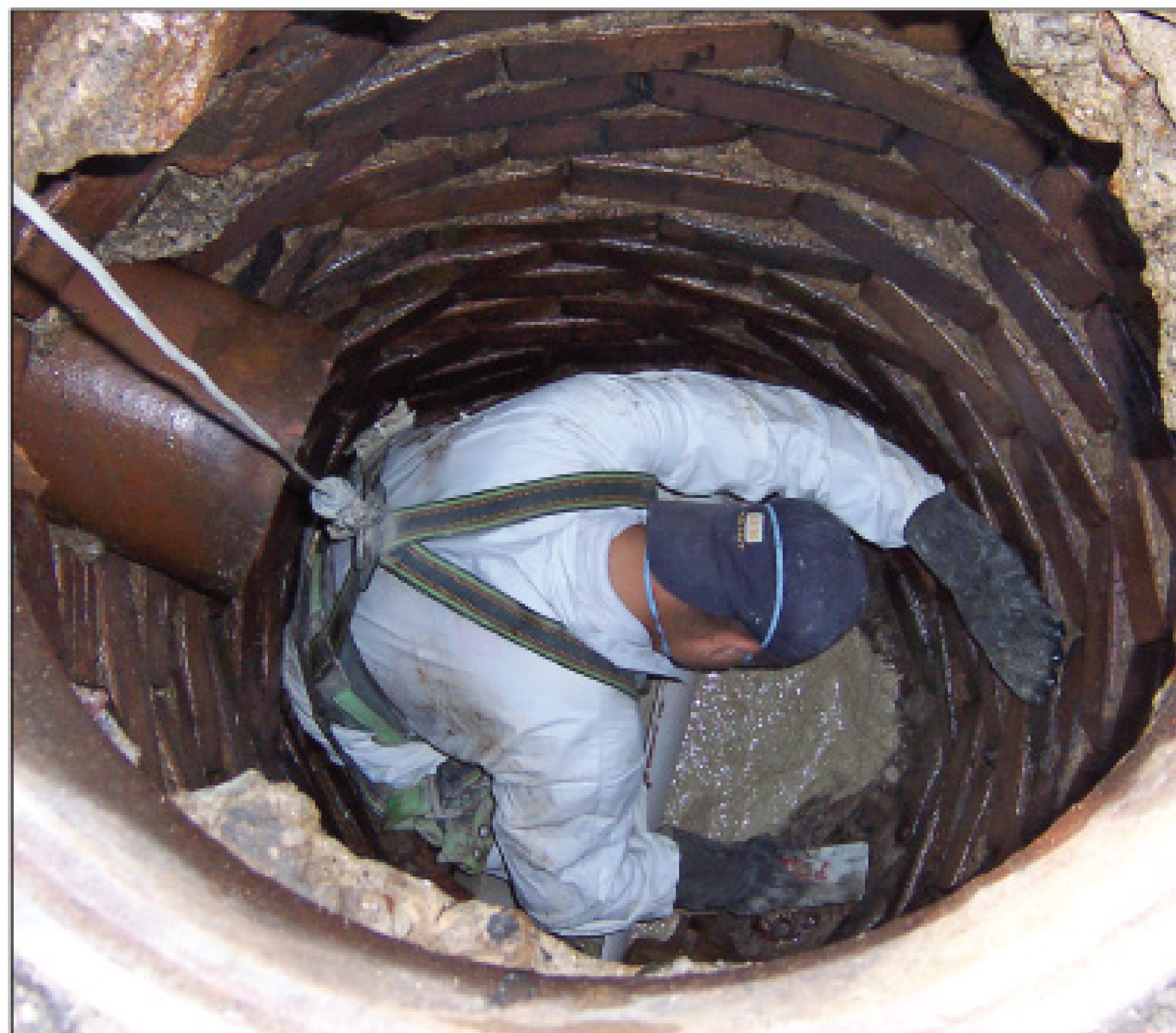
Corunna replaced four manholes, grouted 45, and lined two. Another 24 were rehabilitated through adjustments such as raising to grade, replacement, or sealing chimneys. Replaced and new manholes received custom lids cast by East Jordan Iron Works and bearing the city's name.
