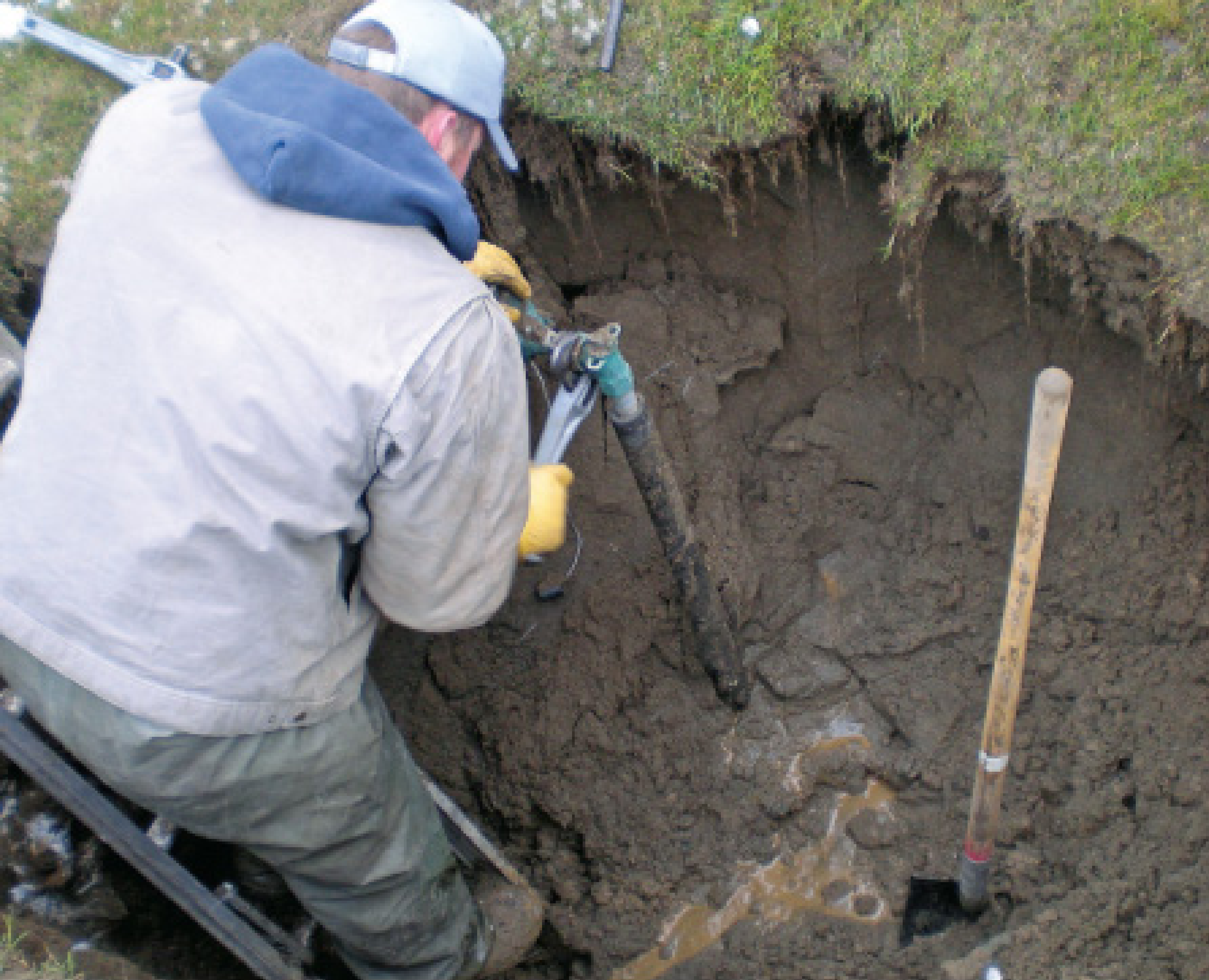
Rusty Widman replaces an outdated water meter with a high-tech Dialog 3G-DS PD wireless water meter from Master Meter.
