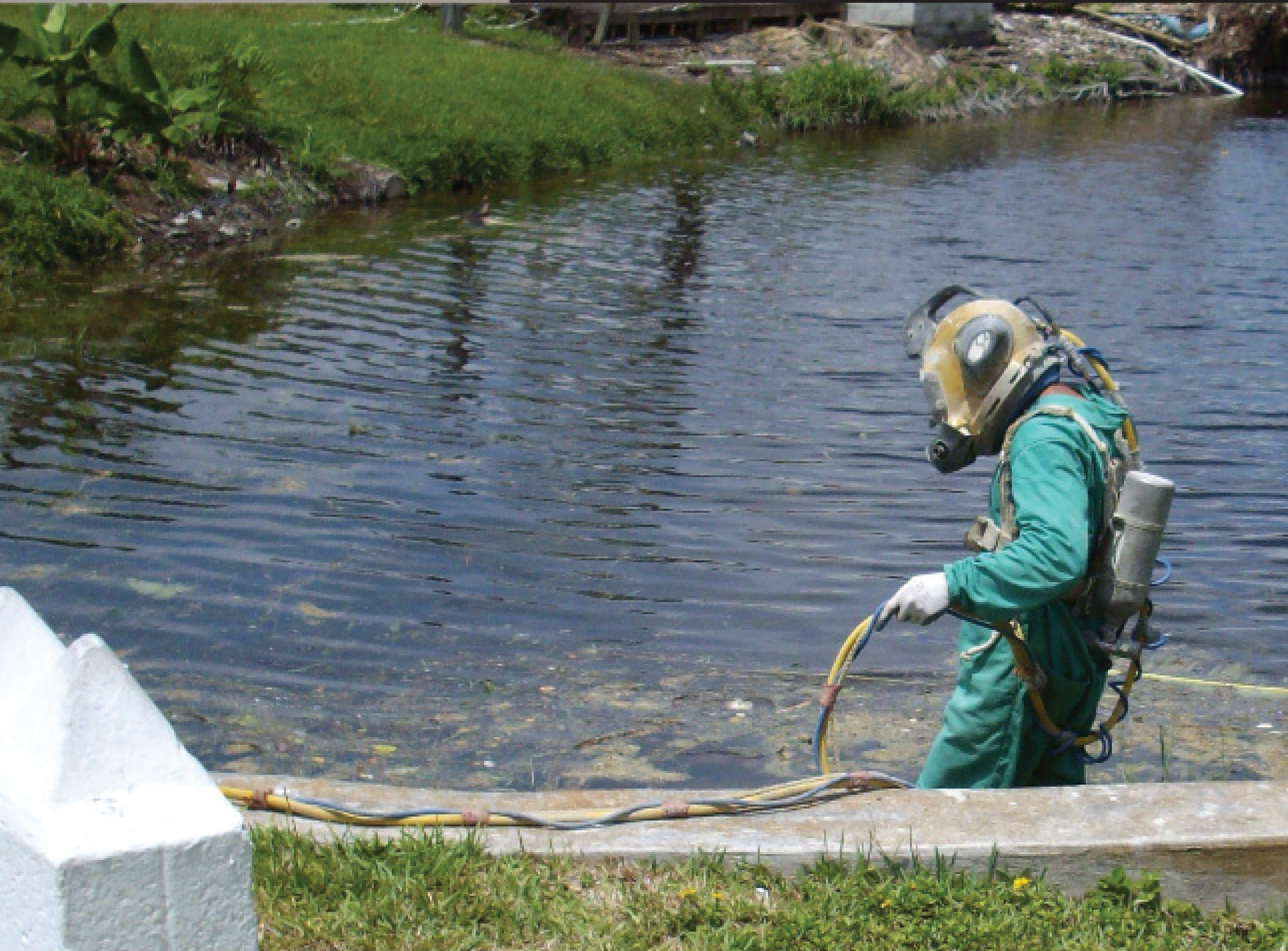
Professional diver Shaune Rogers approaches a blocked culvert with a HydroSurge nozzle. (Photography by Cooper Hong Inc.)
