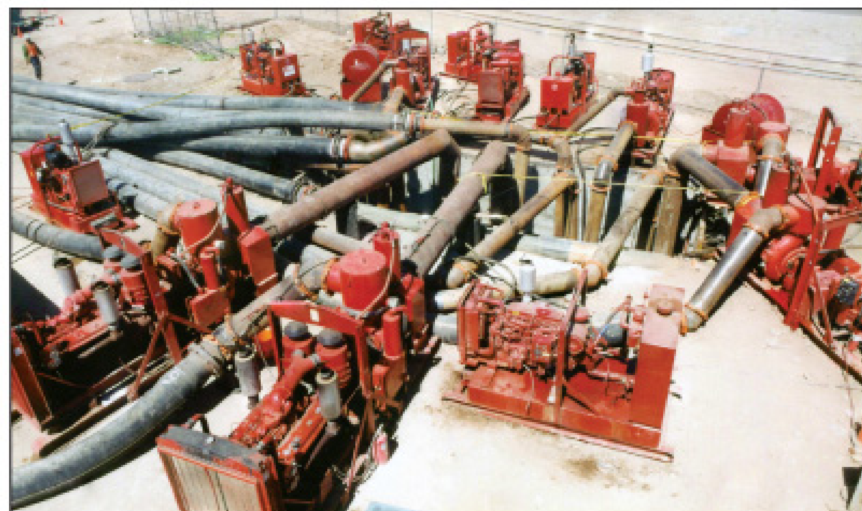
Hydraulic power units/submersible pumps and variable-use vacuum-assisted non-clog pumps are deployed on a bypass project in Phoenix, Ariz. The contractor was asked to provide pumps and backup for what was believed to be peak flow. However, the customer had miscalculated, and additional pumps were necessary. (Photos courtesy of Griffin Dewatering Corp.)
