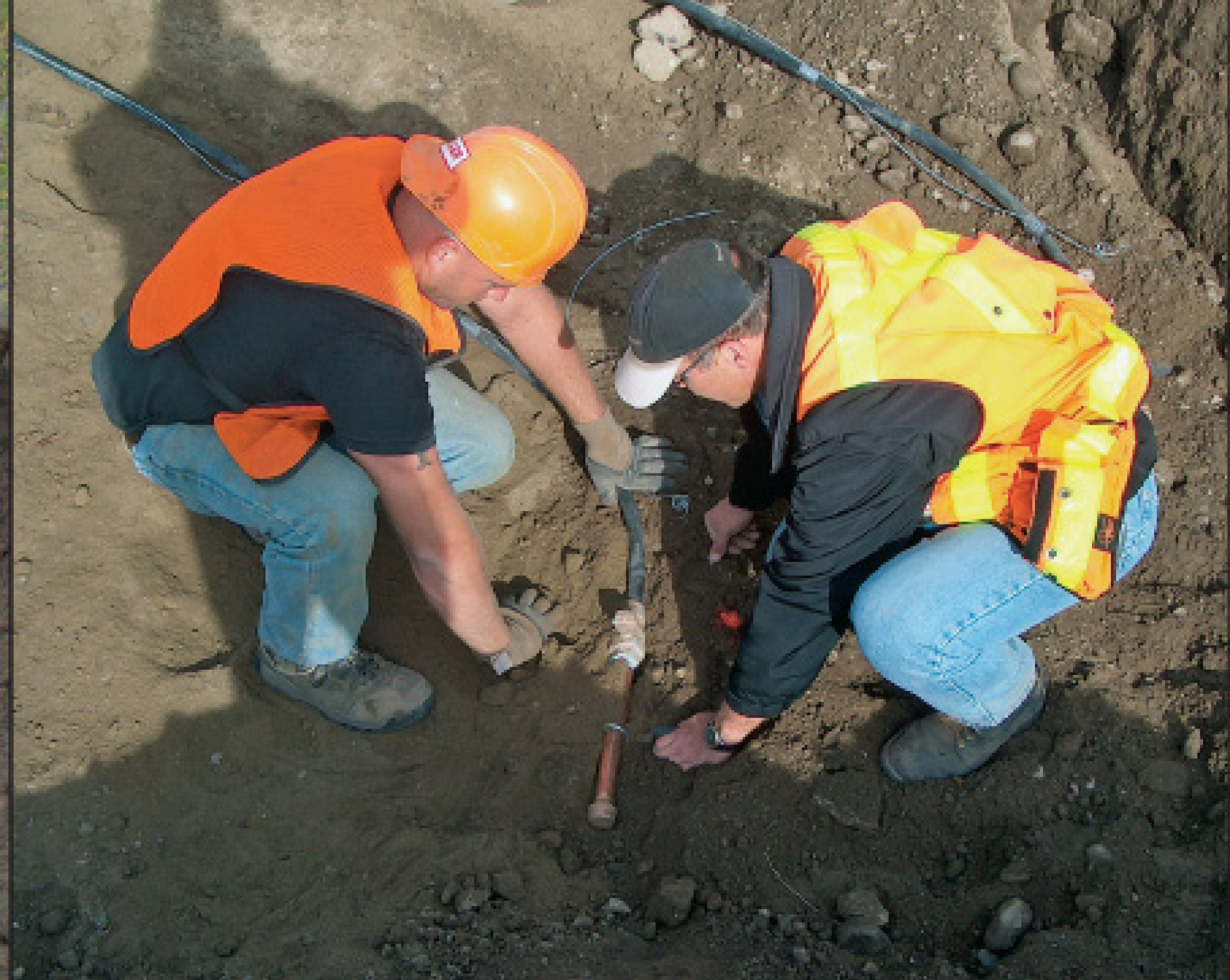
A worker from Eller Corp. finishes installing a service line for a new home using polyethylene pipe and tracer wire. The junction is a galvanized nipple with a brass cap that resists corrosion caused by acid soil. Mike Dschaak (right), an inspector from Simpson Engineering Inc. checks the completed work.
