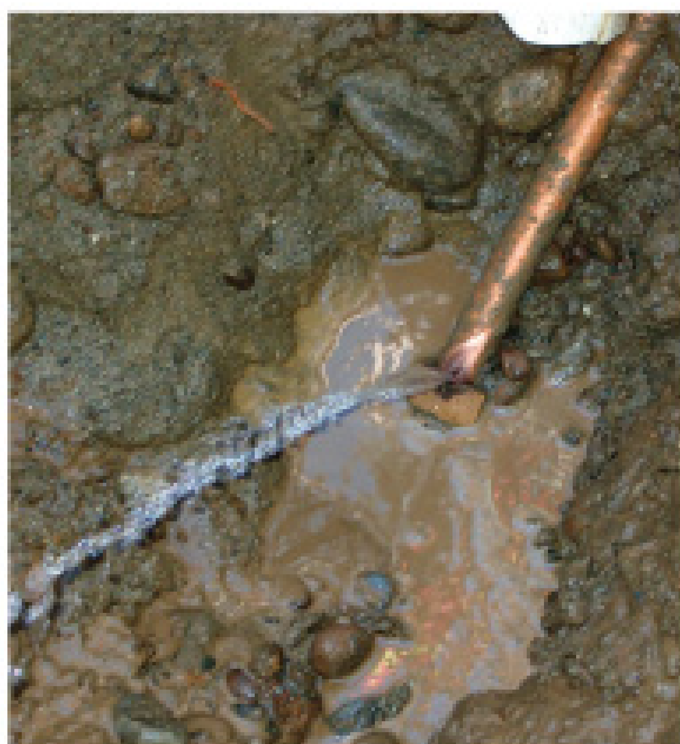
Cast iron lead-joint pipe proved to be the biggest culprit in Pasadena Park's leakage problem. The cast iron was intact, but the lead joints had deteriorated.
