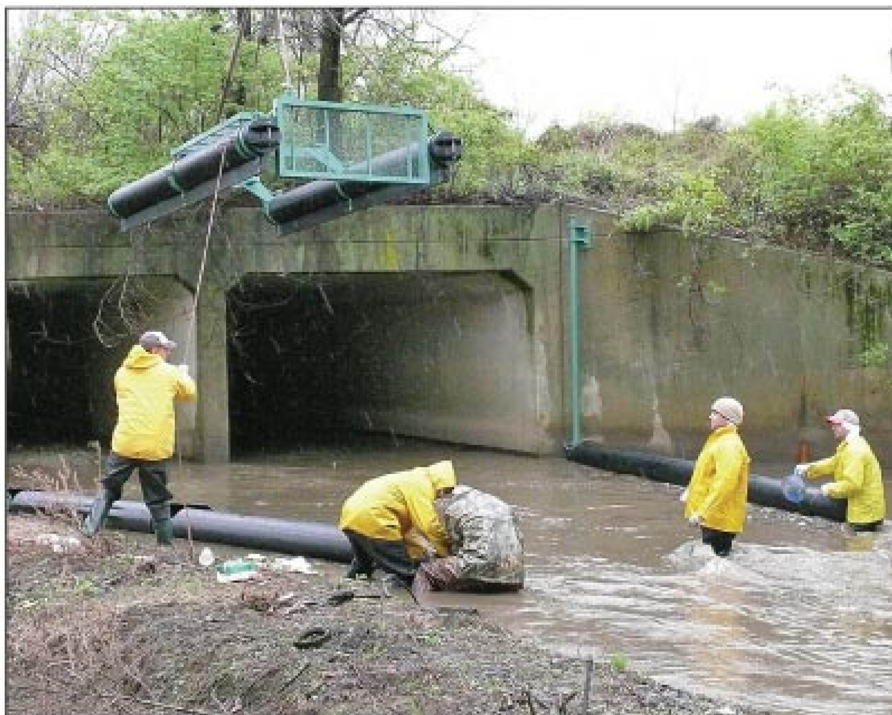
A worker guides the 600-pound partially preassembled aluminum and HDPE trap as the hydraulic lift lowers it over the side of the bridge. Note the first set of flotation booms attached to the rider poles on the wing walls of the bridge.
