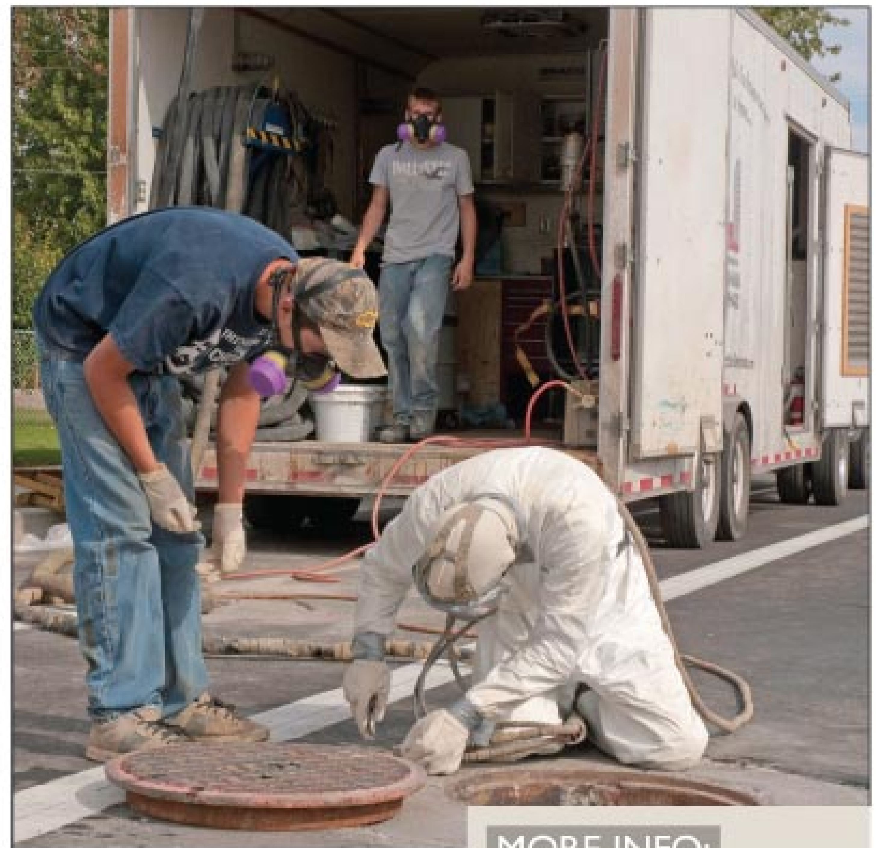
Juan Pena performs maintenance on a lift station grinder pump.
