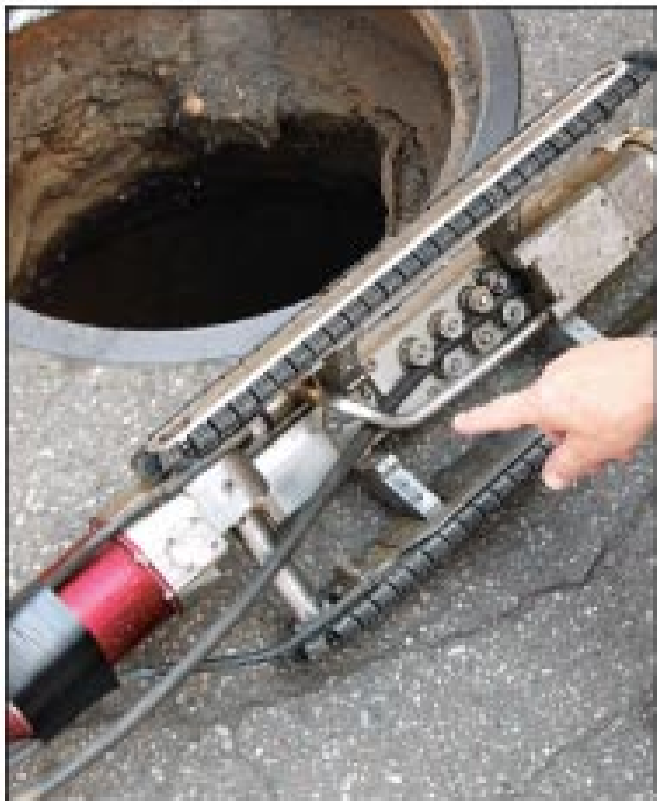
Richard Schantz of Aries Industries points to the powered rollers on the crawler that drive the push cable for the lateral camera.
