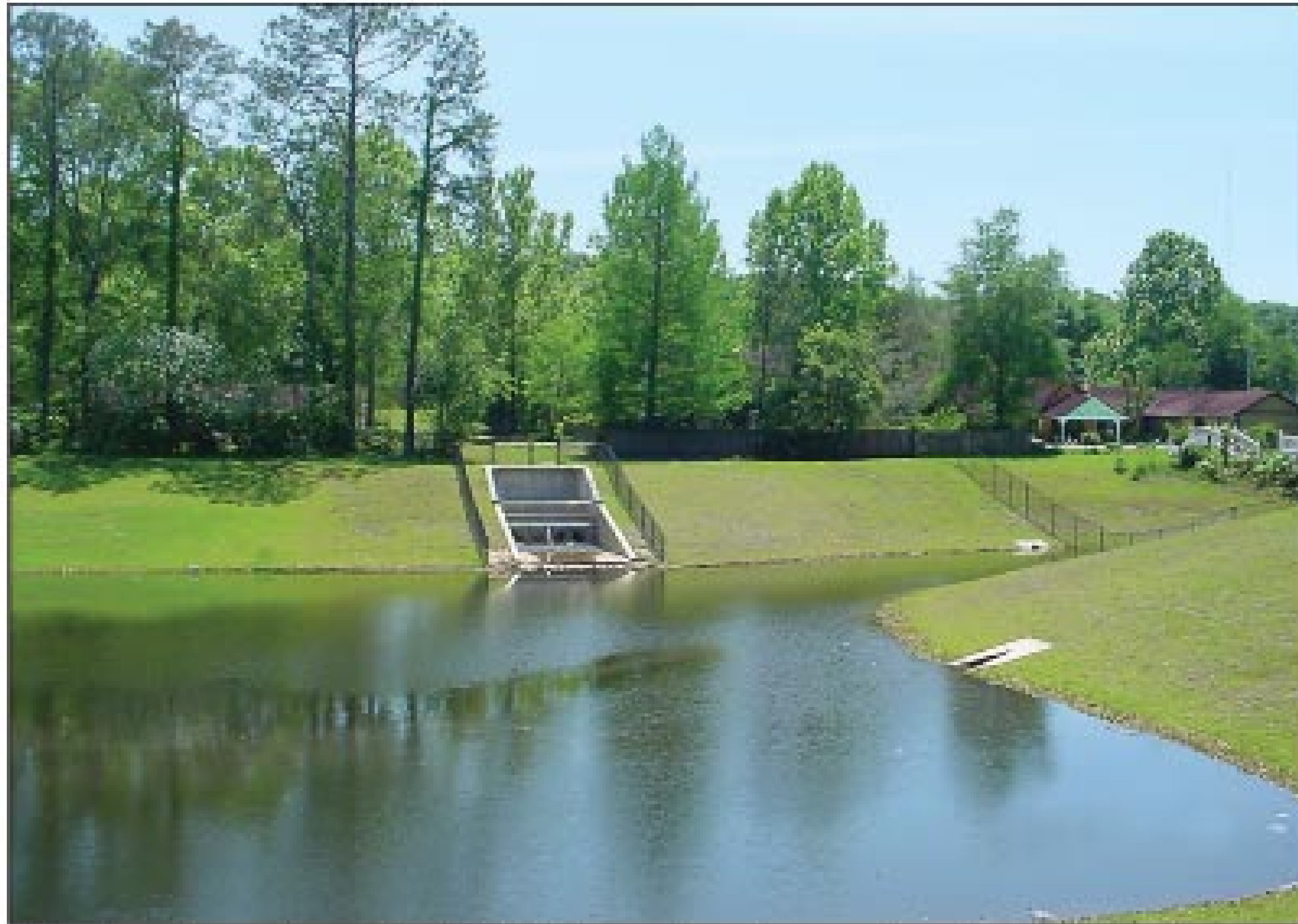
The structure at center left is the major stormwater input to Abbiegail Pond, a wet detention facility in the headwaters of Lake Jackson. The structure includes substantial hardware for trash and debris collection to help maintain the pond's appearance. (Photo courtesy of John Cox)
