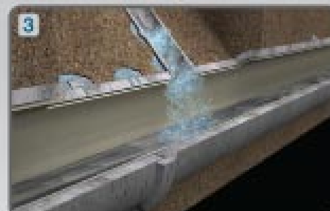
Continues to leak in annular space
