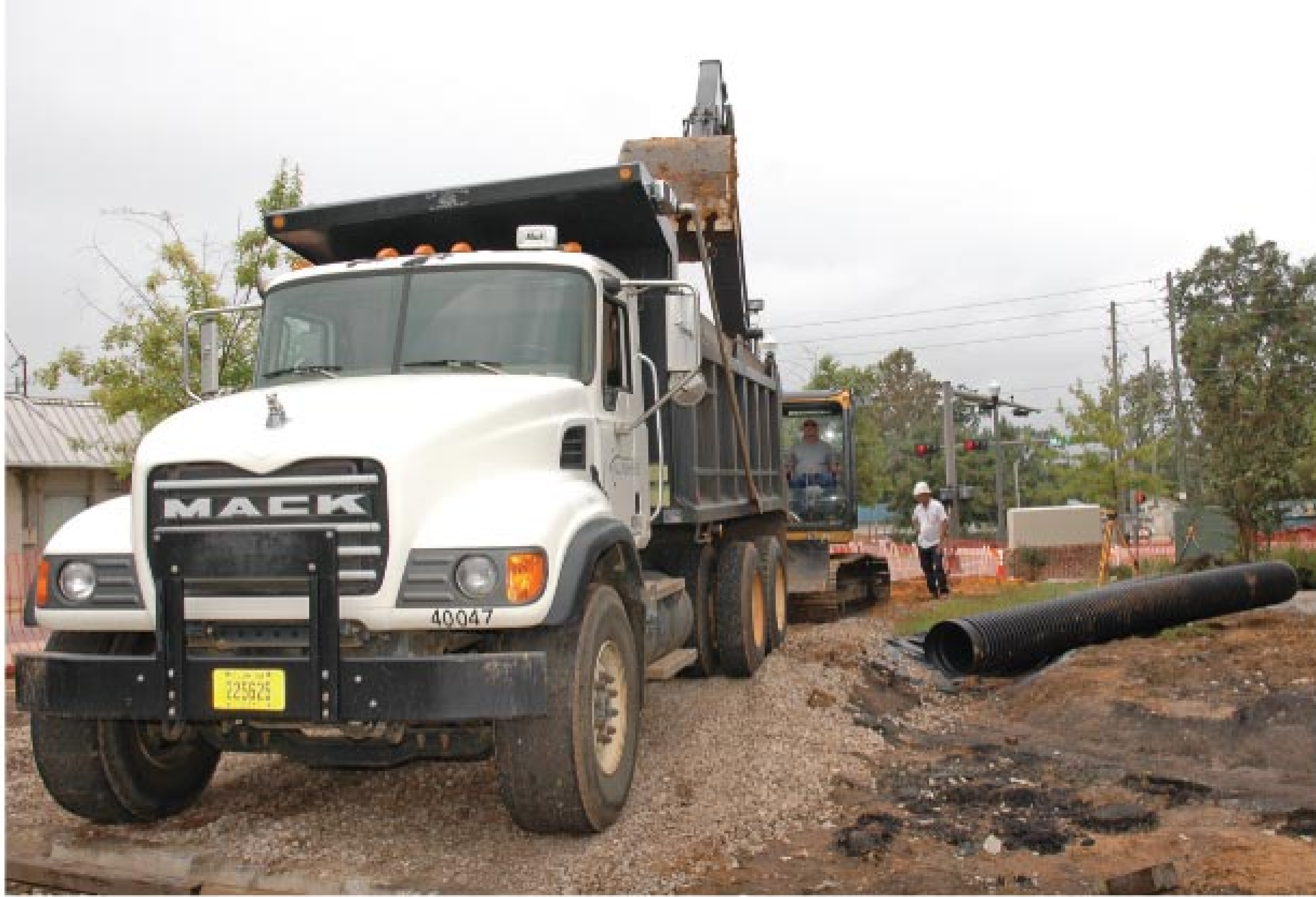
Workers install an advanced drainage system at the City Hall Renaissance Building.
