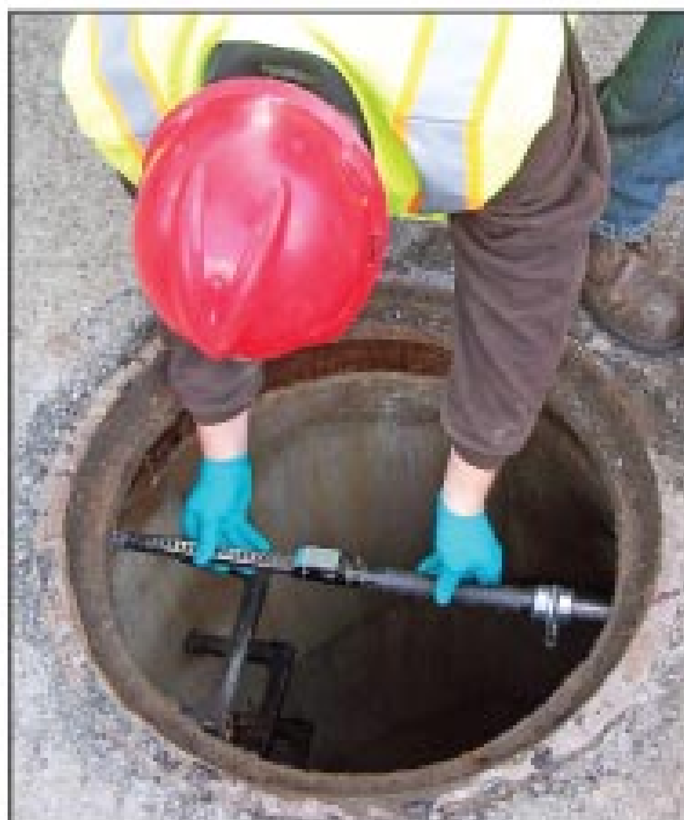
A technician tightens the hanger bar inside the entry manhole. The robotic crawler is tethered to this bar.
