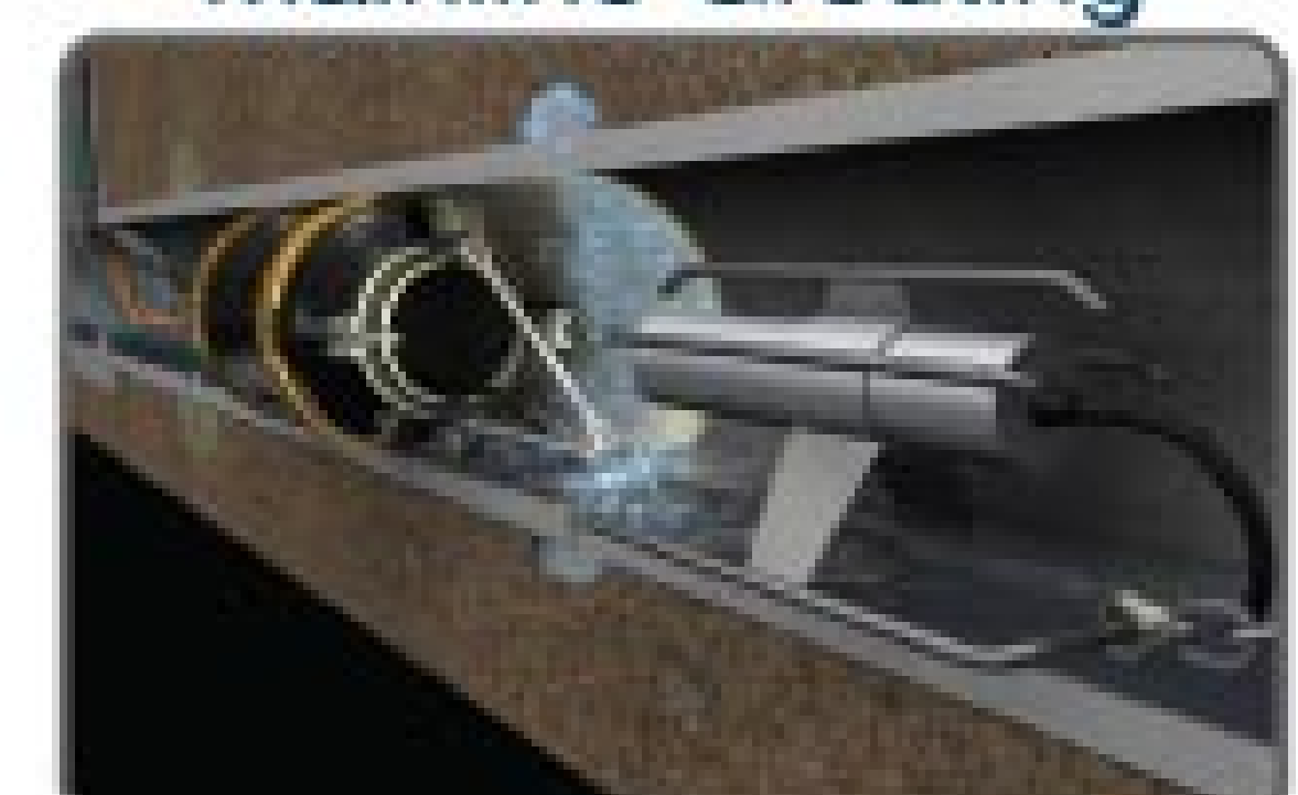
Leaking joint in mainline sewer
