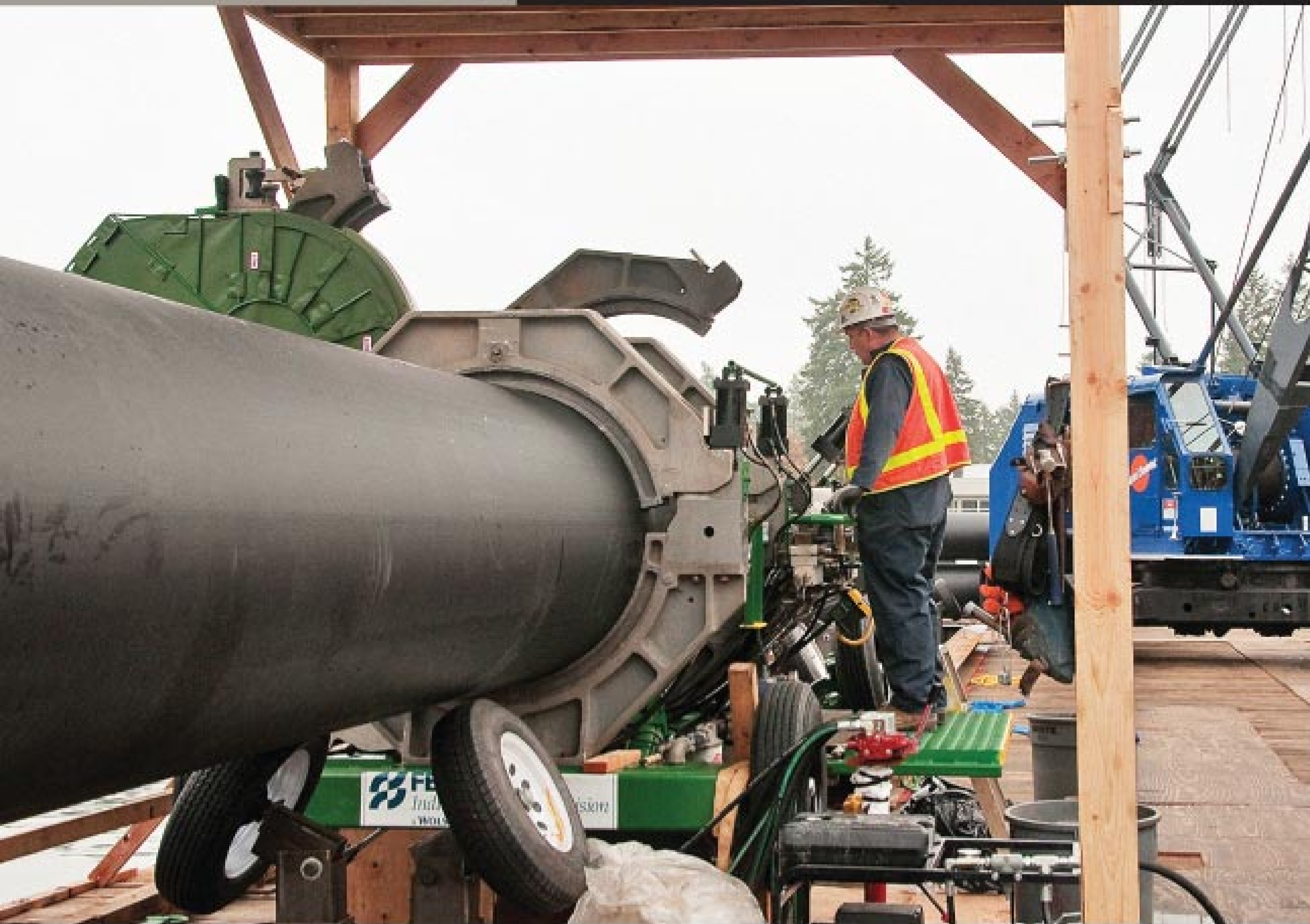
Pipe fusion technician David Marcum from Ferguson Industrial Plastics hydraulically raises the jaws of a McElroy 1648 fusion machine used to fuse the pipe for the Lake Oswego sewer interceptor project. The jaws held and rerounded the pipe during the fusion process. (Photos courtesy of Tyler Henning, McElroy Manufacturing Inc.)
