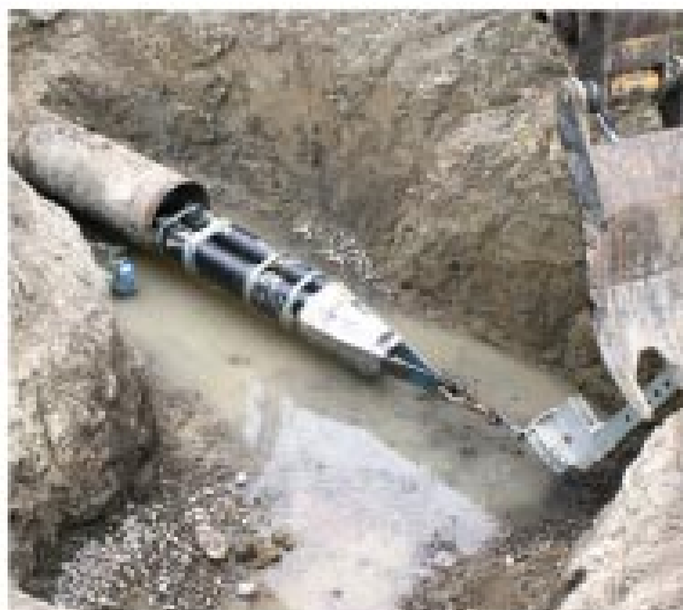
The pulling head for the modified slip-lining process is shown entering the receiving pit.
