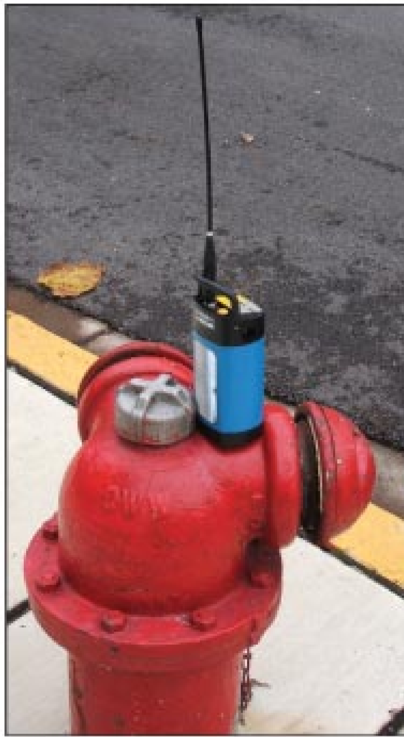
One of two Eureka Digital listening units, this one attached to a fire hydrant near the suspected leak location. A second unit was attached to another hydrant about 300 feet away.
