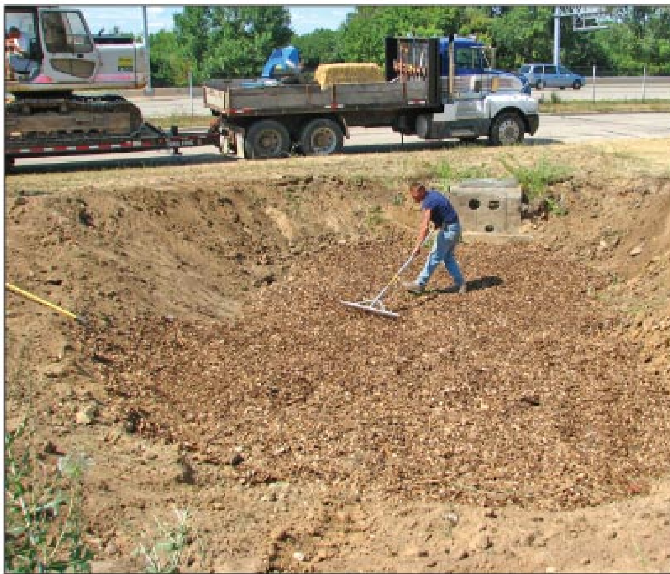
This bioretention system, shown under construction at an early stage, was built on a retail property in the City of Madison.
