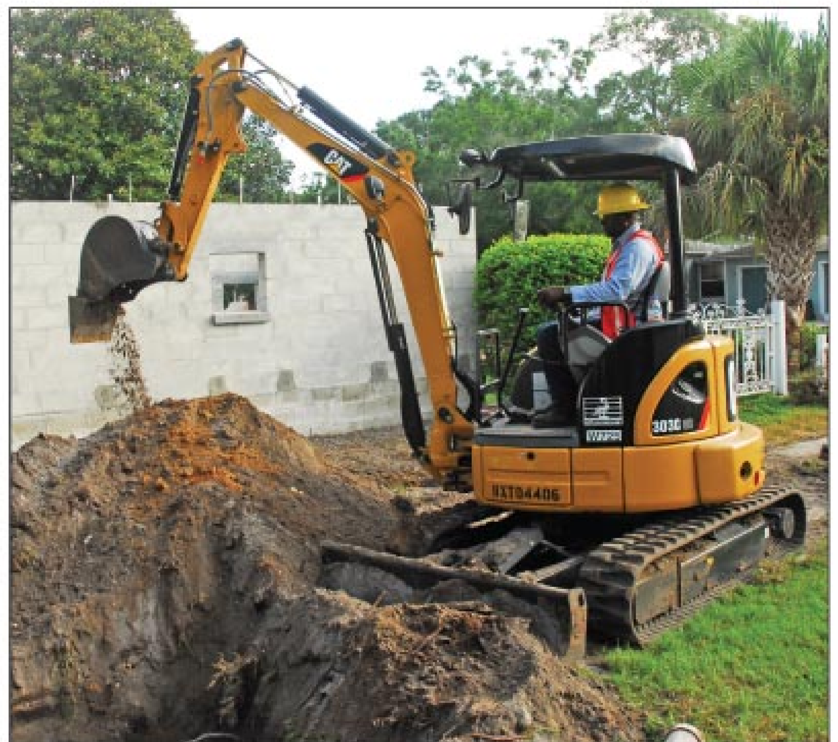
The Corrective Maintenance Repair crew uses a mini-track hoe to excavate a problem line and install a new section of PVC pipe.
