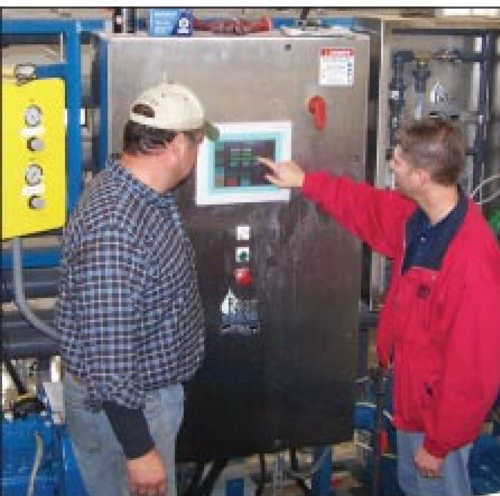
City of Beaver Dam utility foreman Rob Minnema and operator Greg Goodrich review the touchscreen controls on the skid-mounted belt filter press from Bright Technologies. The press serves both the water and wastewater sides of utility operations.
