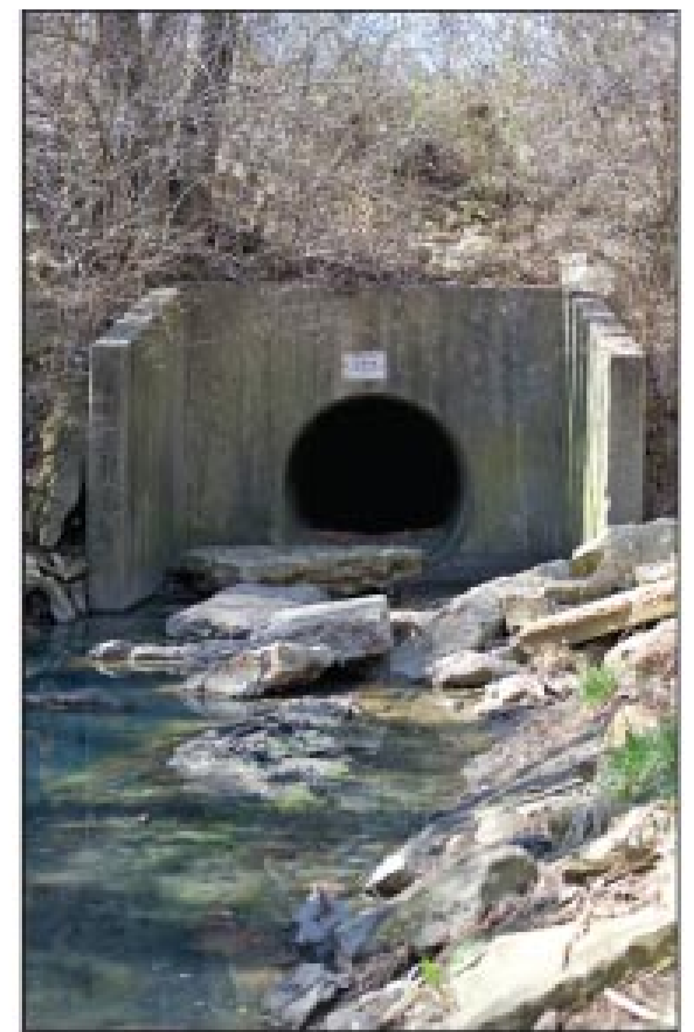
A combined water outfall in Kansas City includes a brick weir that retains sewage. During heavy rains when capacity is reached, runoff topples over the wall and spills into the Brush Creek watershed.
