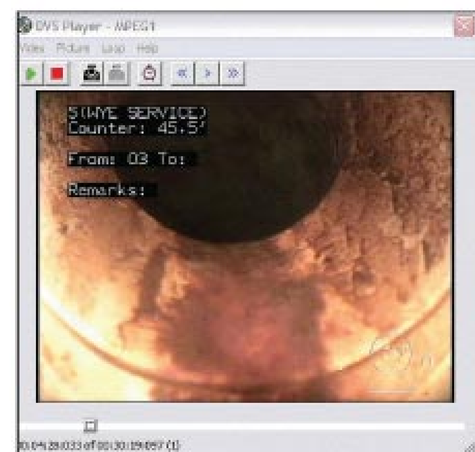
Video and pictures are exported from flexidata survey software to Cityworks, where they can be displayed from the inspection form.
