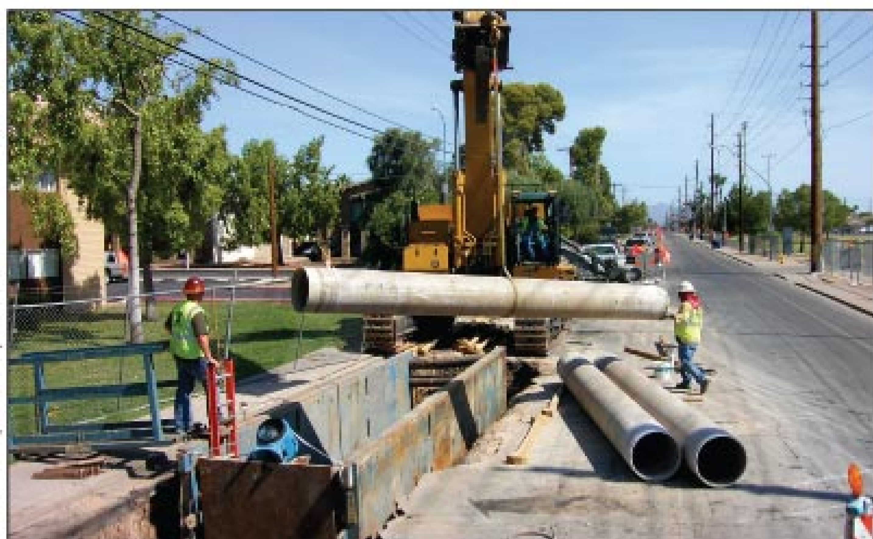
Decisions on which pipes to rehabilitate first, by methods including slip lining, are made with the support of the SCRAPS software application.
