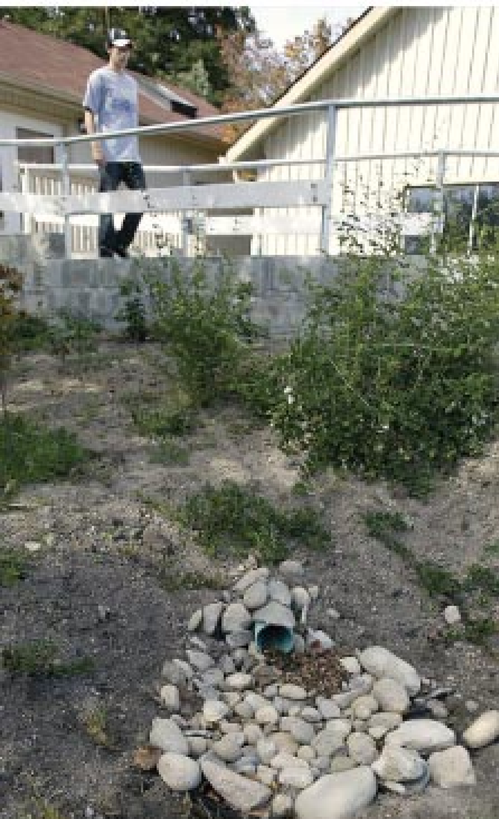
Levi Stuart, a volunteer at the Kitsap Conservation District office, walks past a rock garden. All the rain water from the building's gutters is directed to the rock garden, where it is filtered through the rocks and percolates back into the soil.
