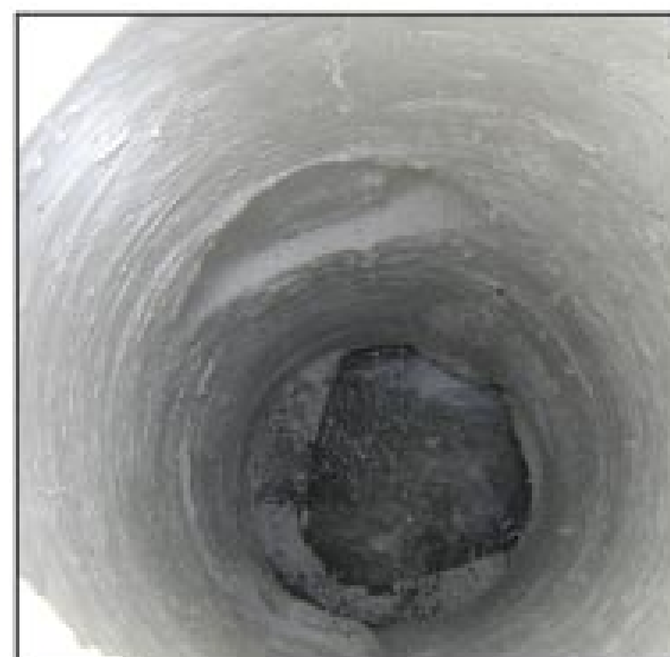
The concrete polymer paste restores manholes by filling voids. This manhole is ready for coating.
