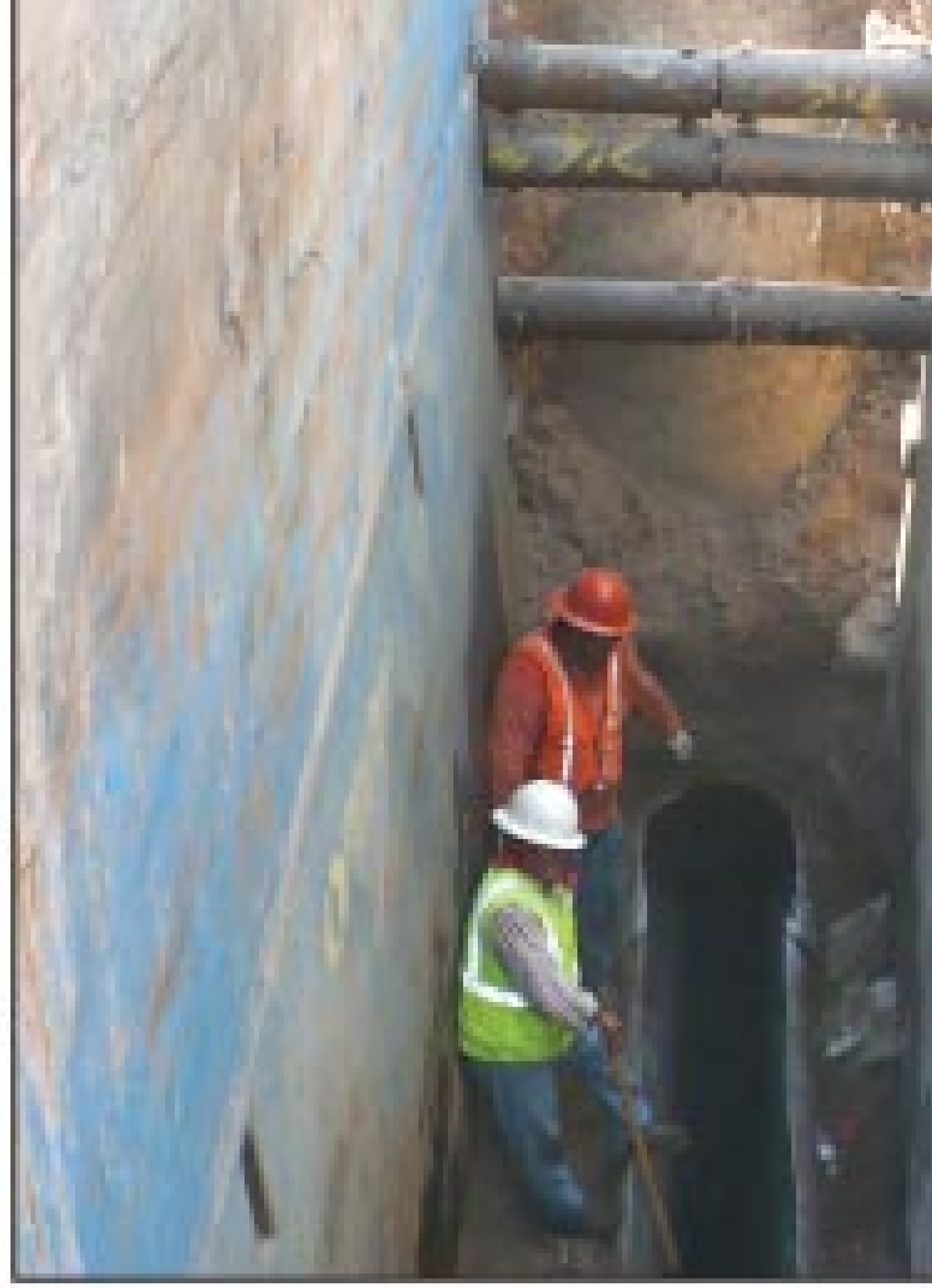
Workers from Achen-Gardner Engineering use slip lining for a trenchless pipe rehabilitation job. Achen-Gardner is a general contractor specializing in wet utility, roadway, and highway construction.
