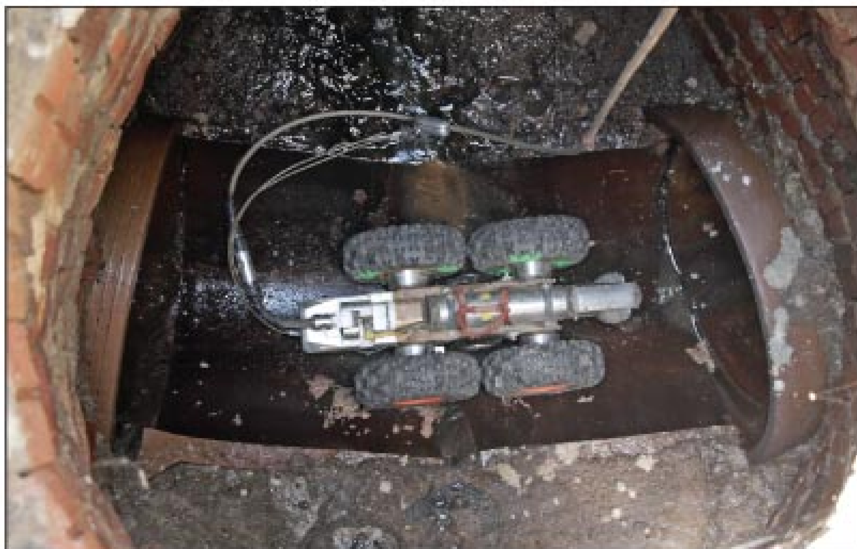
A CUES camera is deployed to inspect a 300-foot section of old vitrified clay pipe.
