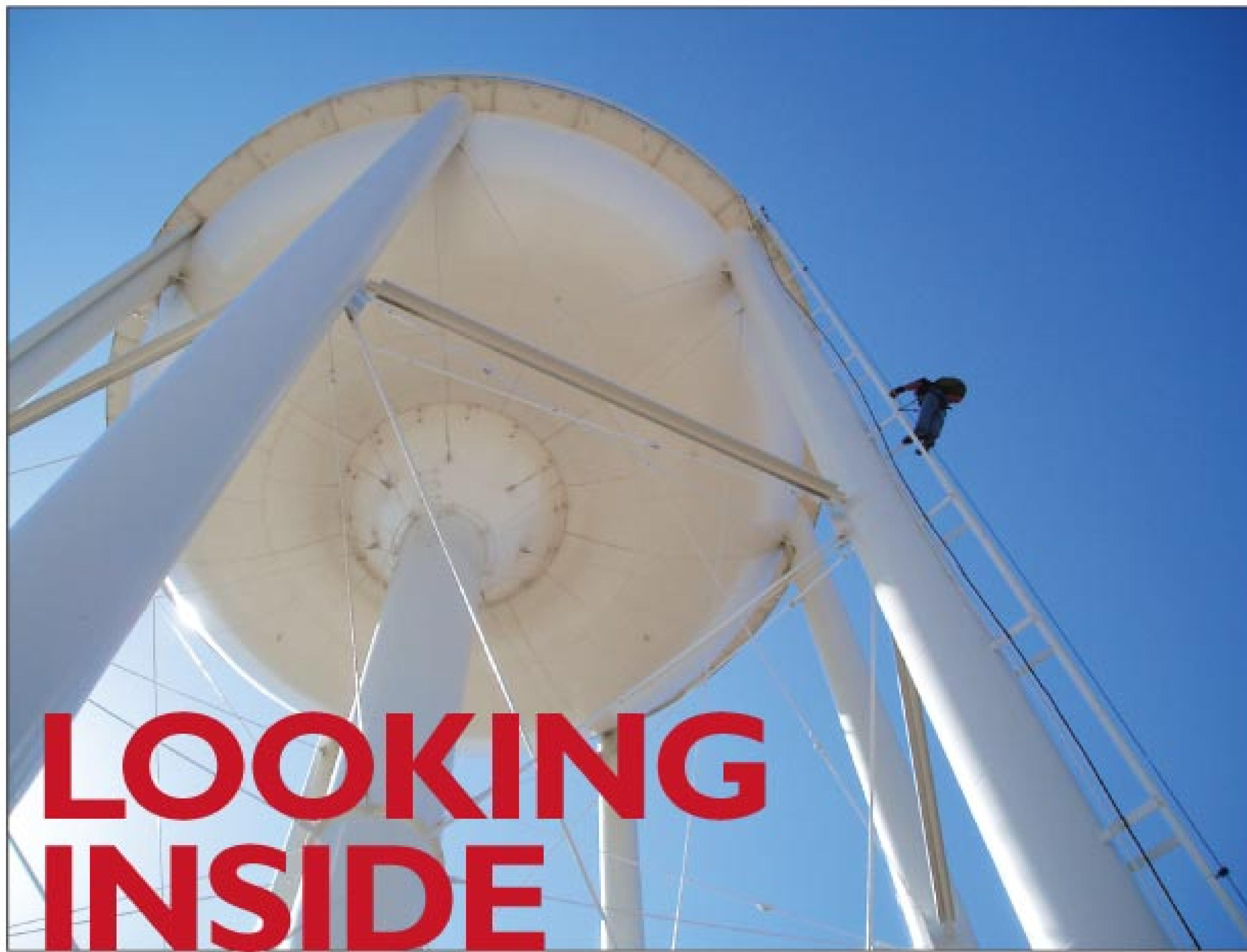
An inspector ascends a water tower for an inspection. (Photos courtesy of Ron Perrin)
