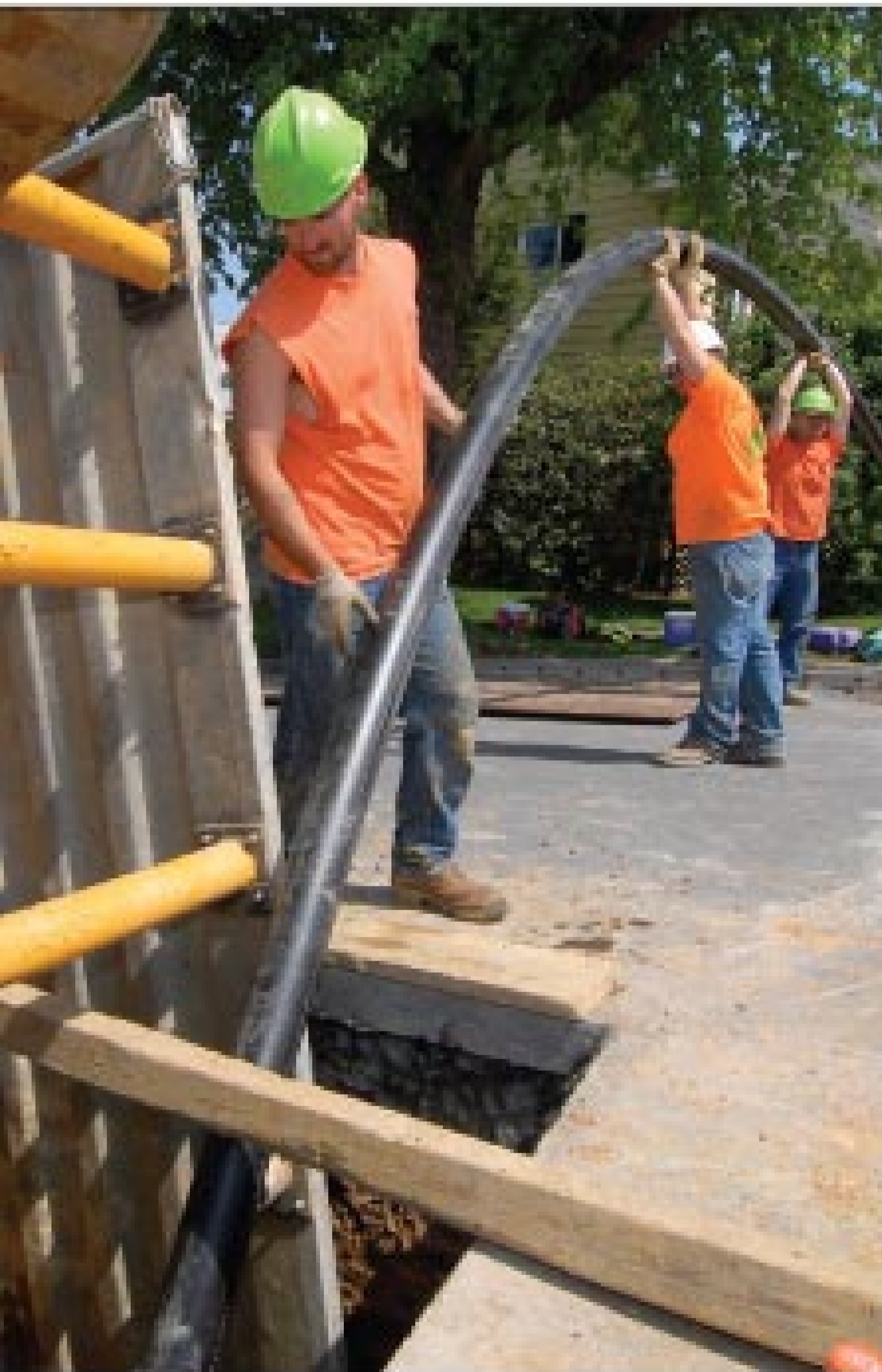
Steven Moyle (foreground) and co-workers of Pine Mountain Excavating guide a new 4-inch pipe on a bursting job. Pipe bursting and CIPP lining are trenchless options available to residents who must have their sewer laterals replaced or repaired.
