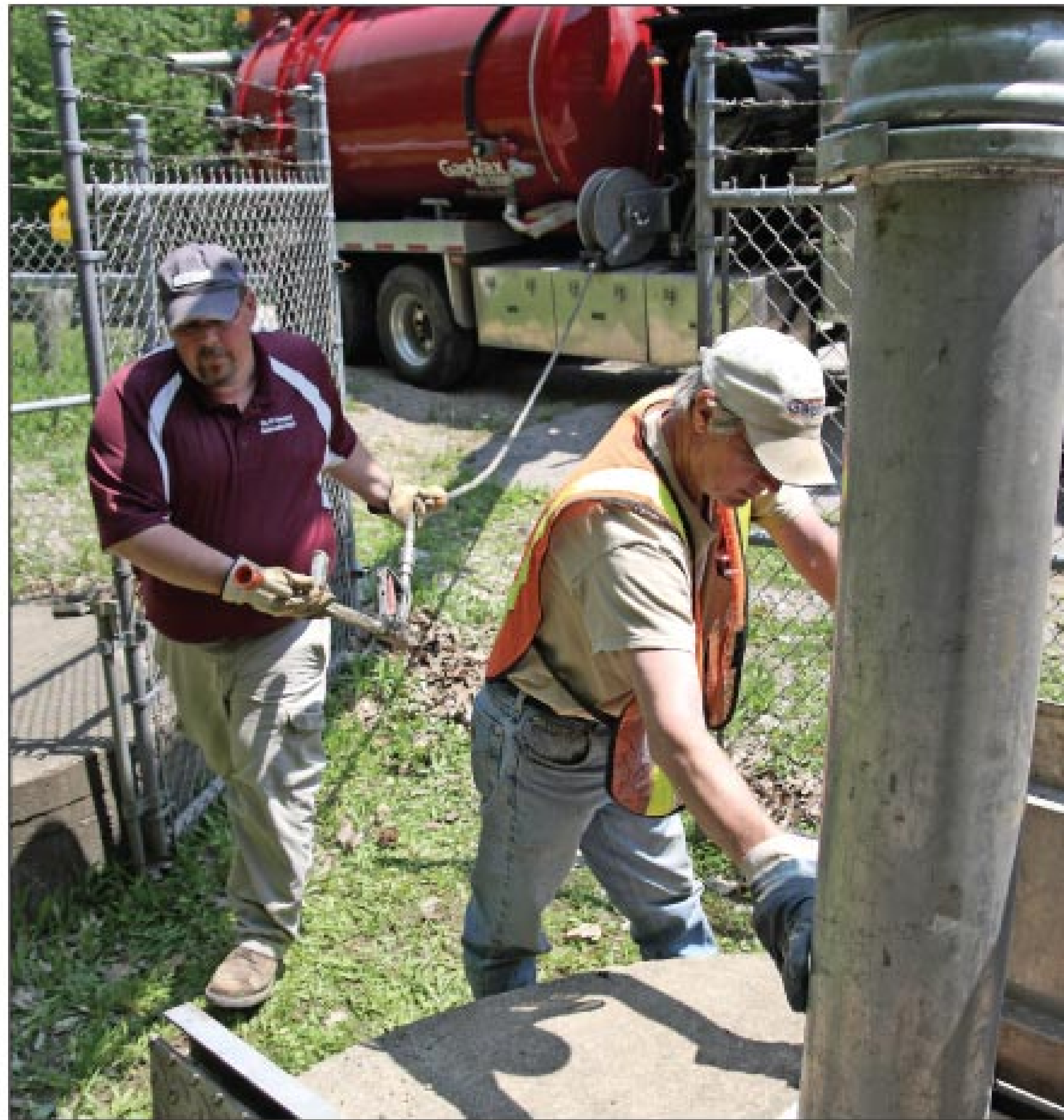
Wastewater superintendent Craig Pierce grabs the gun from the GapVax truck to help Jeff Pelow, jet operator, as he guides the vacuum tube into a lift station well.
