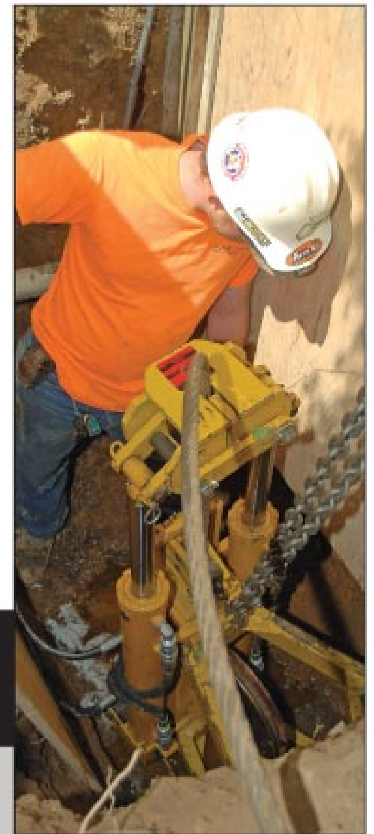
Russel Shemery of Pine Mountain Excavating keeps an eye on the Pow-R Mole PD-33 pipe bursting unit as it pulls the cable, bursting head, and new pipe through the old lateral.
