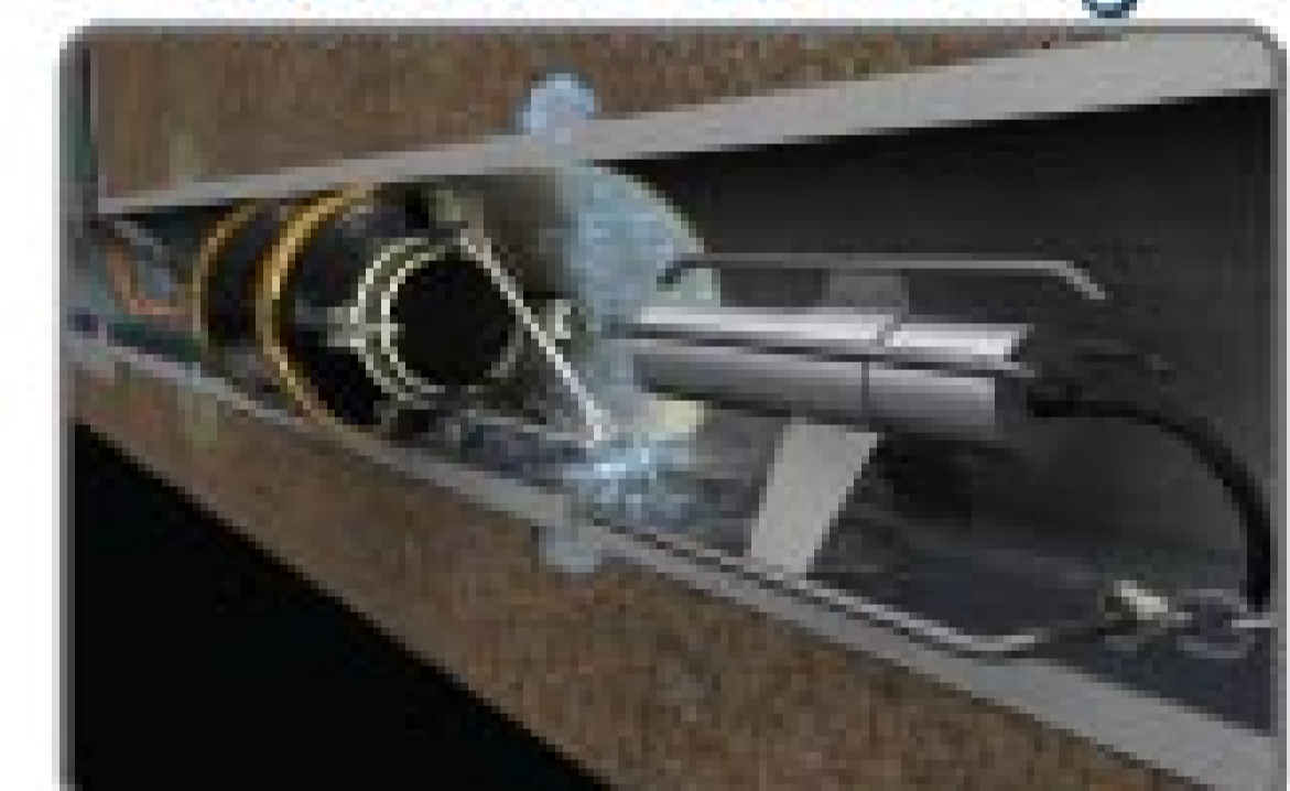
Leaking joint in mainline sewer
