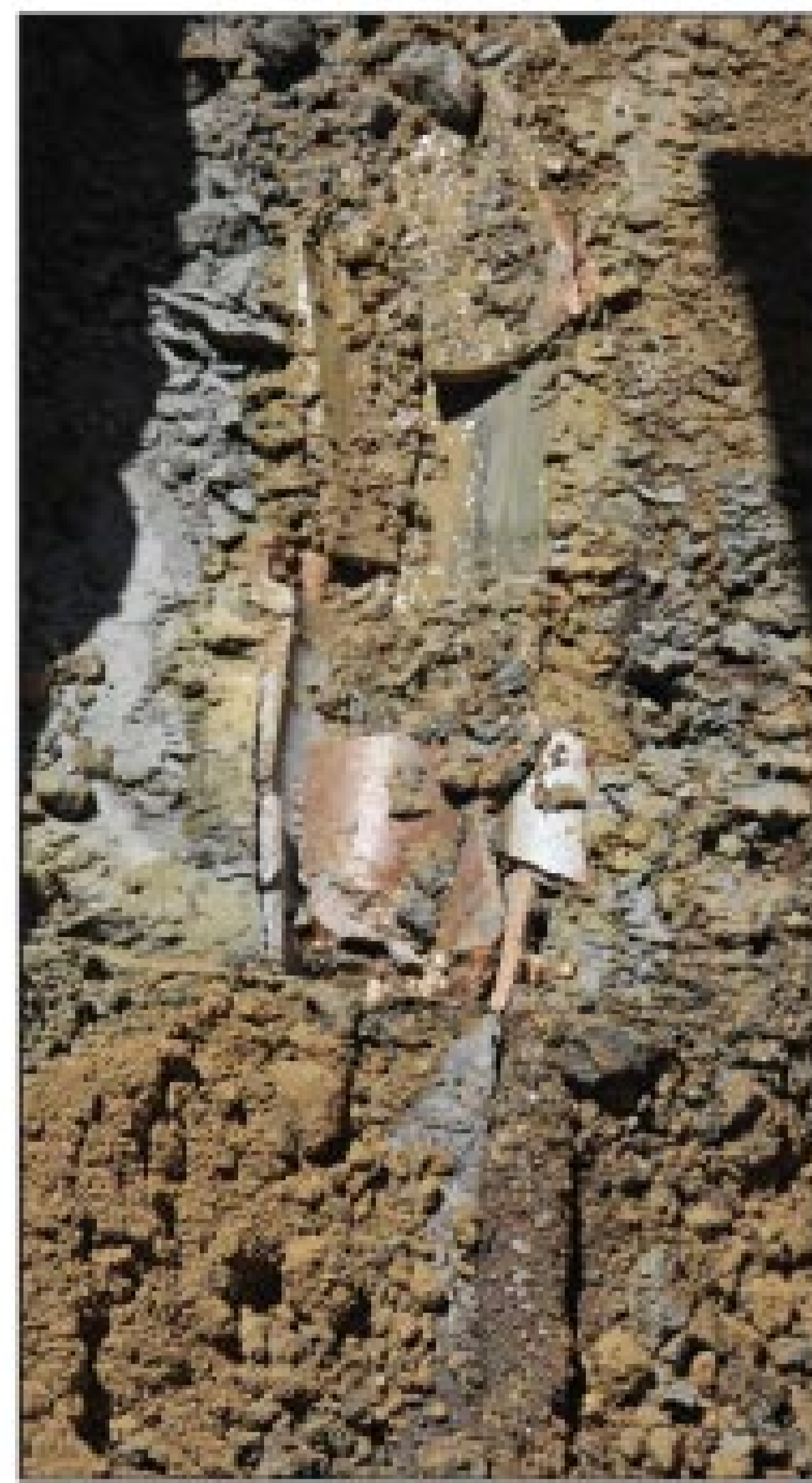
Timbers cover a 20-foot section of crushed vitrified pipe at dig site in Conneaut.
