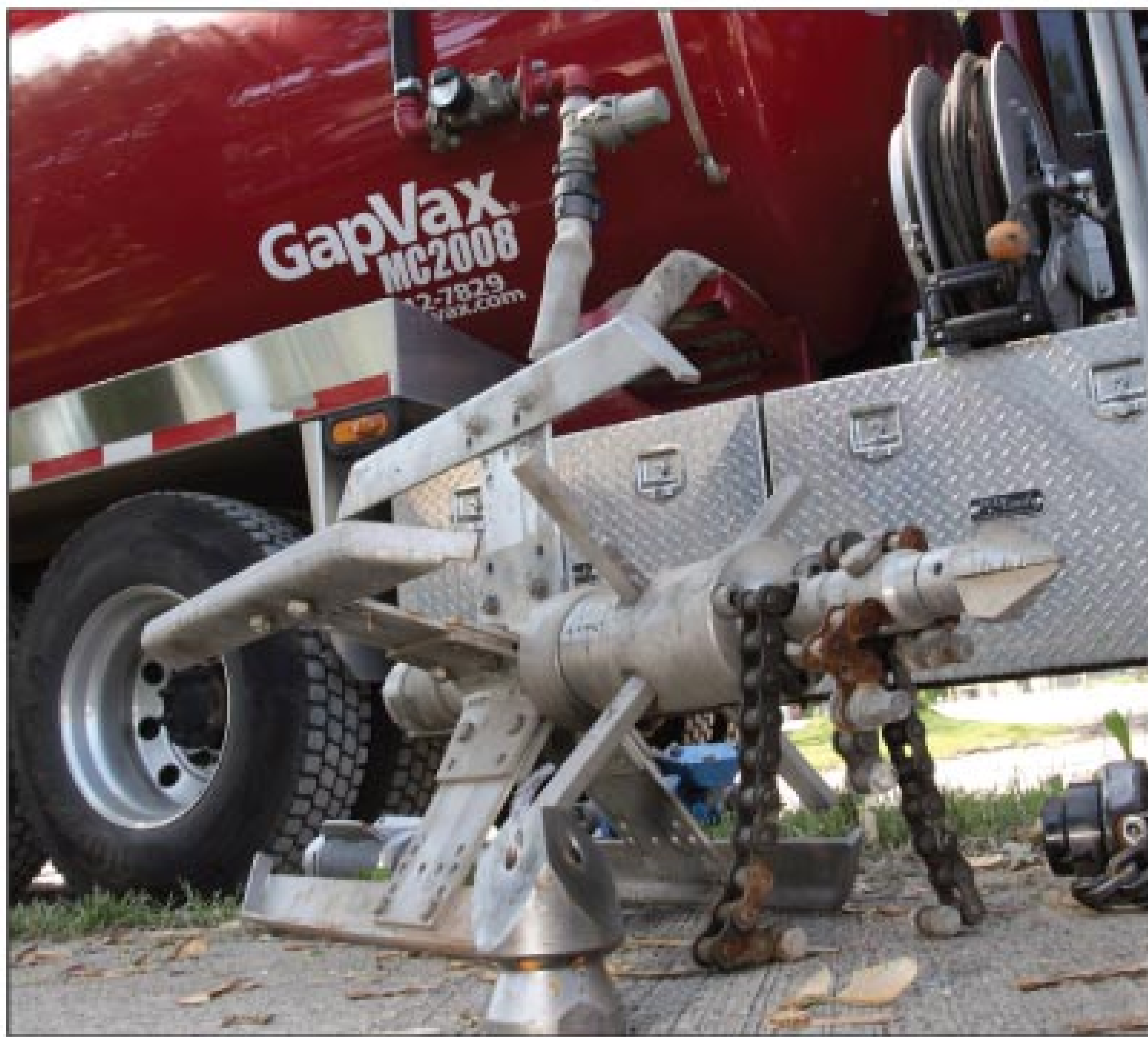
A Conneaut crew used a cutting nozzle to clear a 20-foot section of large-diameter wastewater pipe.
