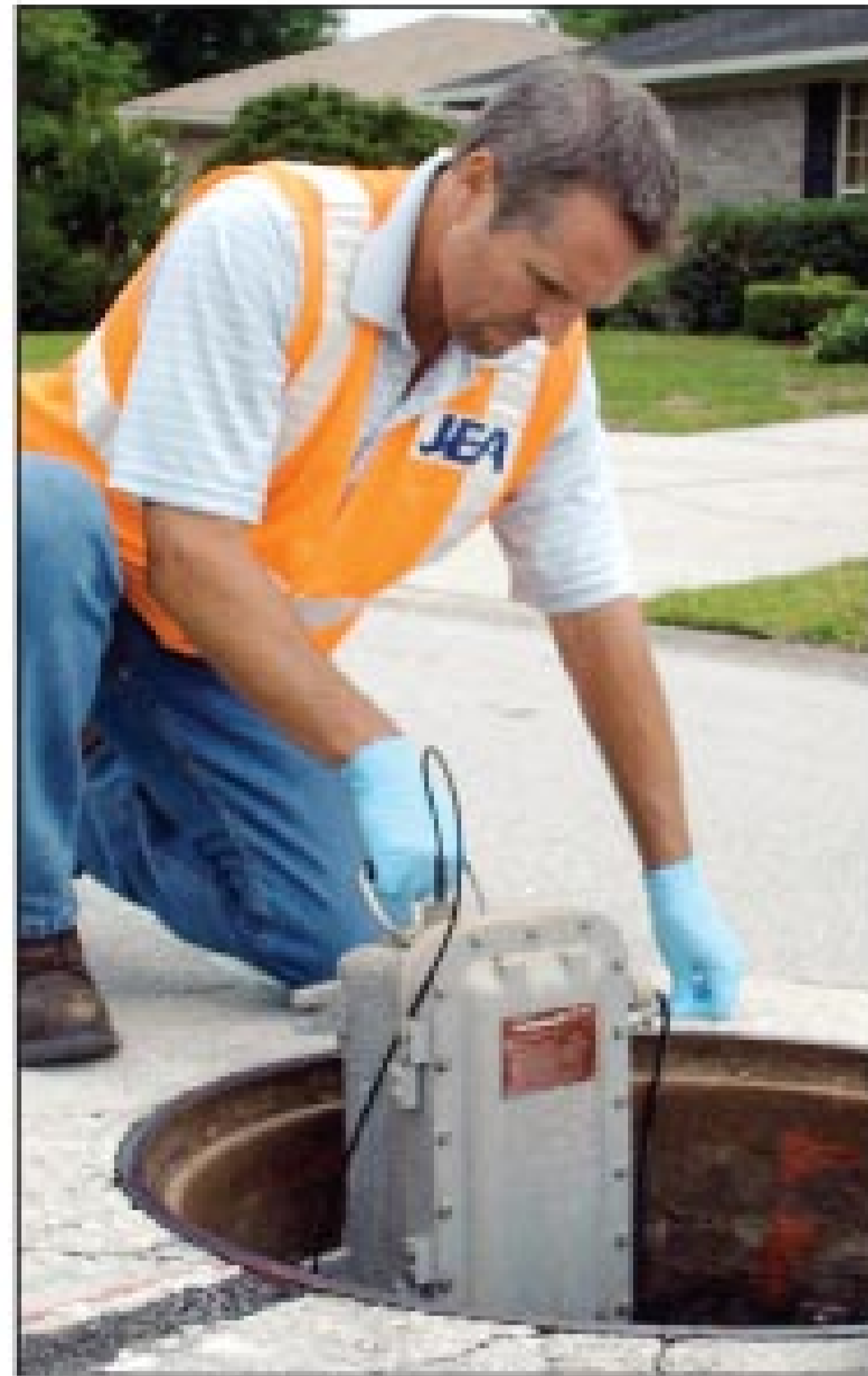
Rodney Williams, water and wastewater reliability specialist for JEA, lowers a remote manhole monitoring transmitter. The device has helped prevent 100 percent of SSOs at 17 monitored locations.
