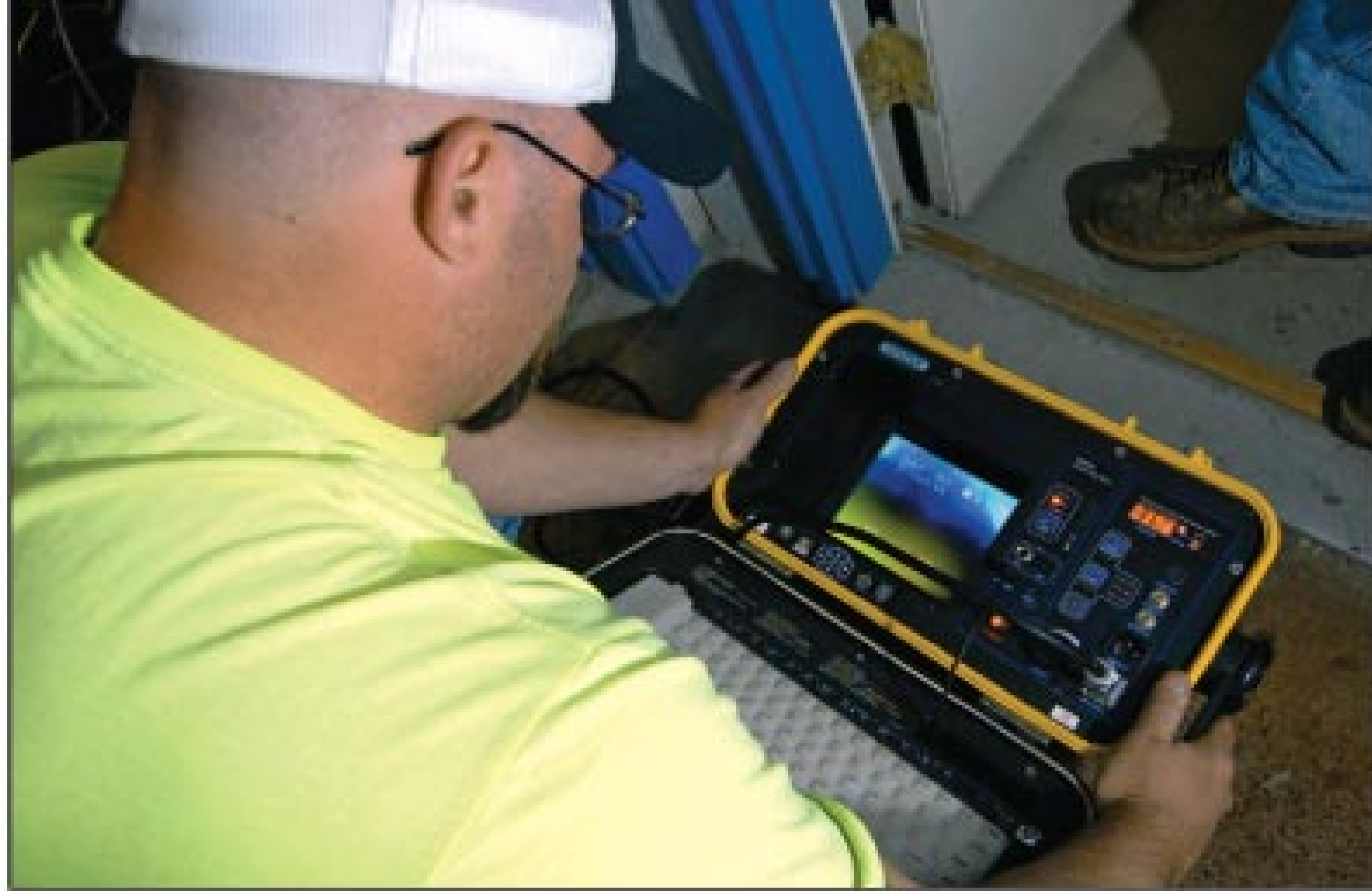
South Williamsport sewer technician Terry Kaichner uses a Vivax vCamDigital to follow the camera through a sewer lateral. The camera allows technicians to inspect the lateral for leaks.
