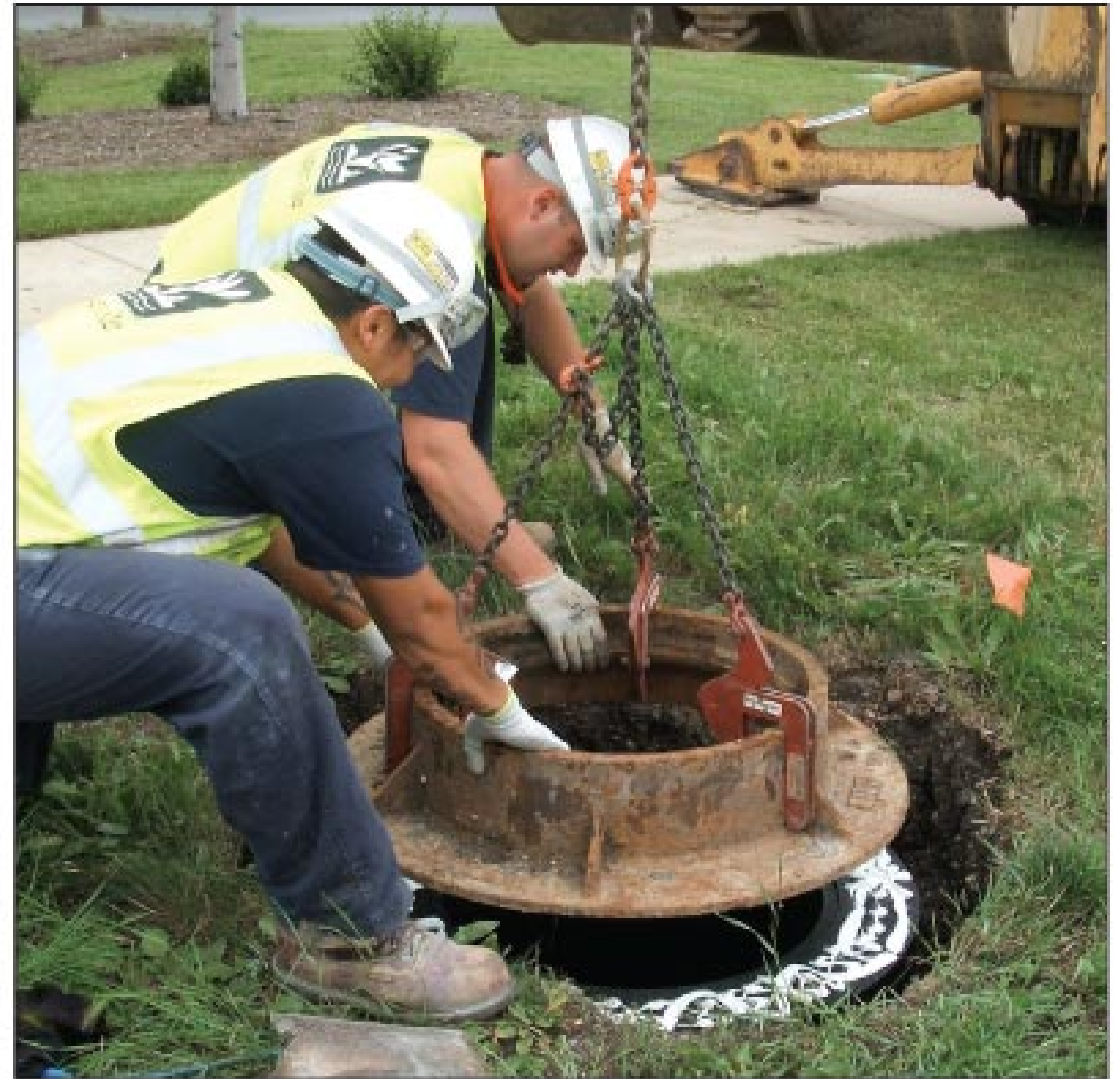
After Rick Flaar has covered the top ring with adhesive, he and Martin Alvarado lower the manhole frame into place.
