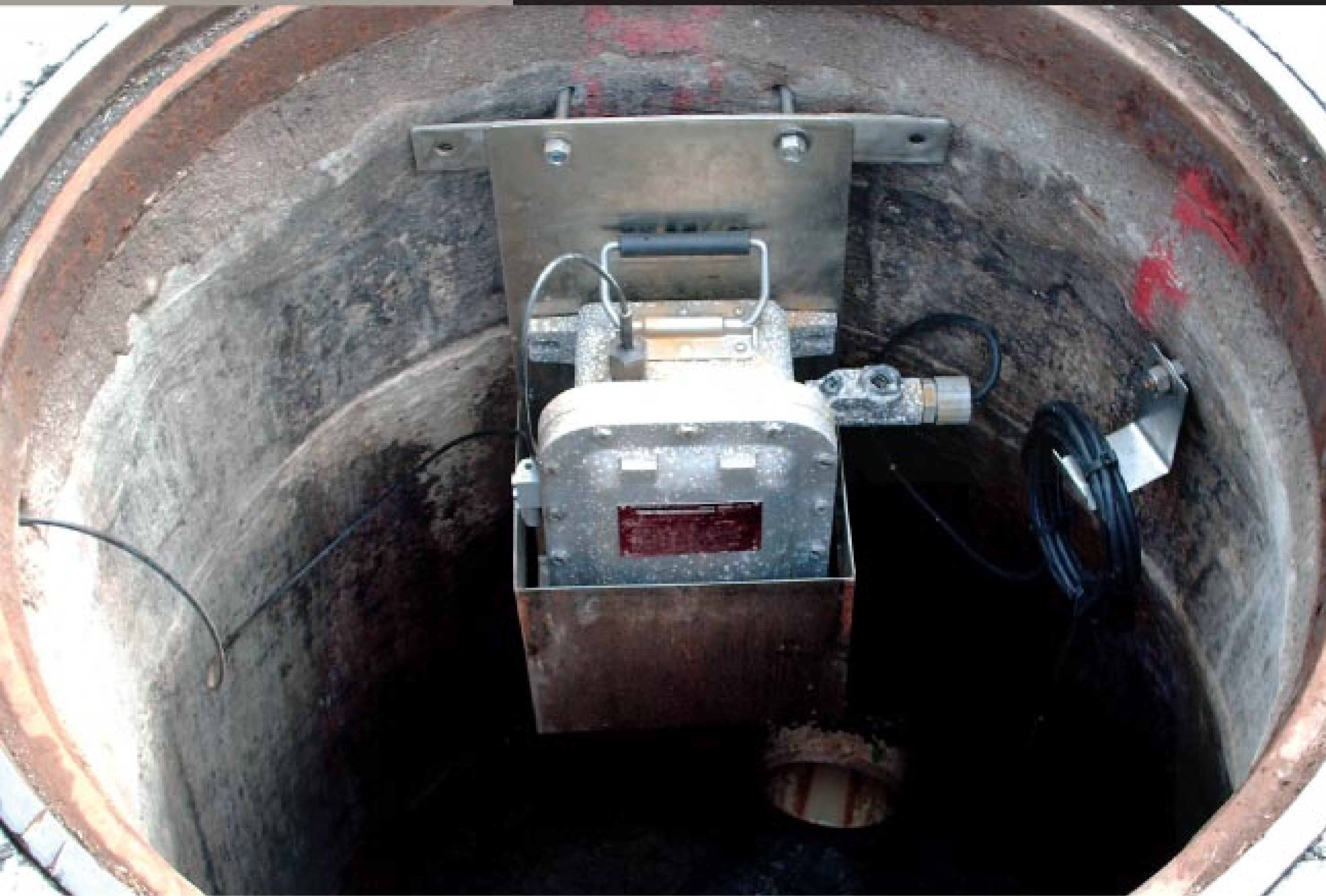
An explosion-proof enclosure with cradle secures the monitoring device to the manhole wall. A small external antenna is mounted on the bracket to the right and exits the left side of the manhole. (Photos courtesy of Rodney Williams)
