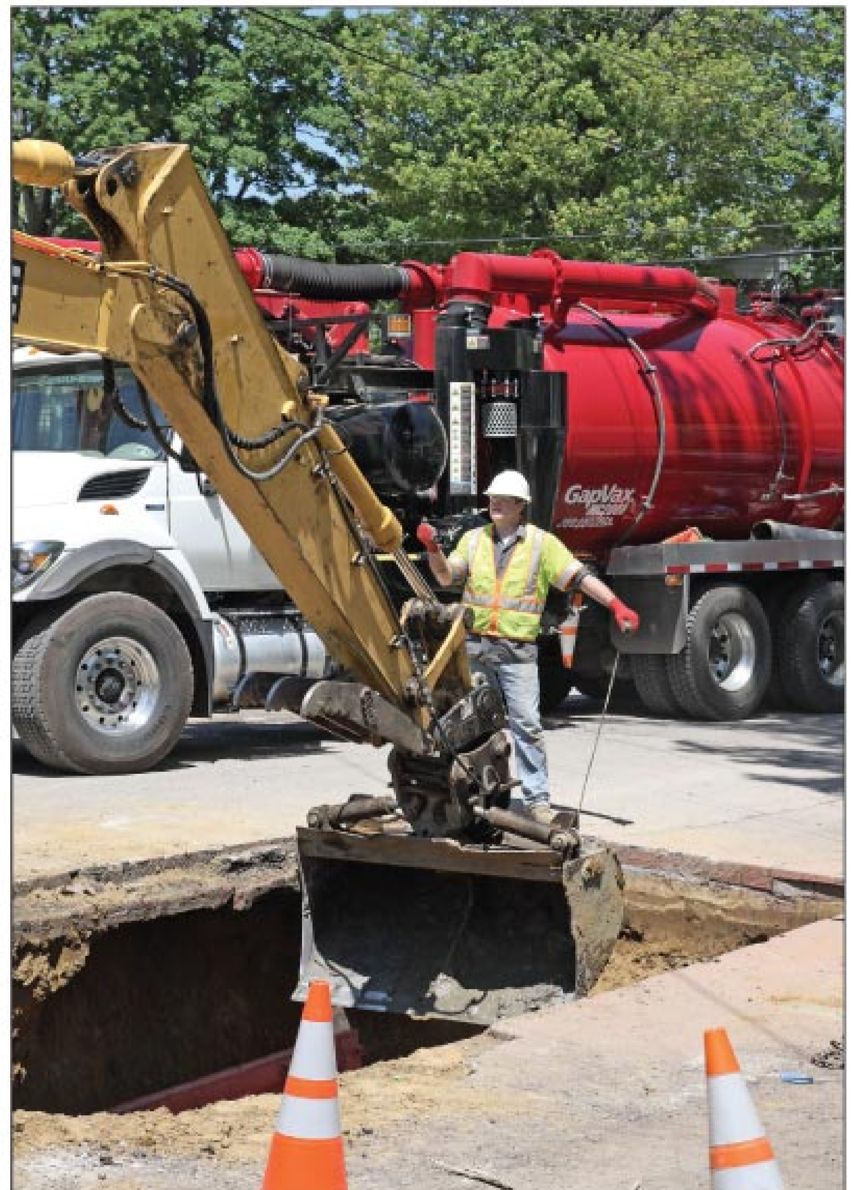
Maintenance worker Dan Rozalski guides an excavator on a sewer pipe repair job.
