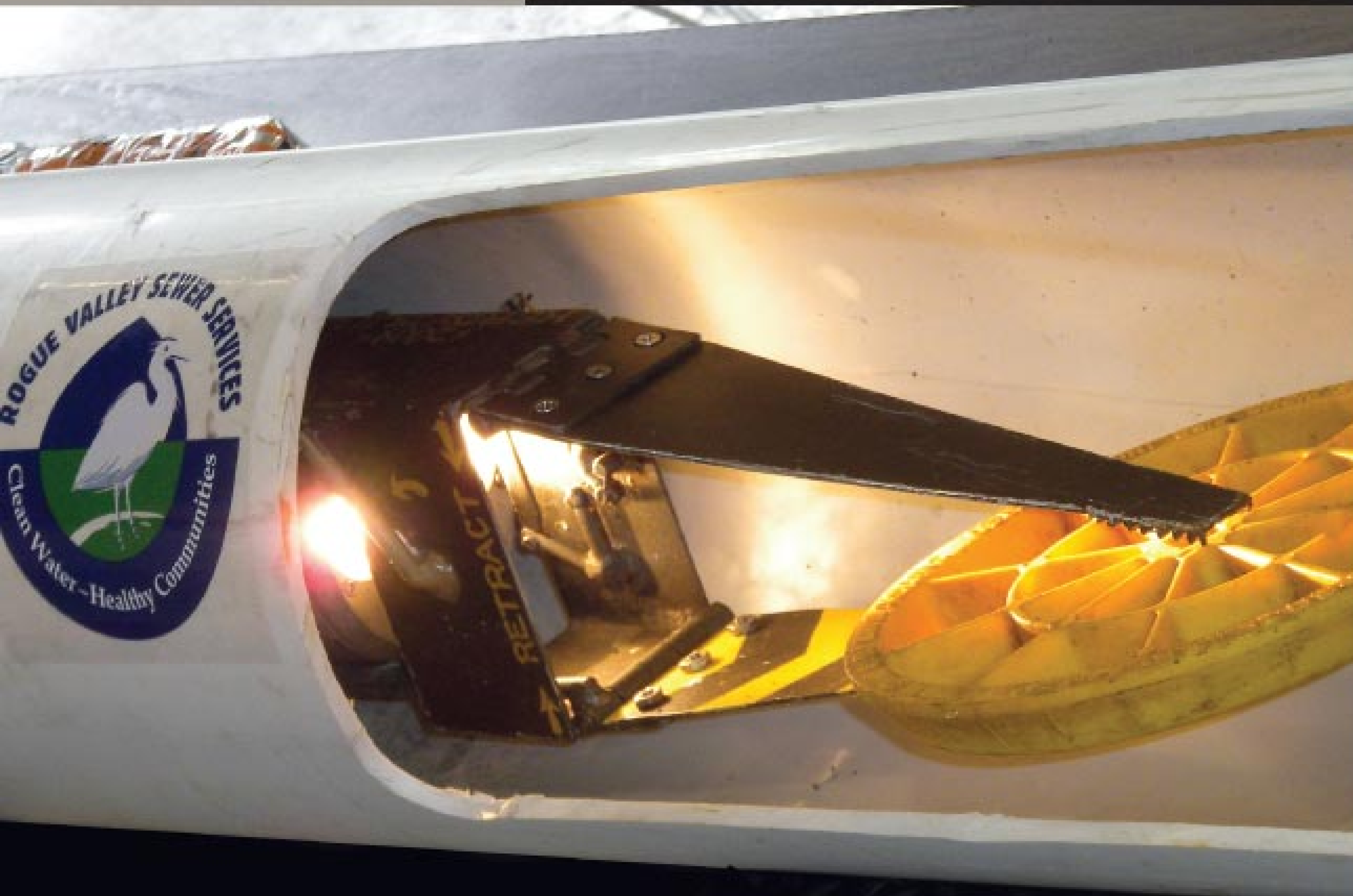
The Pipeline Piranha's 9.5-inch-long jaws with carbide chips glued on the ends grasp a 10-pound plastic mechanical plug. (Photos courtesy of Rogue Valley Sewer Services)
