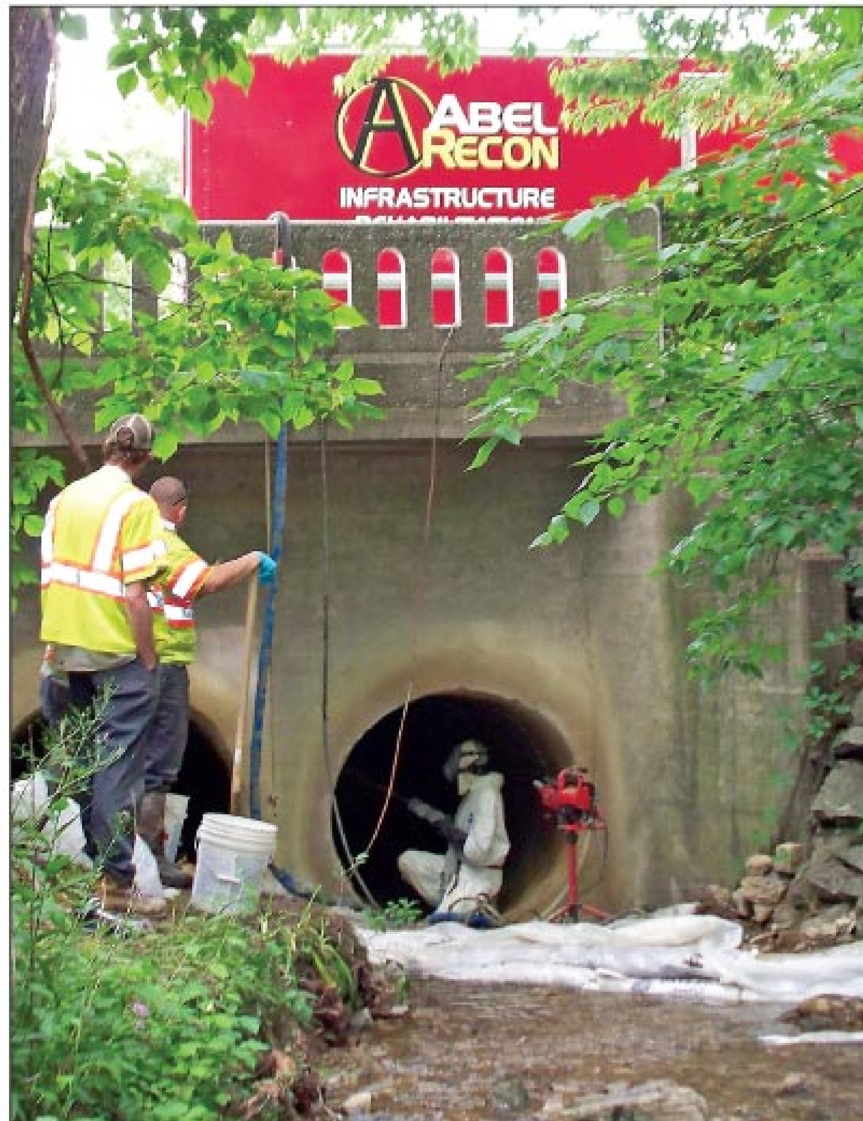
Joe Knight, spray application technician, applies SprayWall lining to the host pipe.
