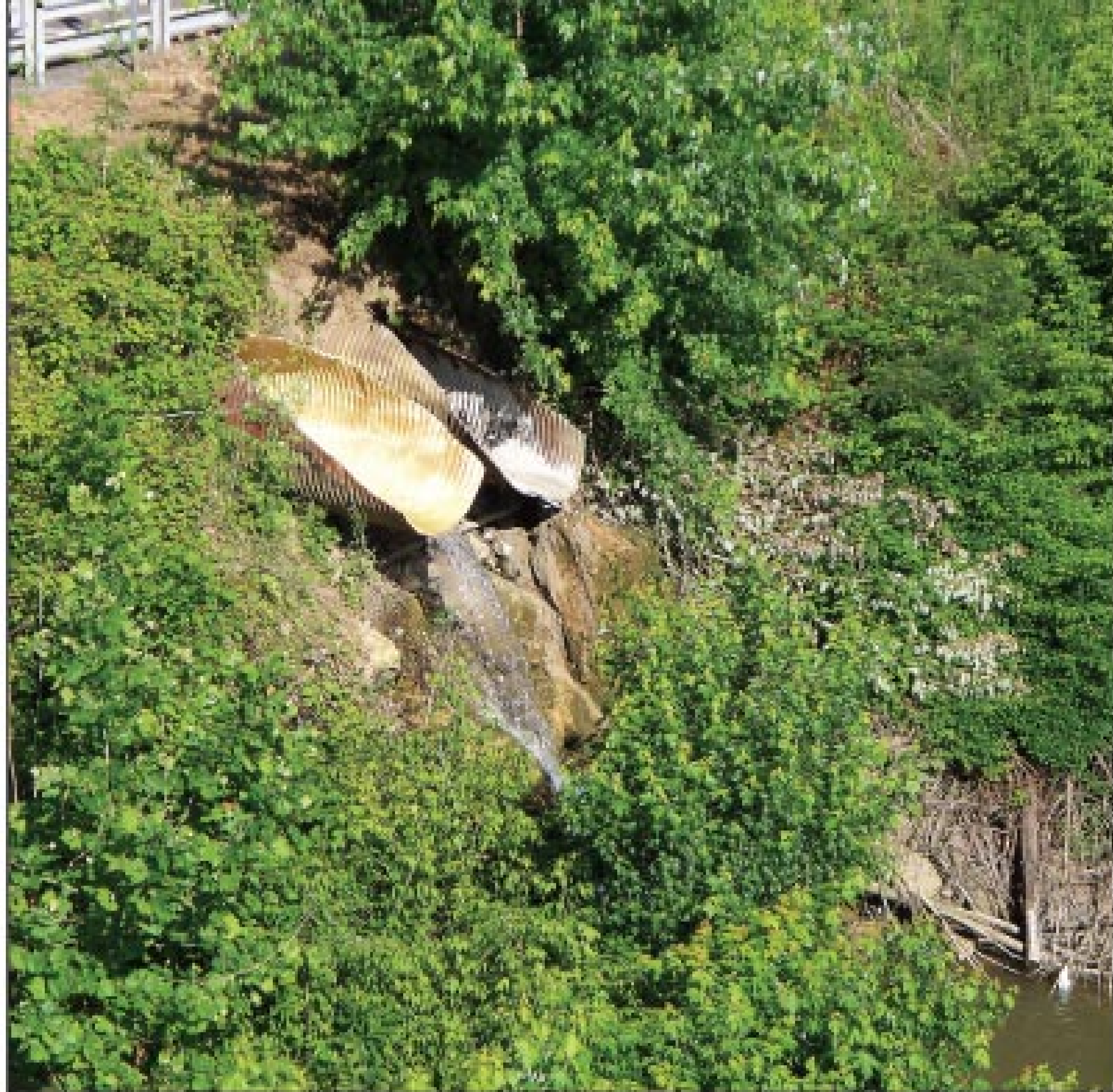
The foreground pipe is shown lined and is back in service while the other pipe has had its flow diverted while being prepared for lining. The pipes discharge directly to the Susquehanna River.
