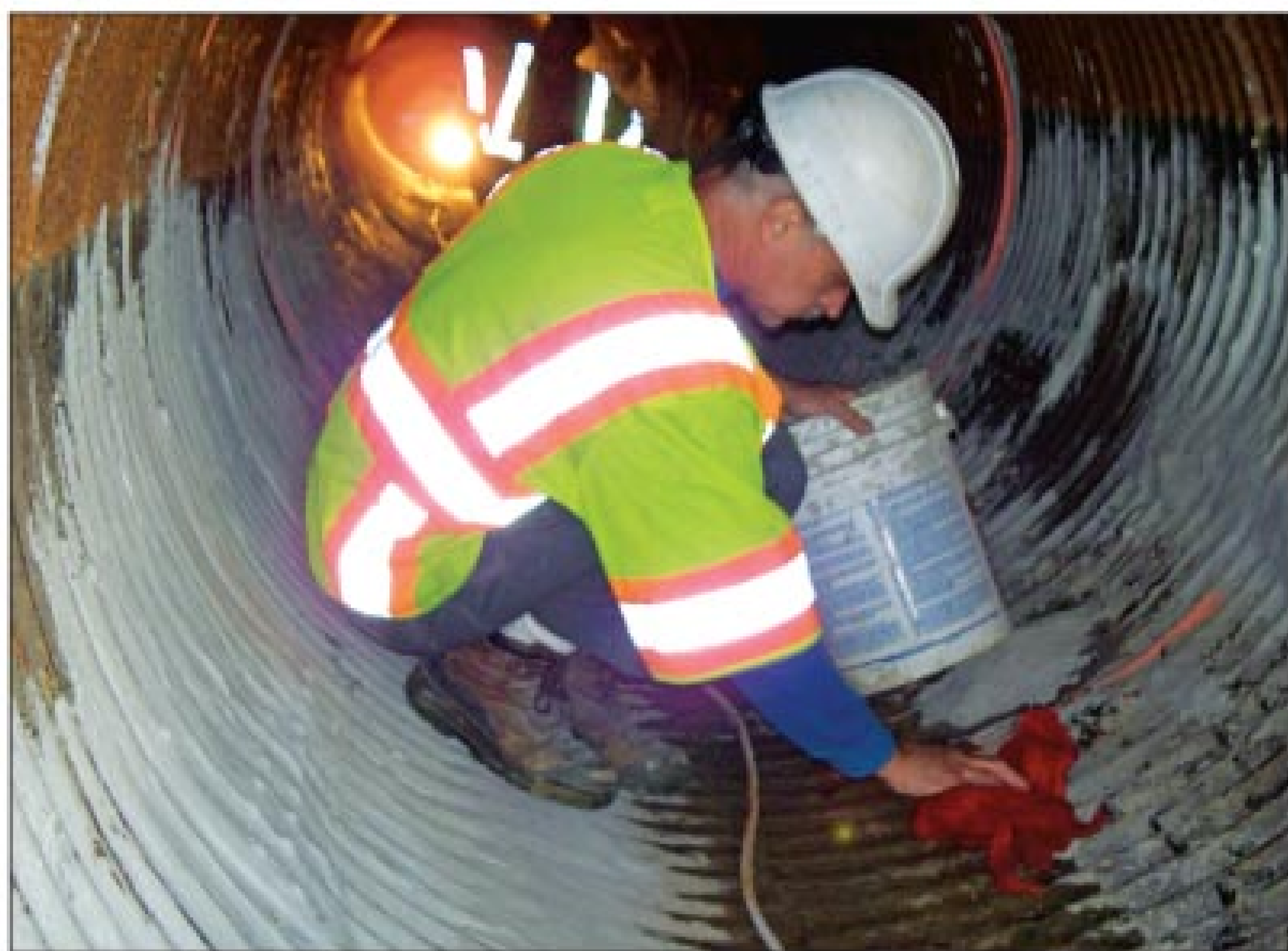
Charlie Mitzel, spray application technician, uses absorbent material to remove water from between the corrugations in the culvert before final drying of the pipe.
