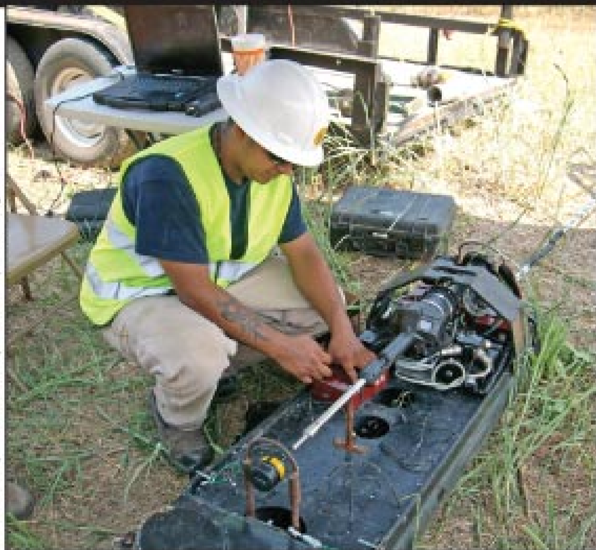
A technician in the field readies the FlyEye system for an inspection of an interceptor.
