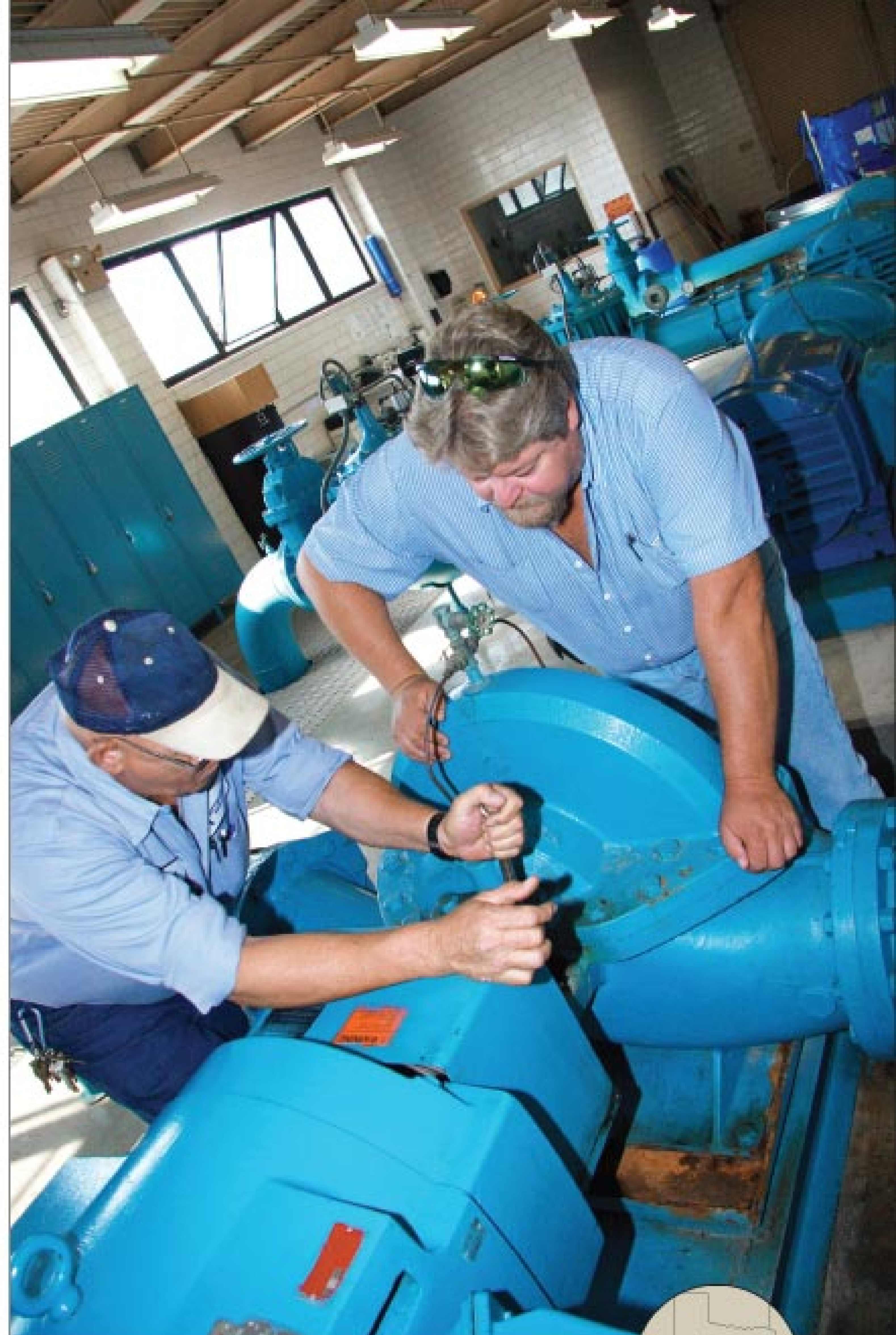
Operators Mike Smith (left) and Chris Zeitner adjust the packing on a 2,400 gpm pump. (Photography by Kay Taylor)
