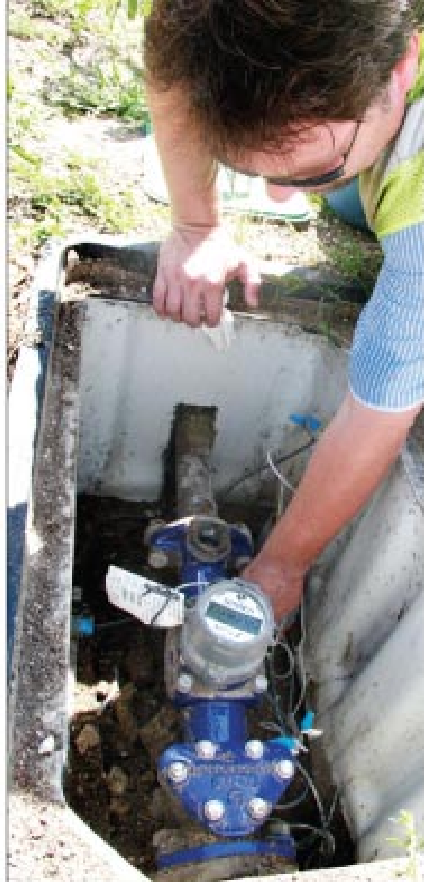
Assistant supervisor of water Clay Culver checks a Sensus radio-readable meter installed at the new Killeen Police Department.
