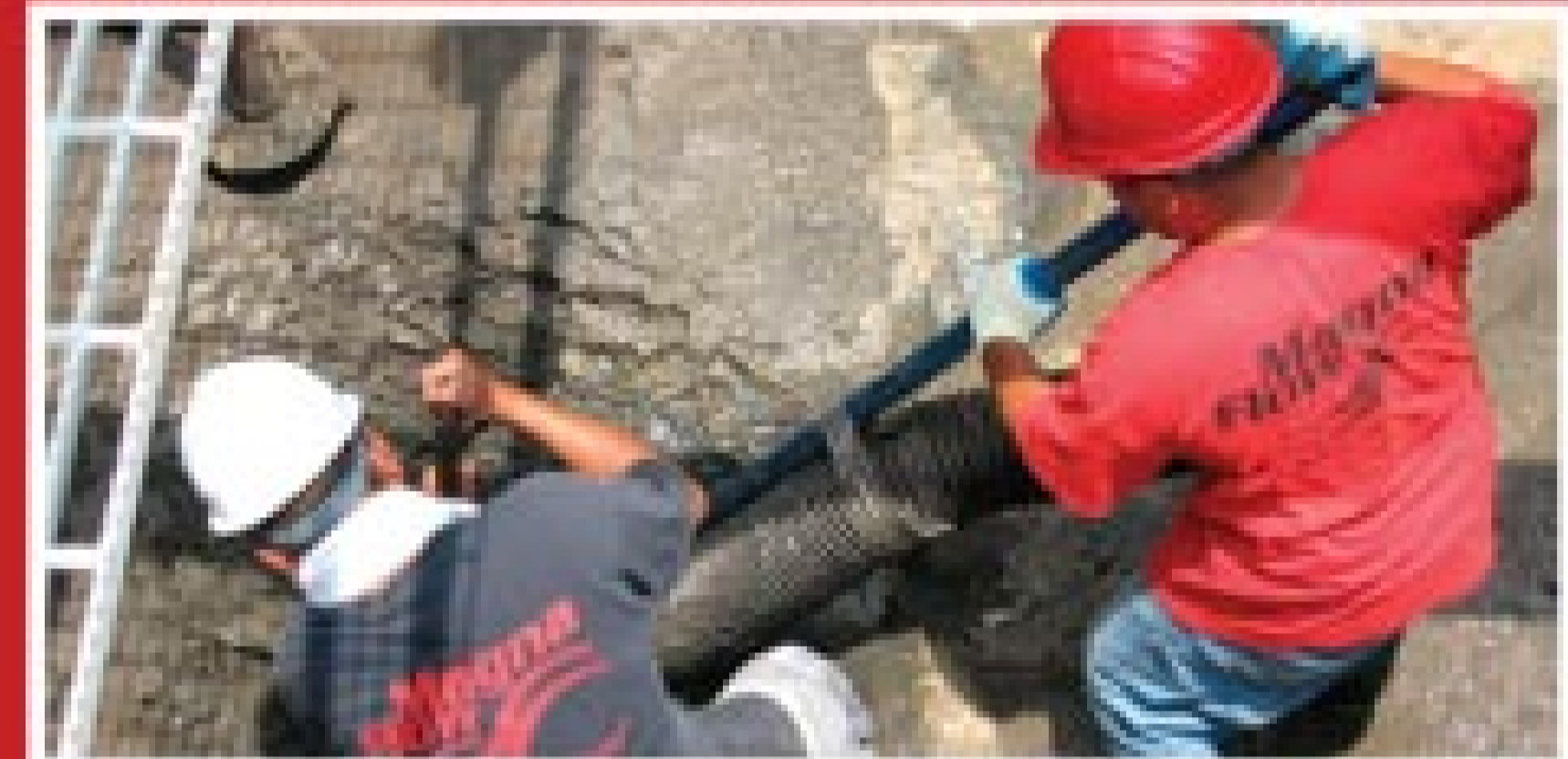
Total Plant Cleanouts
