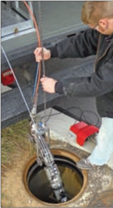
Rausch Electronics operator Jordan Newcomer uses the foot control to operate the power as he introduces the system into a manhole.
