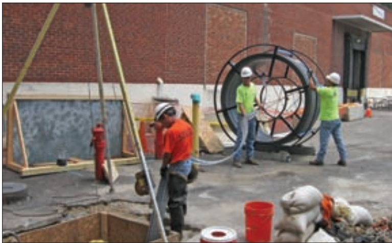
Metropolitan Sewer District employees feed SPR material through a manhole to the self-propelled spiral winding machine.
