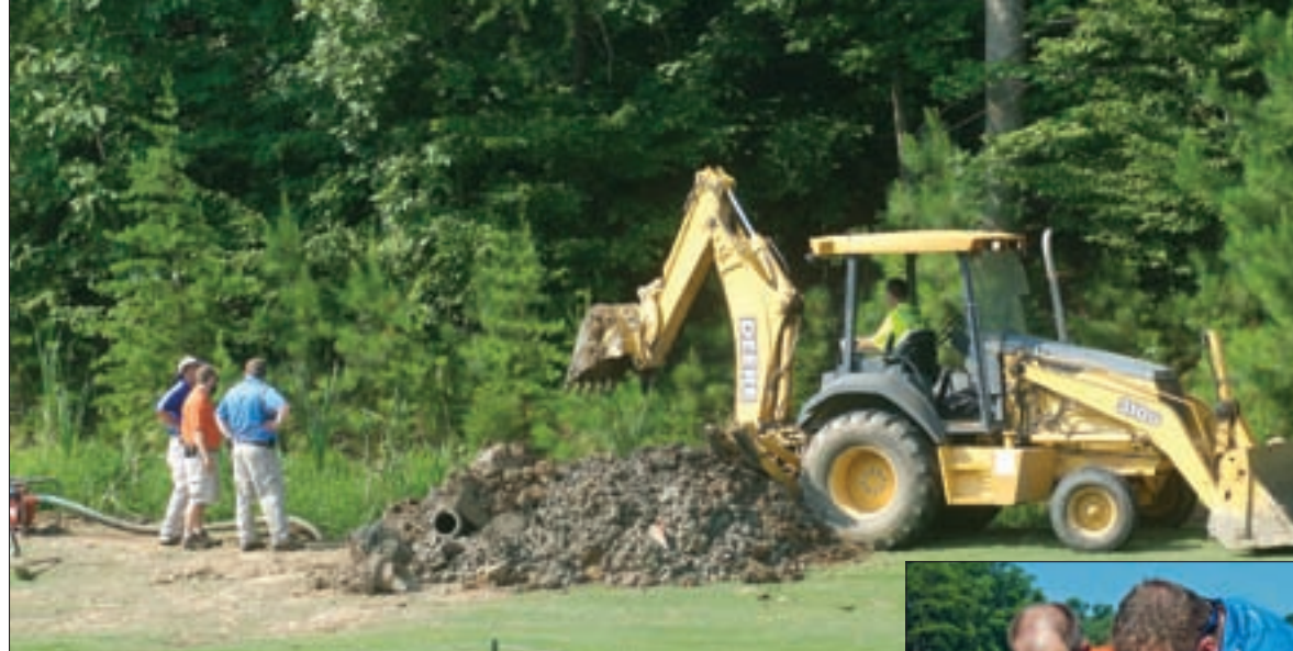
A stormwater department crew digs a trench between two ponds on the Tega Cay golf course to remedy a poor drainage system.
