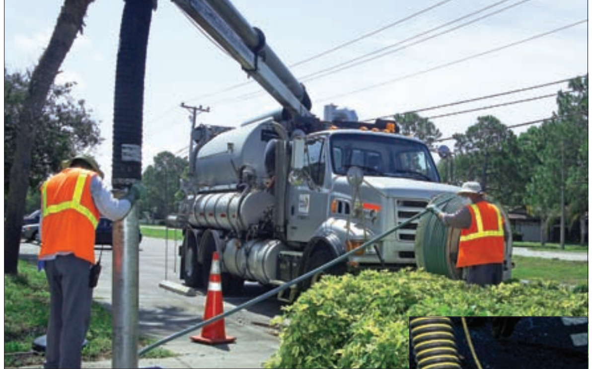
Utilities specialist 2 Jeff Gallo (right) pulls out high-pressure hose while utilities specialist 1 Steve Griffith monitors the vacuum tube.
