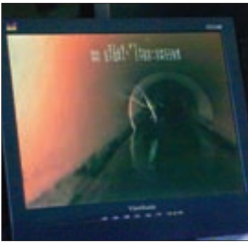
A video inspection reveals root intrusion at a sewer pipe joint. Roots are among maintenance issues Pinellas County crews face regularly.
