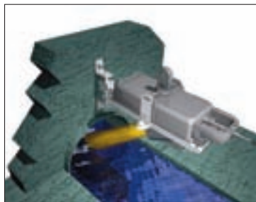
A four-bolt permanent bracket mounted on manhole walls suspends the Flo-Dar sensor above the stream. The flowmeter combines digital Doppler radar velocity sensing technology with ultrasonic pulse echo depth sensing to measure flows.
