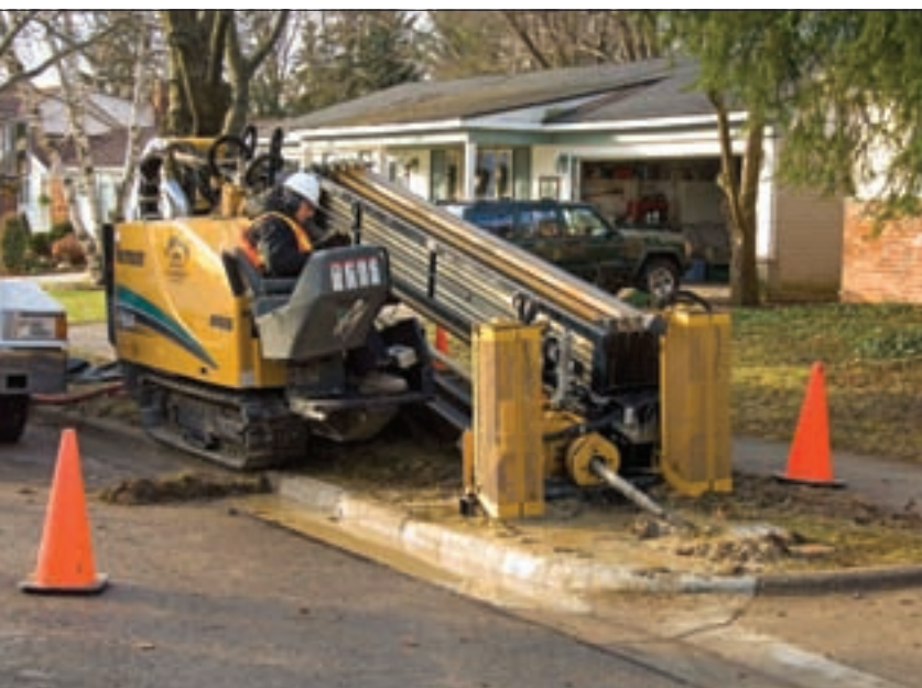
Horizontal directional drilling is gaining favor for pipe replacement when examined in a “whole project” context that includes the costs of surface disruption and subsequent repair. (Photos courtesy of Vermeer Corp.)
