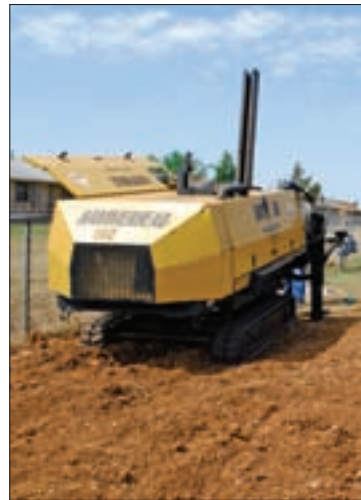
A HammerHead HG12 winch pulls a length of pipe on a Lawton sewer rehabilitation project.
