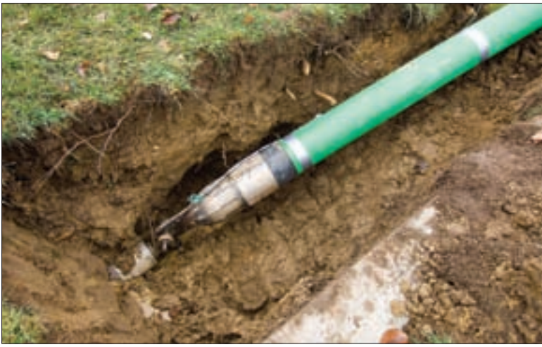
HDD can enable replacement of water and sewer pipes with a minimum of disruption to streets, sidewalks and landscapes.
