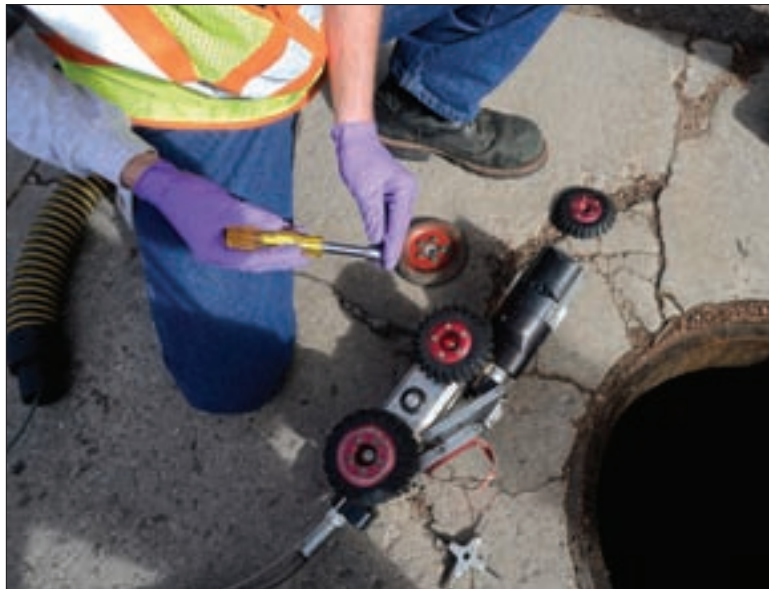
A crew member prepares to perform a CCTV inspection with an Aries camera outfit in a system using Pipeline Assessment and Certification Program defect coding from NASSCO.
