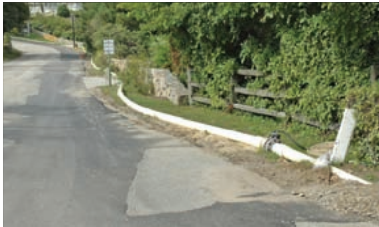
During main replacements, residents received water through bypass piping with locking groove joints and temporary service taps. The 200 psi class Certa-Lok Yelomine piping from CertainTeed allowed quick assembly, had good hydraulic characteristics, and required minimal piping restraint.
