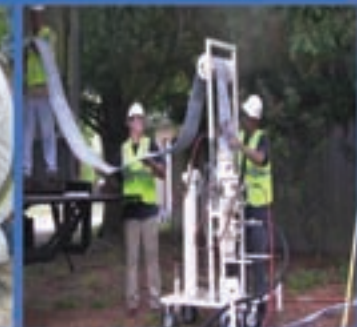
Perma-Main™ Continuous Air Inversion
