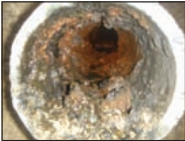
The tuberculation in the 4-inch cast-iron water main reduced flows by 50 percent.
