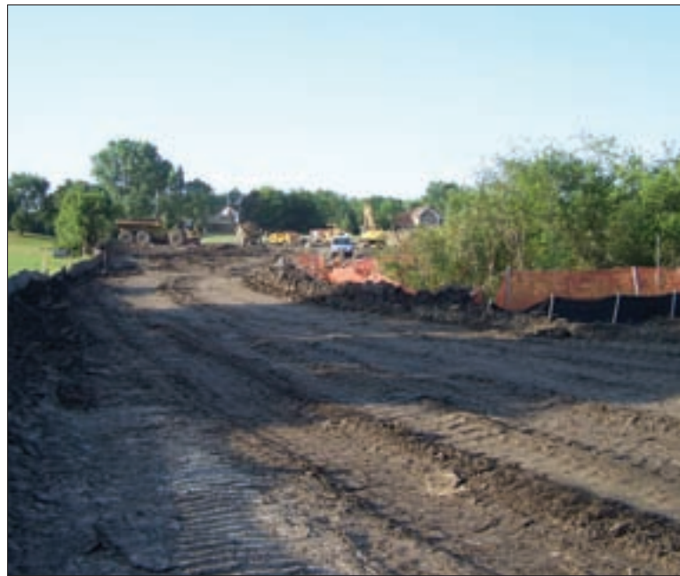
The village of Green Oaks used township property to create a flood basin in an 80-acre field overgrown with invasive buckthorn. (Photo courtesy of Libertyville Township)
