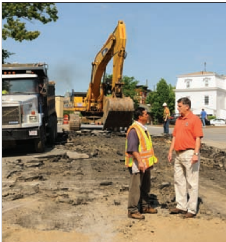
Leominster Public Works director Pat LaPointe (right) talks with assistant director Ray Racine on a job site for a project involving road reconstruction and water, sewer and drainage improvements.
