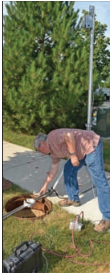
Guenter Schaarschmidt sets a support bracket to hold the pole that positions the wireless receiver at the bottom of the manhole. Behind him is the Wi-Fi transmitter, which will send the camera signal back to the Wi-Fi receiver mounted on the truck.
