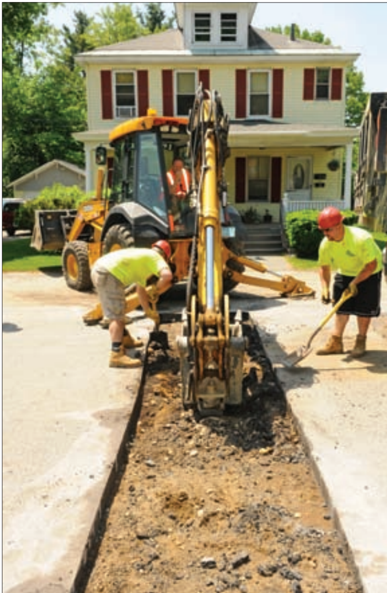
Truck driver John Bessette, equipment operator Mike Russo and laborer Shaun Booth prepare a job site for replacement of an outdated drainage pipe.
