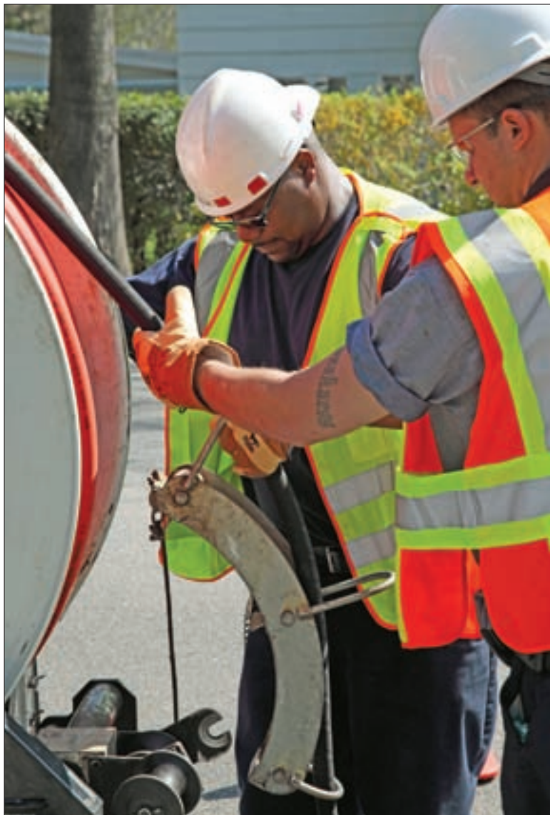
Team members like senior servicer Kenny Bunn , left, and attendant Tyler Olsson use a variety of jetting nozzles on the district's Vactor truck to clean pipes effectively in varying applications.
