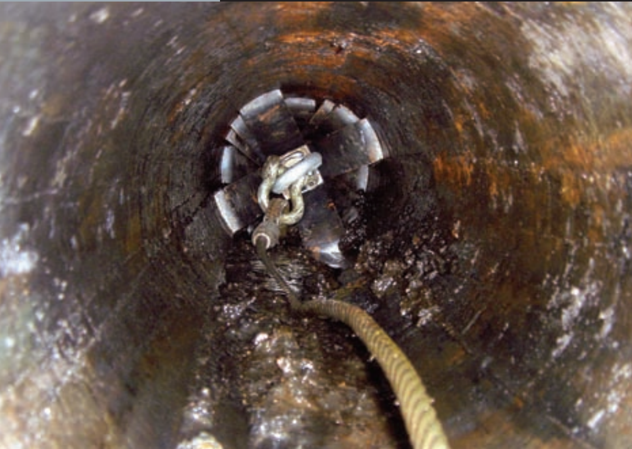
The drag scraper is pulled through the pipe to clean the walls before epoxy lining. Note the chatter marks on the walls. (Photos courtesy of Triton Lining Technologies)
