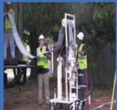
Perma-Main™ Continuous Air Inversion
