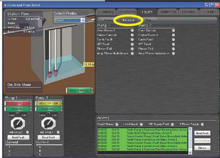
FIGURE 5. The Faults tab includes a sub-tab for monitoring electrical fault conditions.
