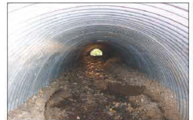
The culvert became filled with gravel and rocks after a June 2008 rainstorm.
