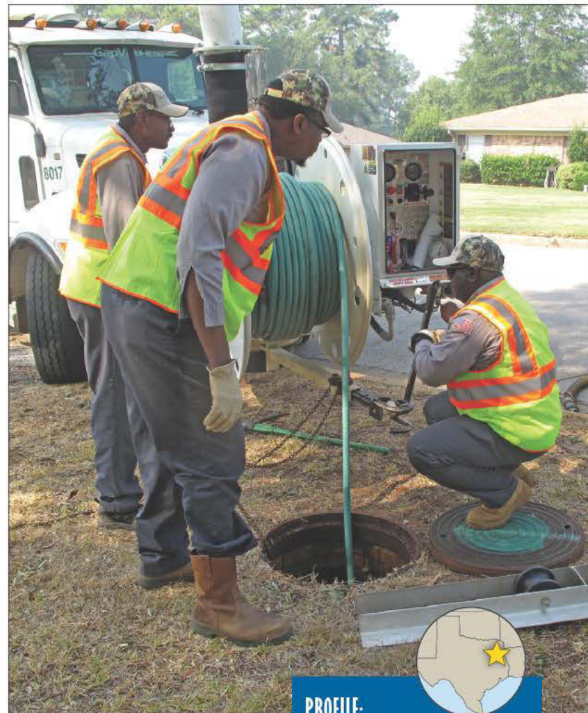
From left, maintenance workers James Pegues and Damien Reese and crew leader Vernon Jackson send a jetter nozzle into a residential sewer. (Photography by Pete Litterski)
