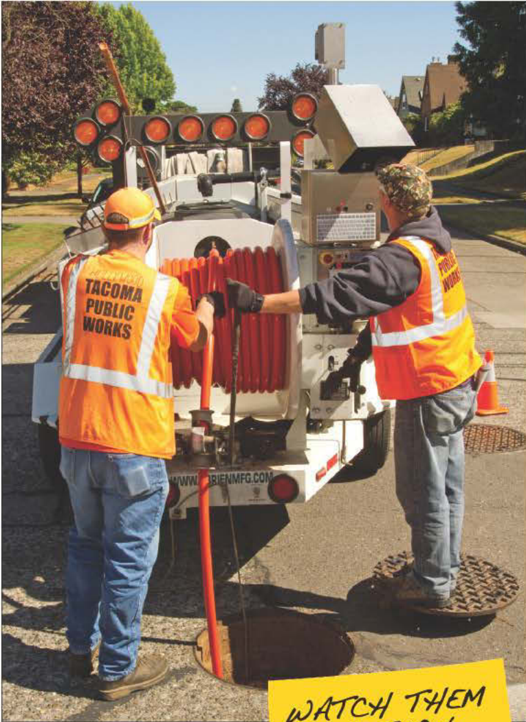
Ryan Welander, left, and Troy Ihlen pull the Kleen-Vue system back to the trailer with the hose reel. Ihlen continues to inspect the pipe on the way back to the trailer.
