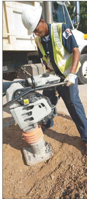
Utility technician Aaron Hillard tamps the soil with a Multiquip tamper after connecting a new service line.
