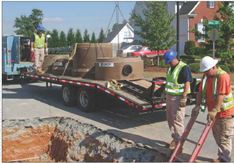
Gwinnett County workers prepare to install the sections of a composite manhole.
