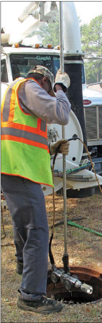
Maintenance worker James Pegues lowers a tractor-mounted camera from RapidView into a manhole to inspect a root-clogged line.
