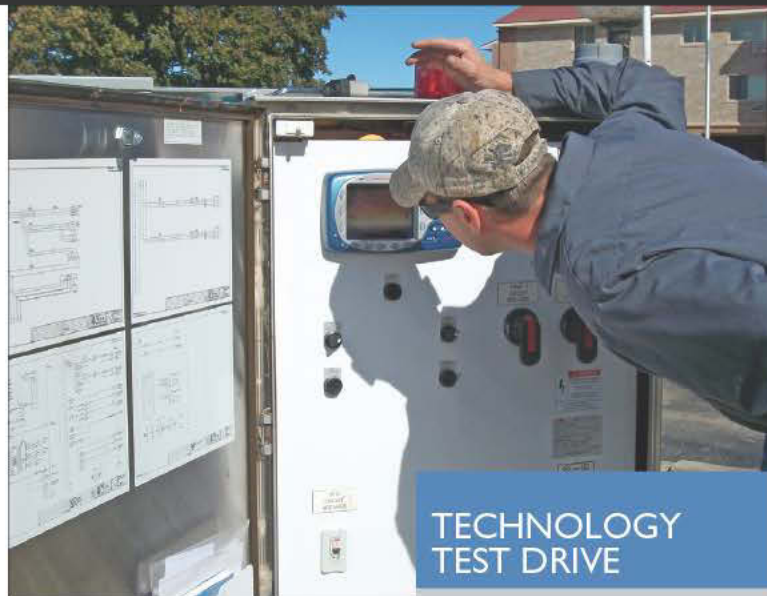
Travis Walker of the City of Beaver Dam shows the operation of the MultiSmart unit that operates a lift station. (Photography by Matt Gunn)
