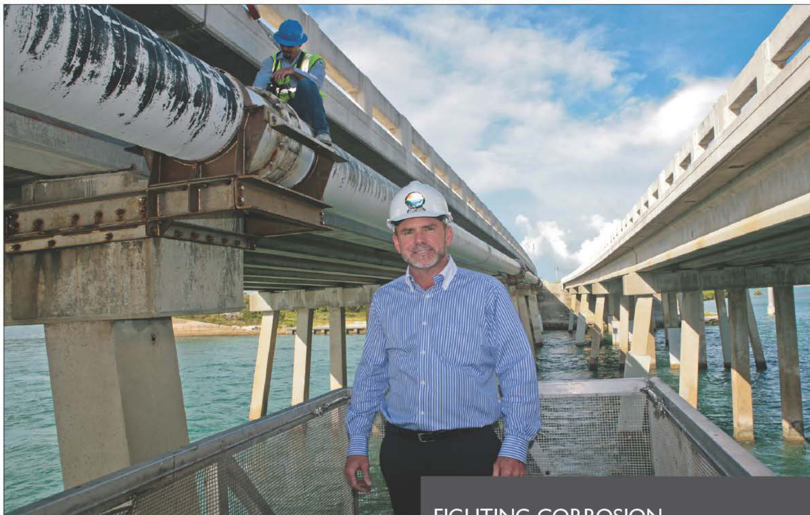
FCAA operations director Roy Coley stands in the lift while Aaron Sipe, distribution system operator B, works on a pipeline hung from a bridge.
