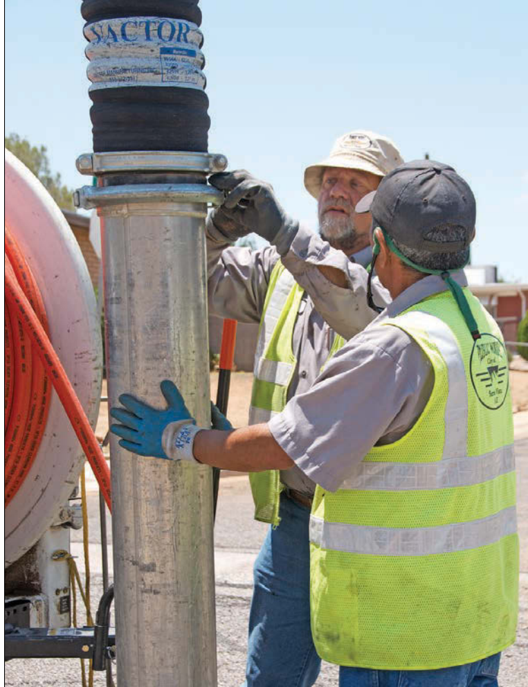
Jet rodder assistants Dan Lewis, left, and David Martinez assemble tubing on the Vector truck for cleaning a section of sewer line.
