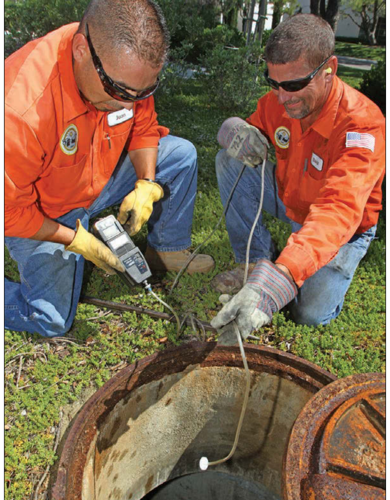
David Davis, right, and Juan Jaime lower a sensor from Industrial Scientific to measure levels of oxygen and carbon dioxide inside of a cistern, a central collection system for final filtration of stormwater before it enters a natural drainage channel.
