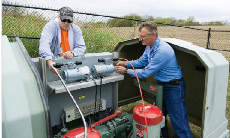
James Haynes and Tony Leighton do routine maintenance on one of Olathe's 18 Smith & Loveless lift stations. The collections system has 22 lift stations total.
