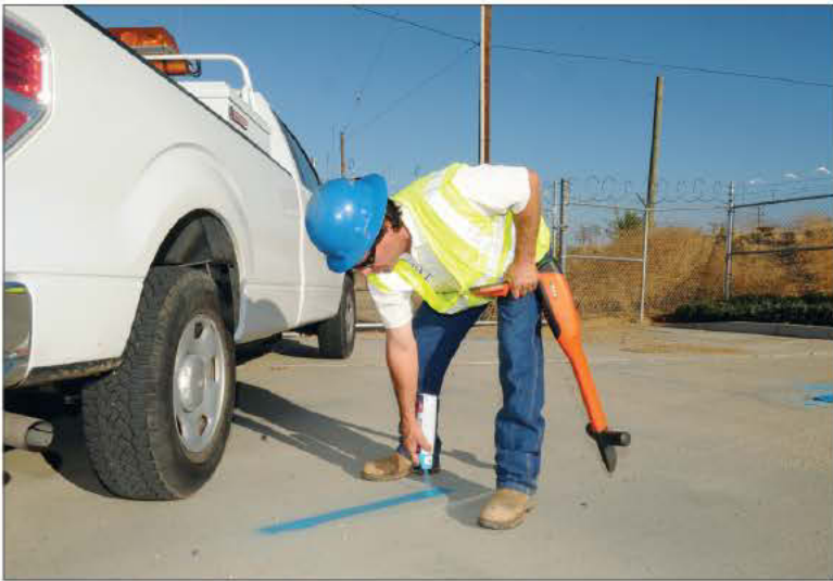
Bob Frosheiser, operations technician IV, marks pipe locations for USA DigAlert with a Vivax-Metrotech 810 locator.
