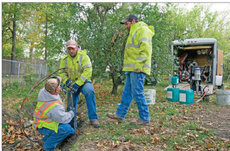
From left, Denton Lewis, Ira Speer and Chris Dankenbring use Prime Resins' Prime Flex Hydro Gel SX to seal leaking joints in a sanitary sewer line buried about four feet deep.
