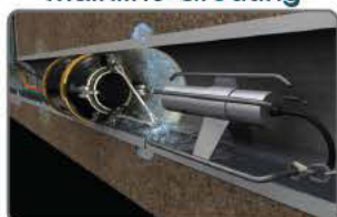
Leaking joint in mainline sewer
