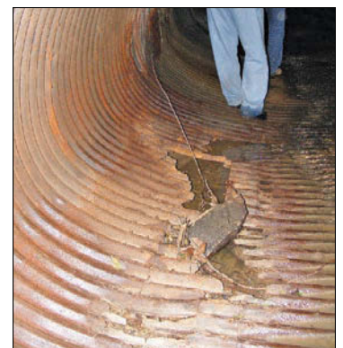
Initial inspection of the culvert revealed severe corrosion and structural failure.
