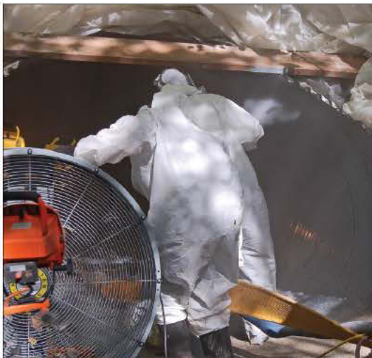
Proper personal protective equipment is vital to employee safety during PolySpray application.
