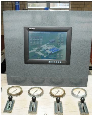
The new SCADA filter control panel from Southern Flow at the Livingston Water Treatment Plant.
