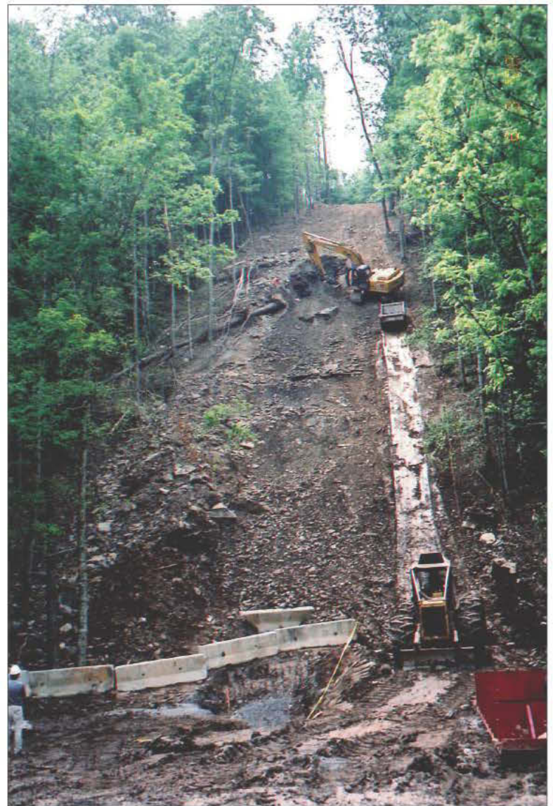
The crew handles the tedious task of running the new pipeline up a steep incline after a creek crossing.
