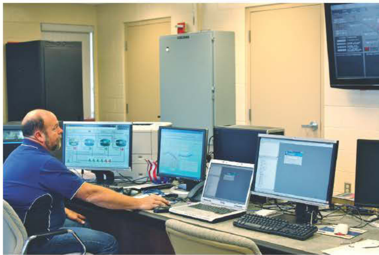
Controller Art Sheridan configures and tests graphics and objects in Wonderware (Invensys Operations Management), in preparation for roll-out at a new area of the facility. (Photography by Kimberly Lemma)
