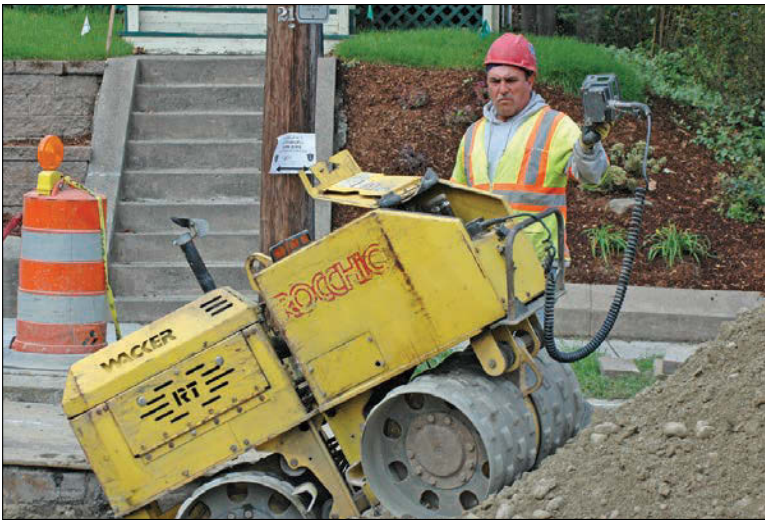
Laborer Francisco Arruda uses the Wacker Neuson vibratory trench roller to compact soil.
