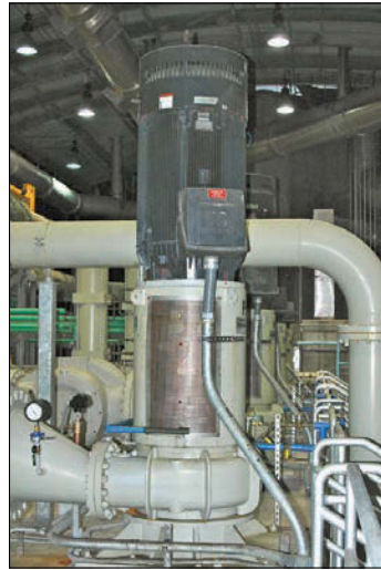
When the rain stops and the flow to the treatment plant drops below 65 mgd, crews turn on one set of pumps stationed 300 feet underground to pump out the stored stormwater and sewage from the tunnel at a rate of 12 mgd, sending it to the treatment plant for complete treatment (US Motors pumps, Siemens Water Technologies).
