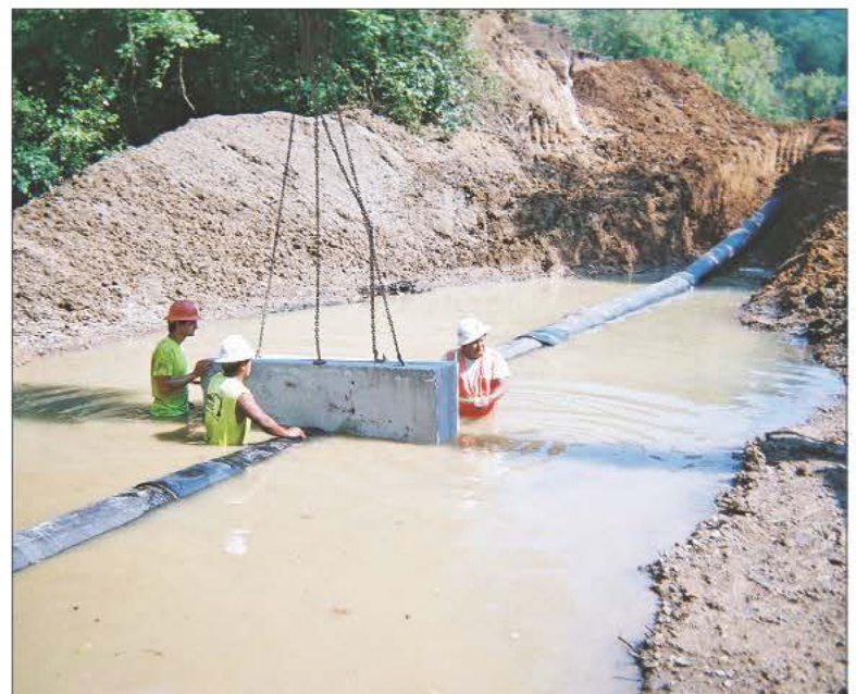
A temporary construction dam in Dry Fork Creek aided in the first of seven creek crossings but didn’t keep construction workers dry.
