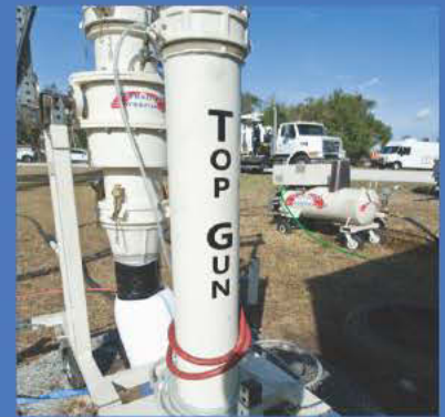
Perma-Main™ Continuous Air Inversion
