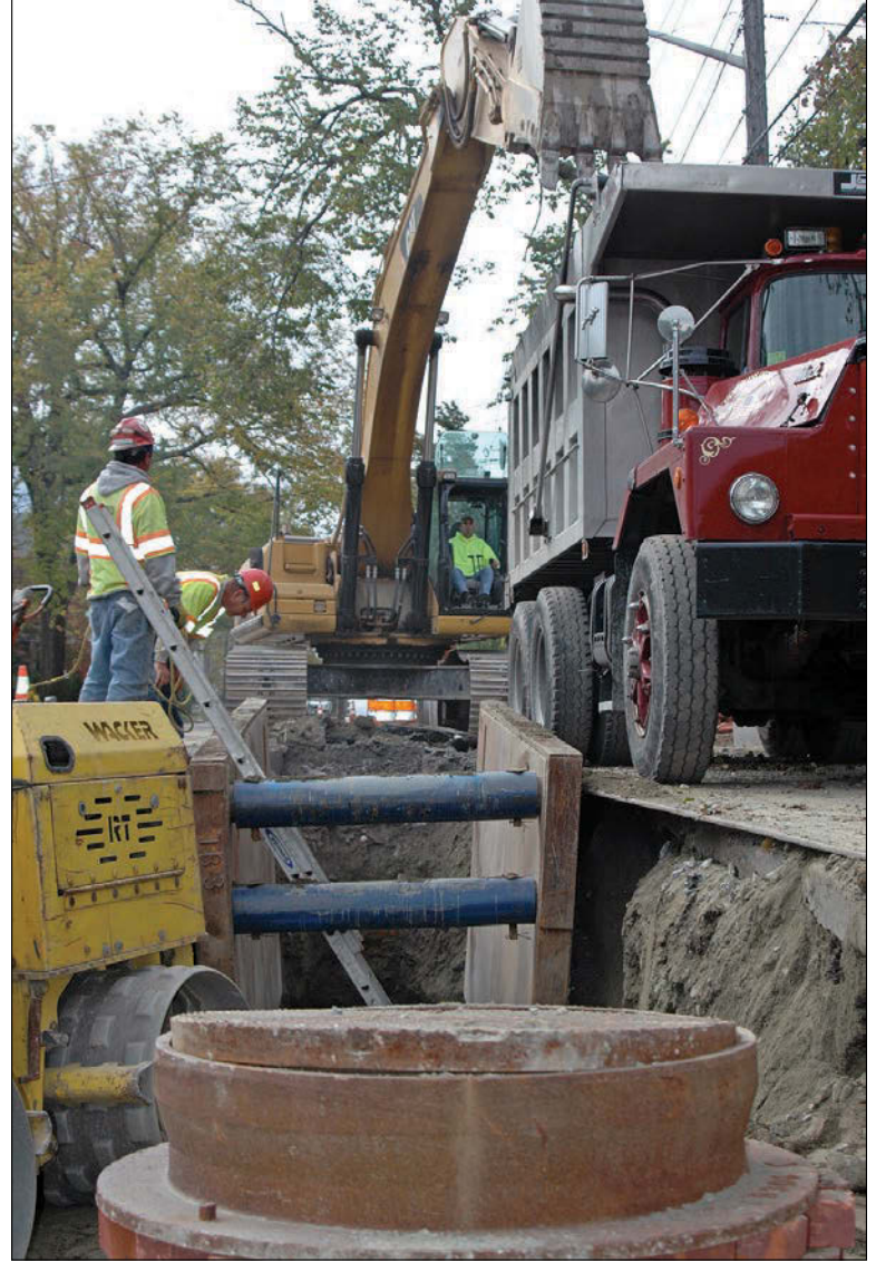
Laborer Francisco Arruda, foreman Antonio Duarte and equipment operator Richard Molis Jr. dig a trench to install storm sewers as a part of Phase 2 of the CSO project.
