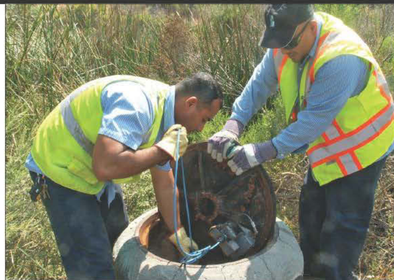
Field service technician Mauricio Avalos, left, and field service supervisor Marvin Gonzalez install a SmartCover monitor from Hadronex.
