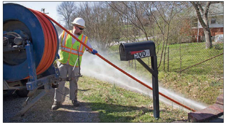
Stormwater crew member James Madden cleans a culvert, part of the routine maintenance schedule. The crew uses a Vac-Con truck and blasting heads to blow out sand, gravel and debris. Then a large vacuum attachment is used to suck up the debris that was blown from the culvert.
