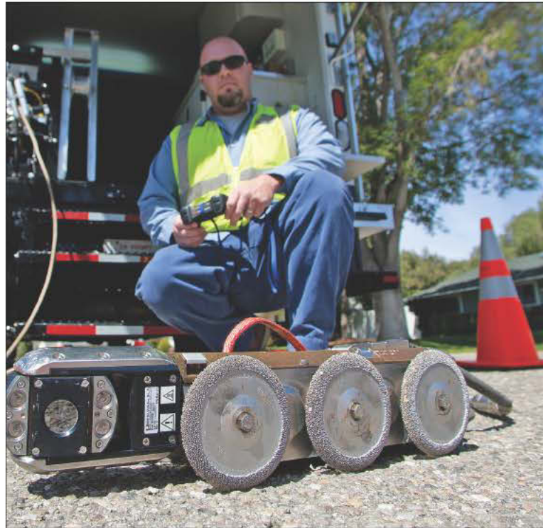
Jason Vollmer operates an OZIII camera-equipped Compact Pipe Ranger from CUES.
