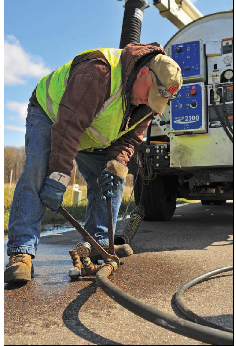
Tony Sterling disconnects a hose after flushing an air relief valve on a pressure system in a Stevens Point subdivision.
