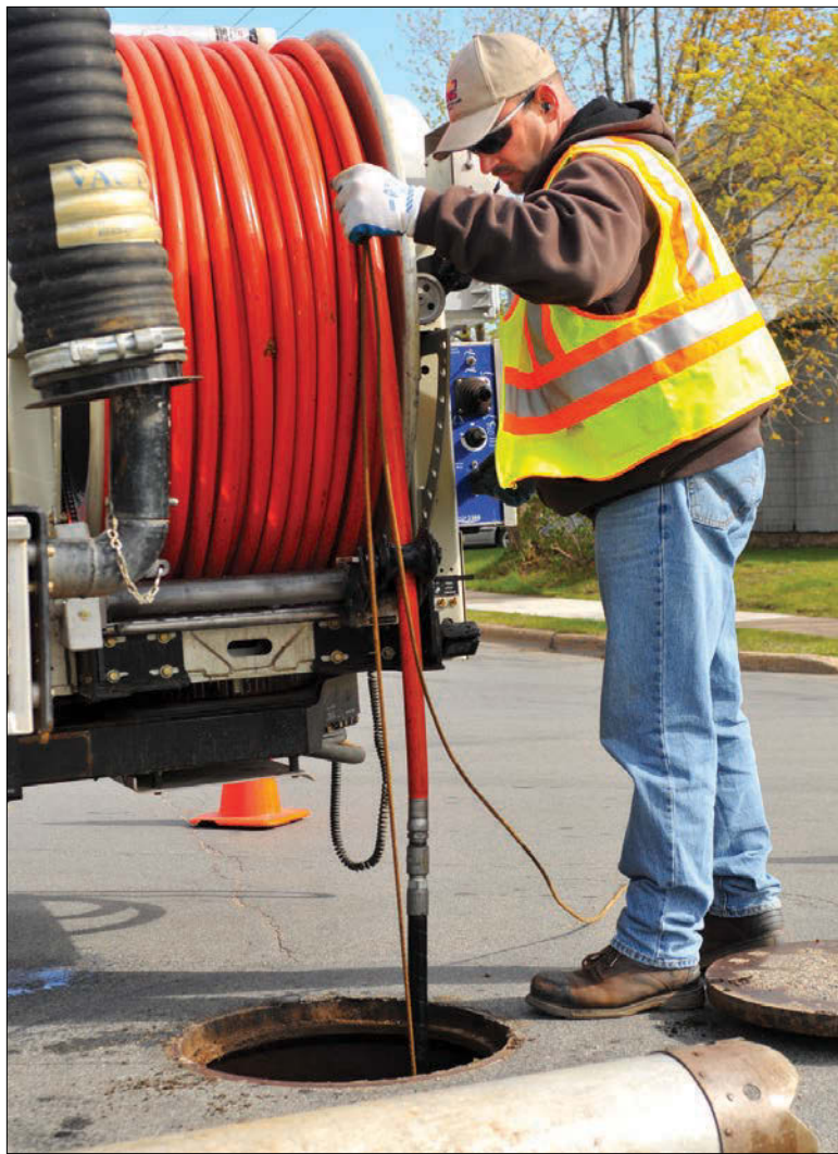
Dan Woitczak guides the jetter hose from the department's Vector 2100 down a manhole to begin cleaning the sewer main.
