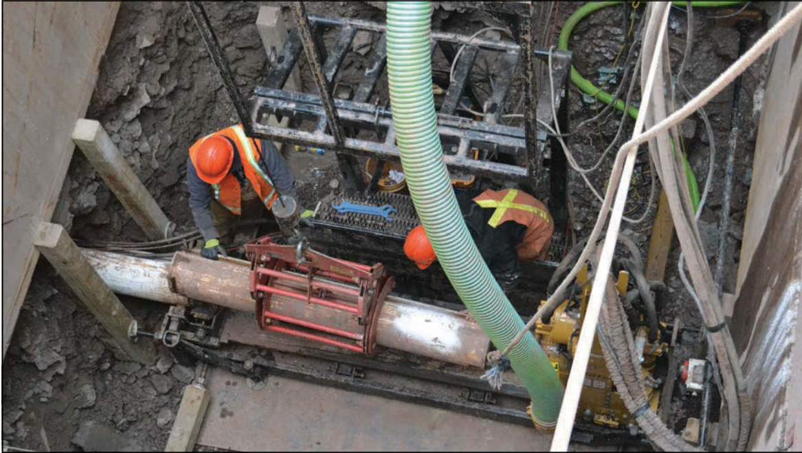
Workers maneuver a casing — still in the crane's claws — into place on the rack as it's lowered into the pit.
