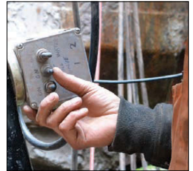
The controls on the unit are very simple.
