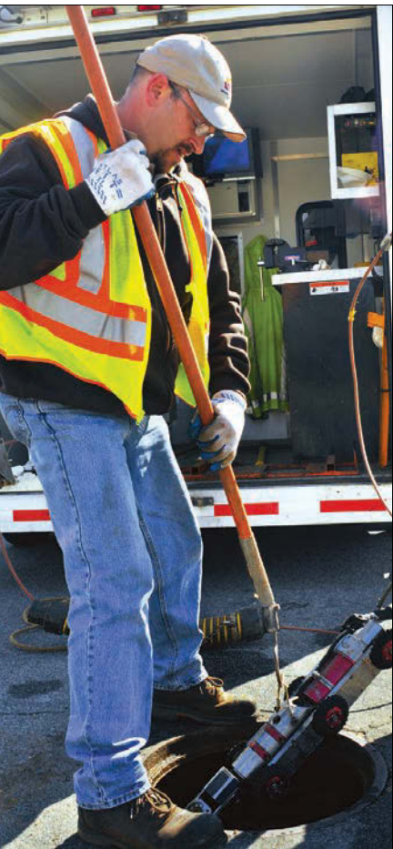
Dan Woitczak lowers the Aries camera and transporter down a manhole before inspecting a section of mainline sewer.
