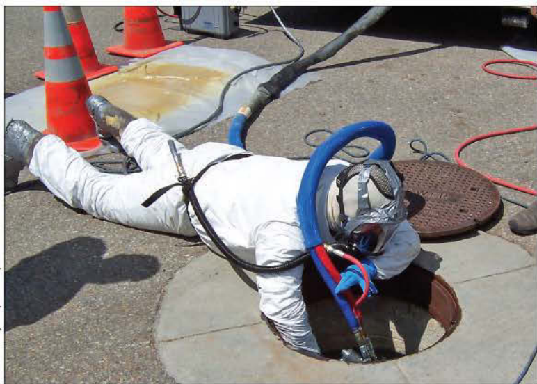
Cody Aberasturi of Pipeline Inspection Services uses SprayWall spray-applied polyurethane coating from Sprayroq to rehabilitate an existing manhole.
