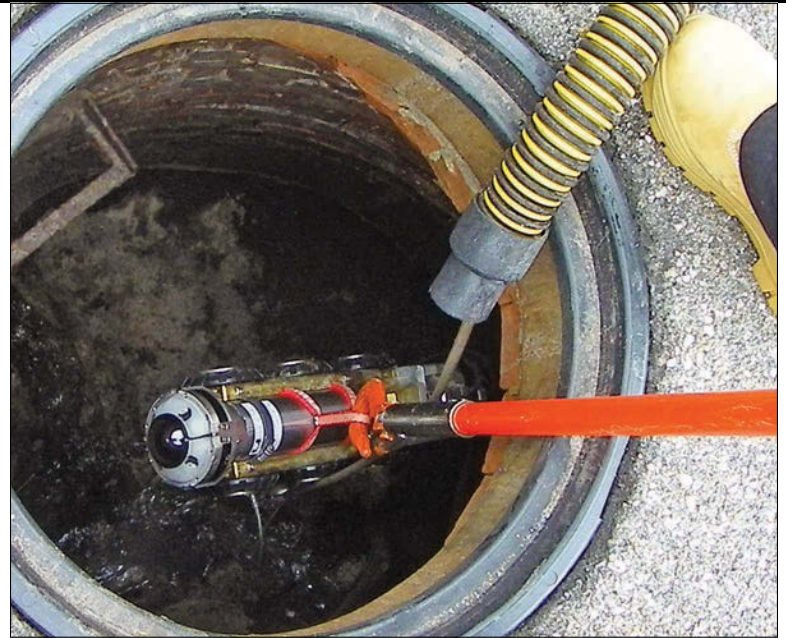
The transporter and DUC are being lowered into the manhole using a standard CUES introduction pole.
