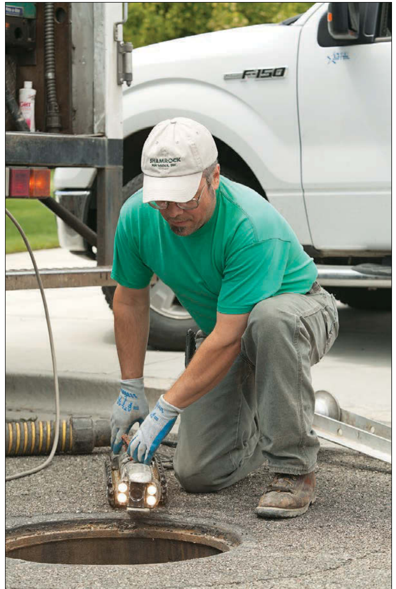
Chris Wilson of Pipeline Inspection Services prepares to send a CUES inspection camera into a sewer main.
