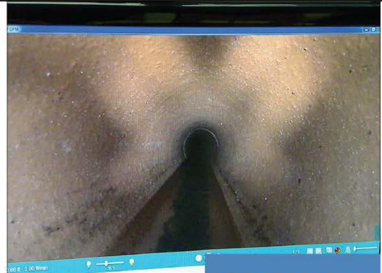
A "down the line" view of an 8-inch vitrified clay pipe created by the Granite XP software stitching successive individual "still" images into a continuous virtual movie of the traverse. (Photography by Gil Longwell)
