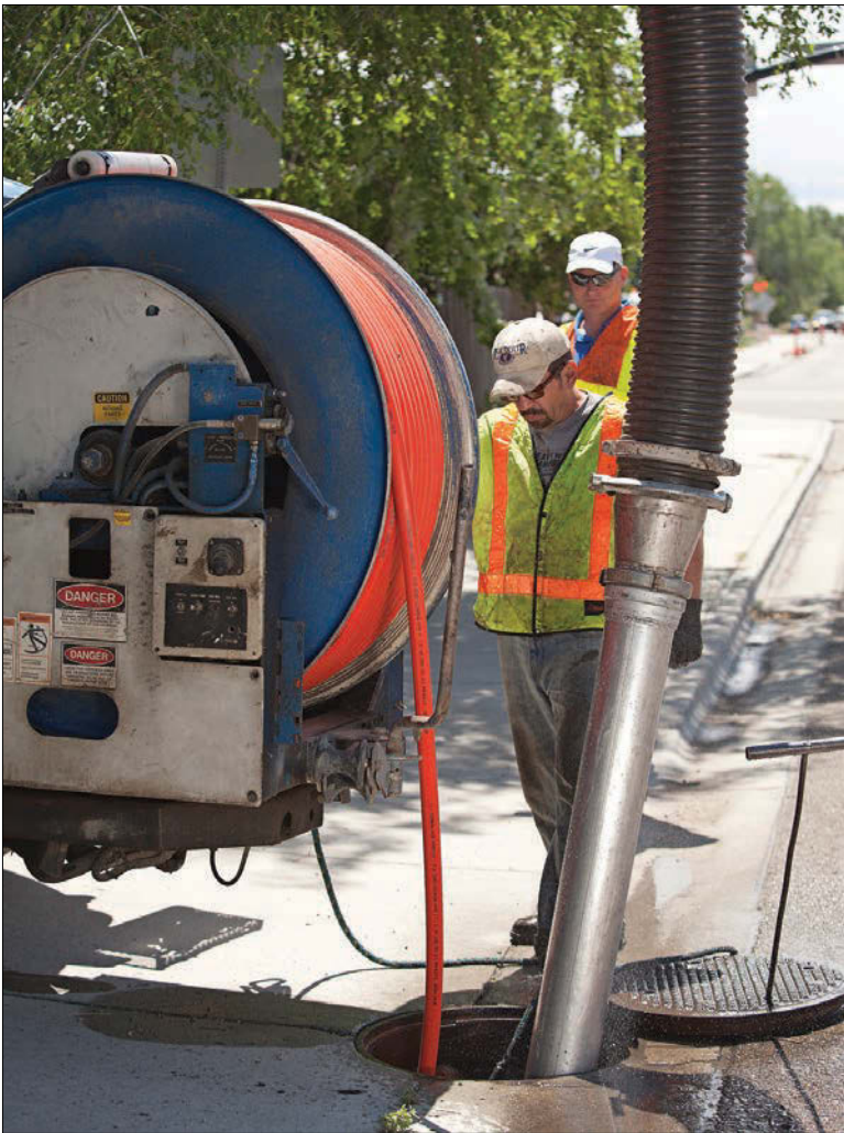
Hydroexcavator operator Robert Dunfee of Pipeline Inspection Services operates the Vactor 2115 combination sewer cleaning unit while Pipeline Inspection Services president Darin Barnes supervises.
