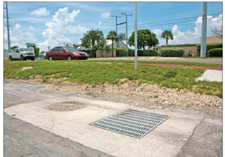
Injection wells are part of the citywide stormwater management system.
