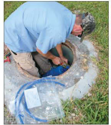
U.S. Water collection system technician Heath Townsend installs a valve in a vacuum pit.
