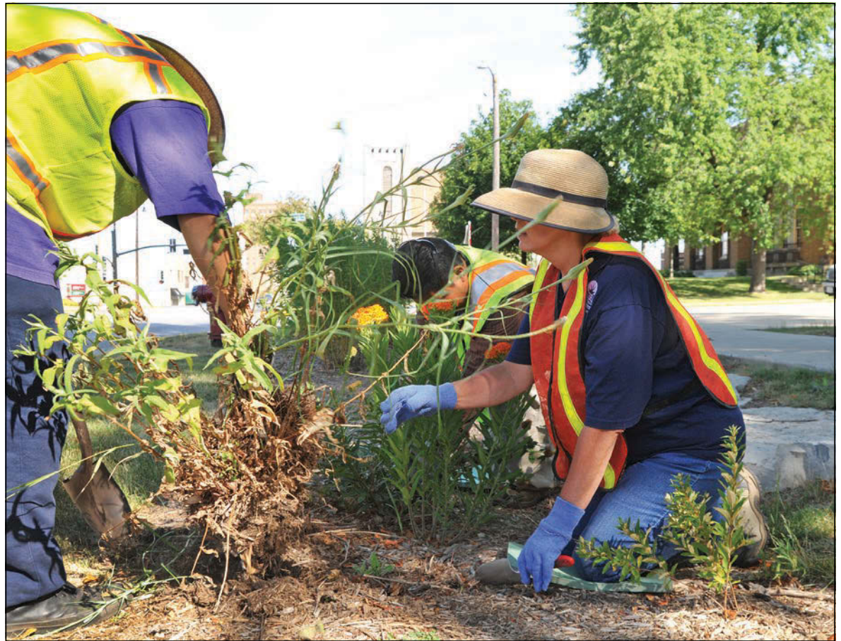
City of Aurora personnel maintain a green drainage area along a city street.
