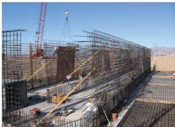
The Lake Havasu team reinforces bars for an aeration basin at the North Regional WWTP.
