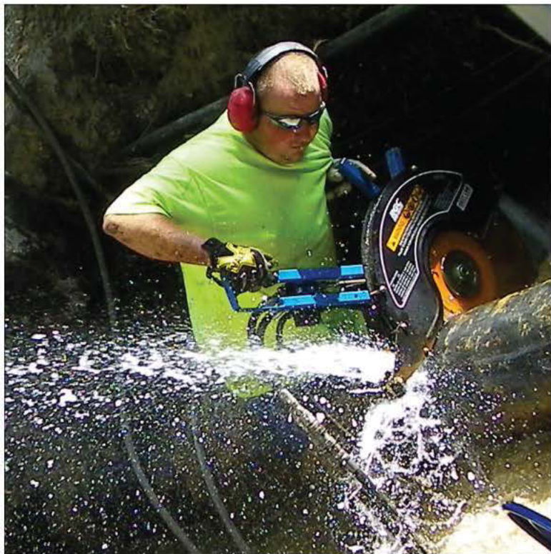
Bellefonte Water and Sewer Department crew member Brett Meyer uses a hydraulically powered circular saw to cut out a section of the old water main to gain access for the repair work.
