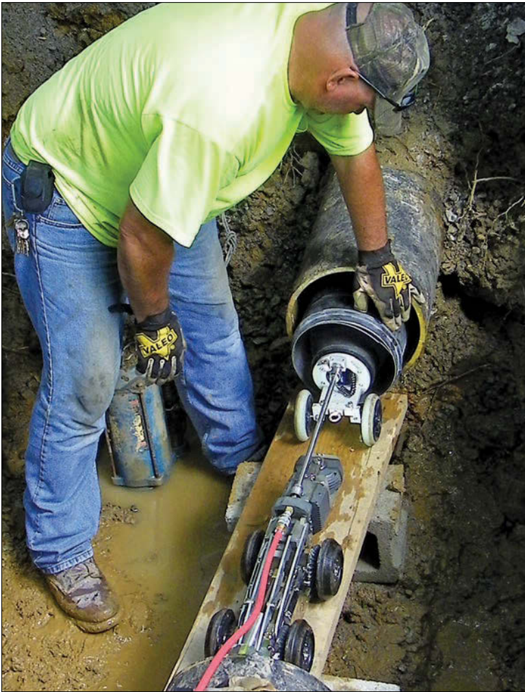
Bellefonte Water and Sewer Department crew member Dave Kleinfelter holds the sleeve in position as the operator inflates (expands) the bladder. The packer, pushrod, tractor, control cable and air hose are all visible. The train is supported on the temporary work platform.
