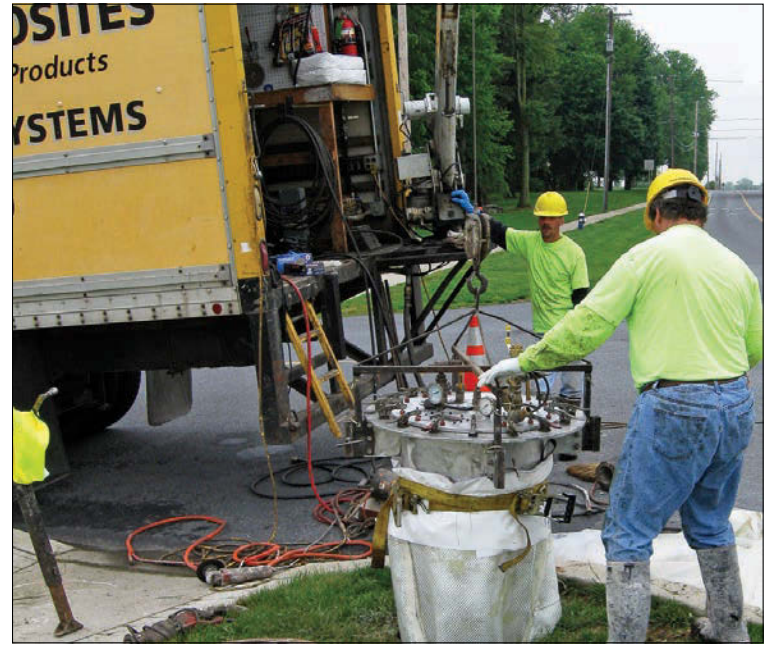
Terry Smith from Terre Hill Composites operates the crane as Bill Kissinger helps guide the liner into the manhole.
