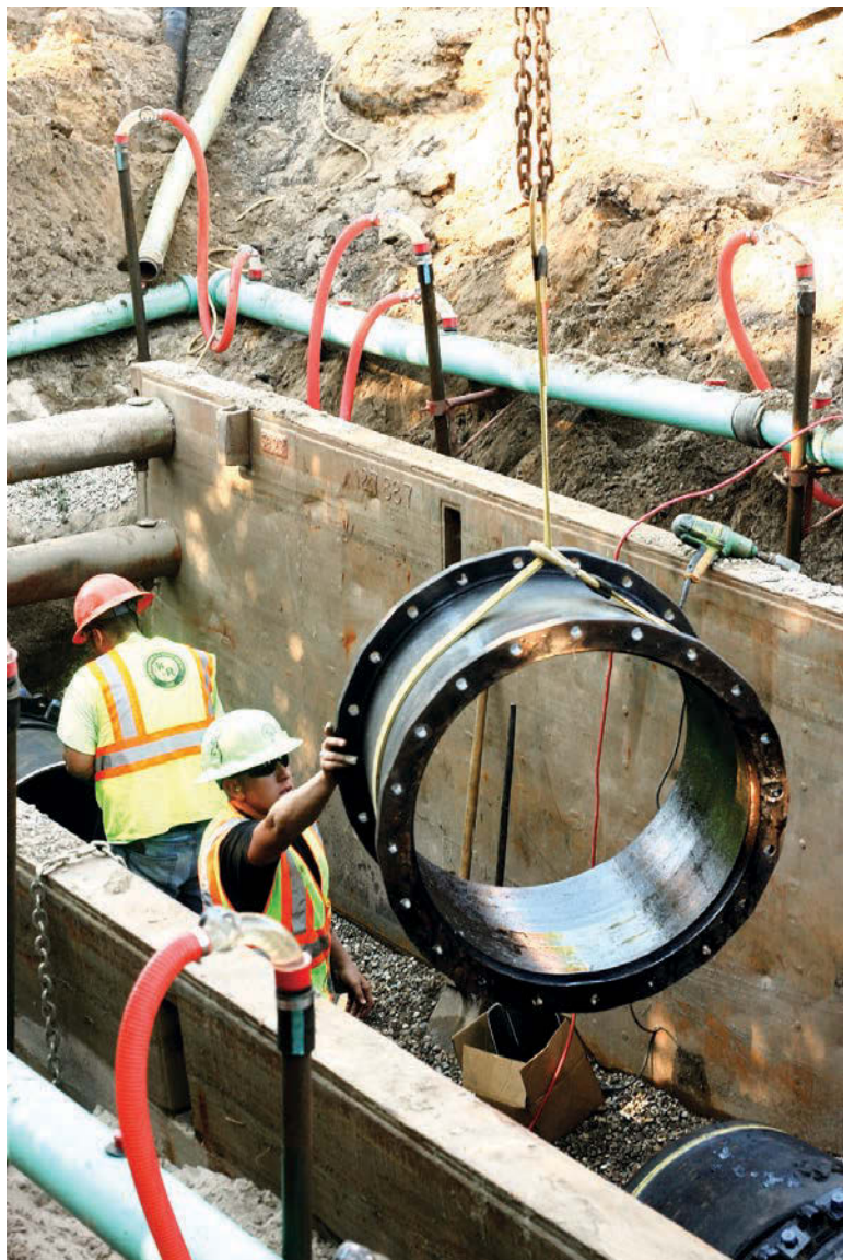
K&R crew members Craig Schram, right, and Carlos Gonzalez guide a 30-inch sleeve into the trench and prepare the pipe for tie-in.
