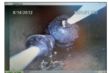
This push camera image shows the probe up at the inflatable plug. This is where the scan will start. The camera will be removed, water put in the pipe, and then the probe will be withdrawn through the water as it completes its scan.
