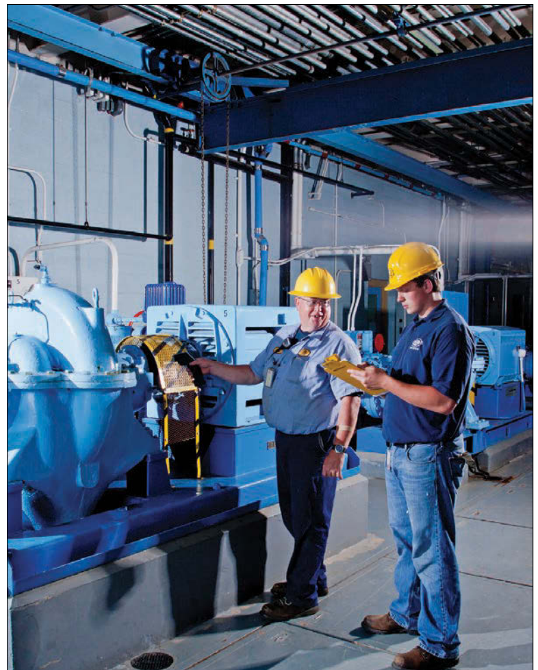
Dave Broene, water treatment maintenance worker, left, reviews a preventive maintenance checklist with Braden Scharlow, water treatment intern, on one of the high-service centrifugal pumps.
