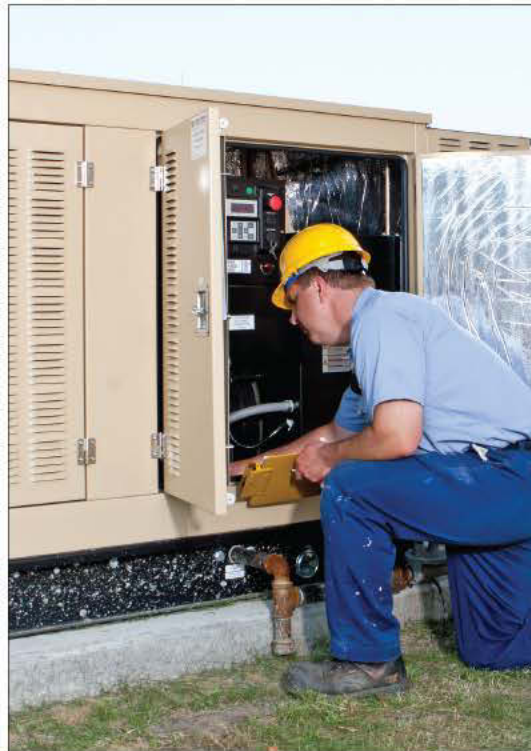
Ross Devries, lead water plant maintenance worker, performs routine maintenance on the new Generac generator.
