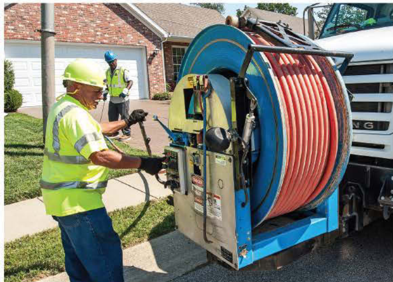
Operator Mike Maggard uses the Vector hydroexcavator to flush a secondary sewer line prior to TV inspections.
