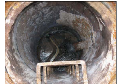
Corrosion and missing mortar in Lower Frederick Township manholes allowed 40,000 gpd or more of inflow and infiltration to reach the 200,000 gpd (design) sewage treatment plant.
