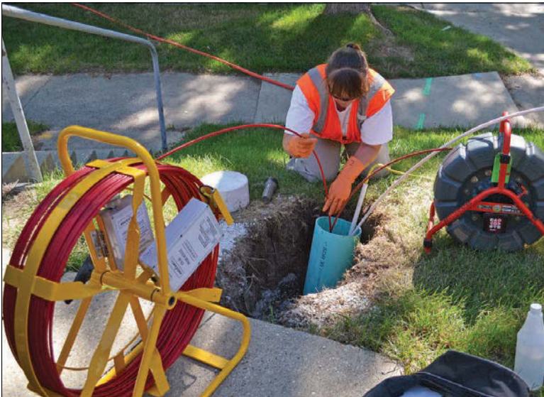
Elizabeth Gruell of Brown and Caldwell inserts the probe into the lateral via the cleanout, pushing it to the end of the section of pipe to be scanned.
