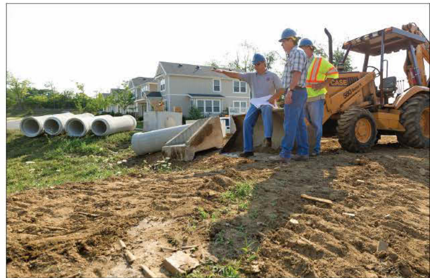
Charles Martin, left, Bill Warren and Jeff Baumgardner review construction drawings for the Anniston-Wickland stormwater project (pipe manufactured by Sherman-Dixie).
