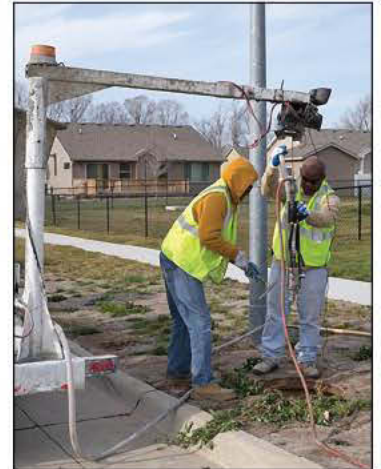
Lenny Terrell, left, and Stan Lamay prepare the PermaCast system for a manhole rehabilitation.
