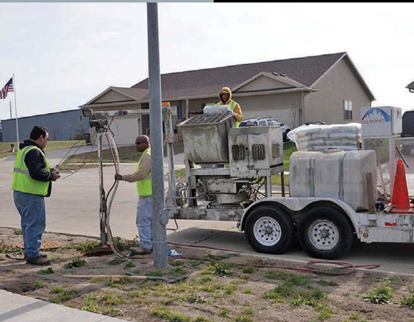
City of Des Moines manhole restoration crew members Albert Salazar, left, and Stan Lamay lower the AP/M PERMAFORM PermaCast system into a manhole while Lenny Terrell mixes grout on the trailer. The city has a dedicated PermaCast trailer outfitted with all the necessary equipment for their work. (Photos courtesy of Linda Keairns)
