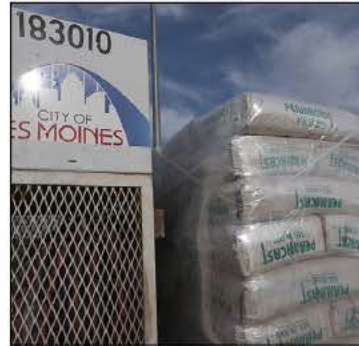
A pallet of PermaCast MS-10,000 grout mix rests on the City of Des Moines' manhole restoration trailer.
