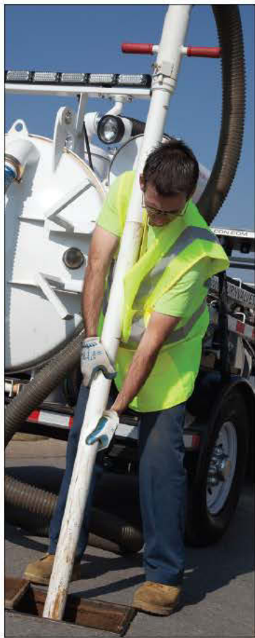
Valve technician Nash Dent from Mueller Service Co. uses the E.H. Wachs Trav-L-Vac to clean a valve box.
