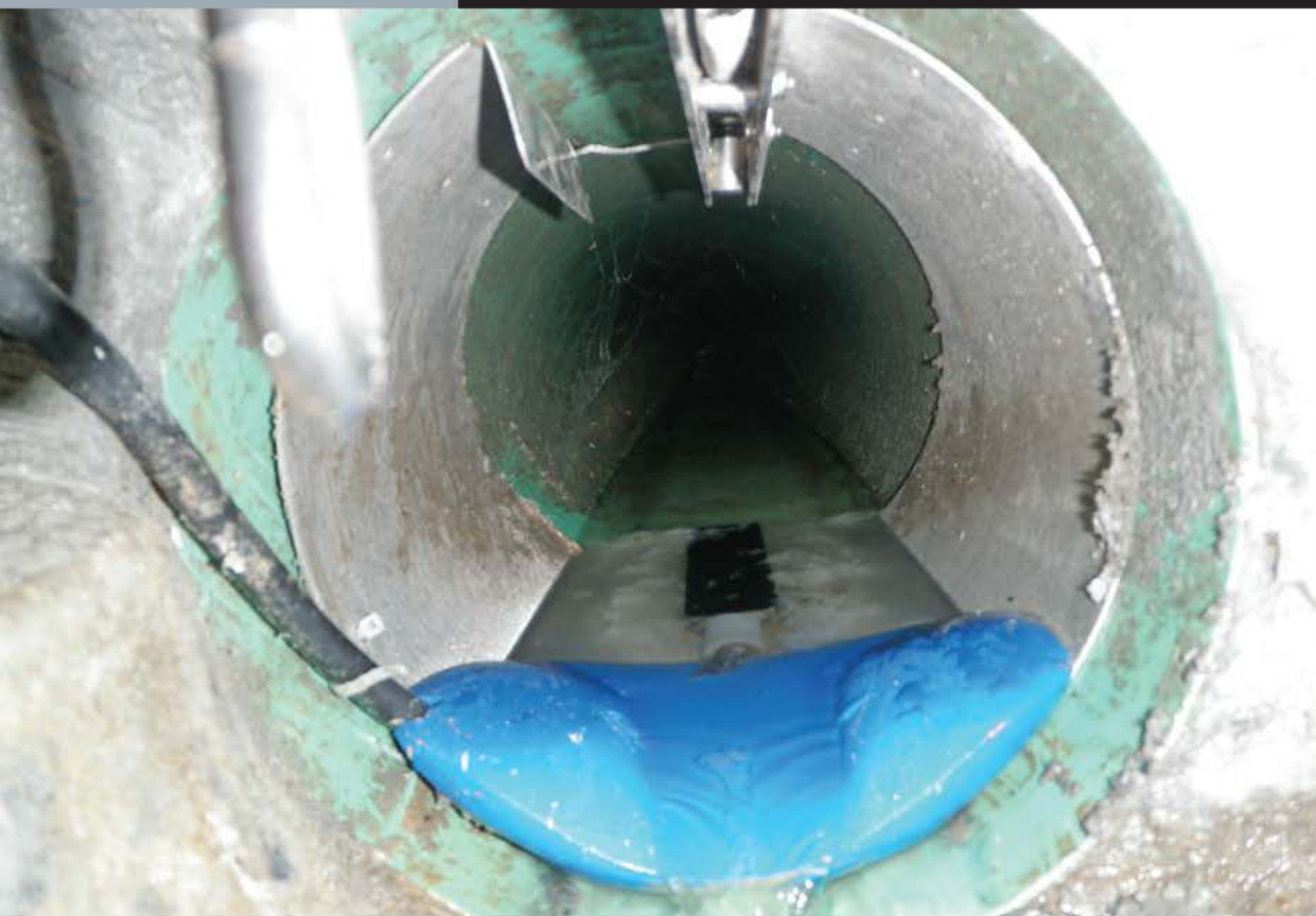
The Stantec Micromonitor, installed here in a sewer line, is a modified version of a standard area-velocity flow probe with the addition of a fabricated fiberglass weir insert installed behind the probe on a single stainless ring. (Photos courtesy of Stantec Consulting Services)
