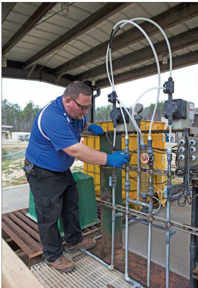
Kai Vannoy checks a 12-inch Badger Magnetoflow meter at the Holly Springs water reclamation facility.
