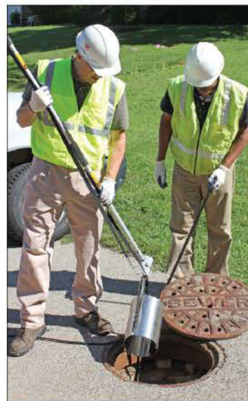
Stantec senior associate John Barton, left, and engineering team leader Joseph Kamalesh begin installation.
