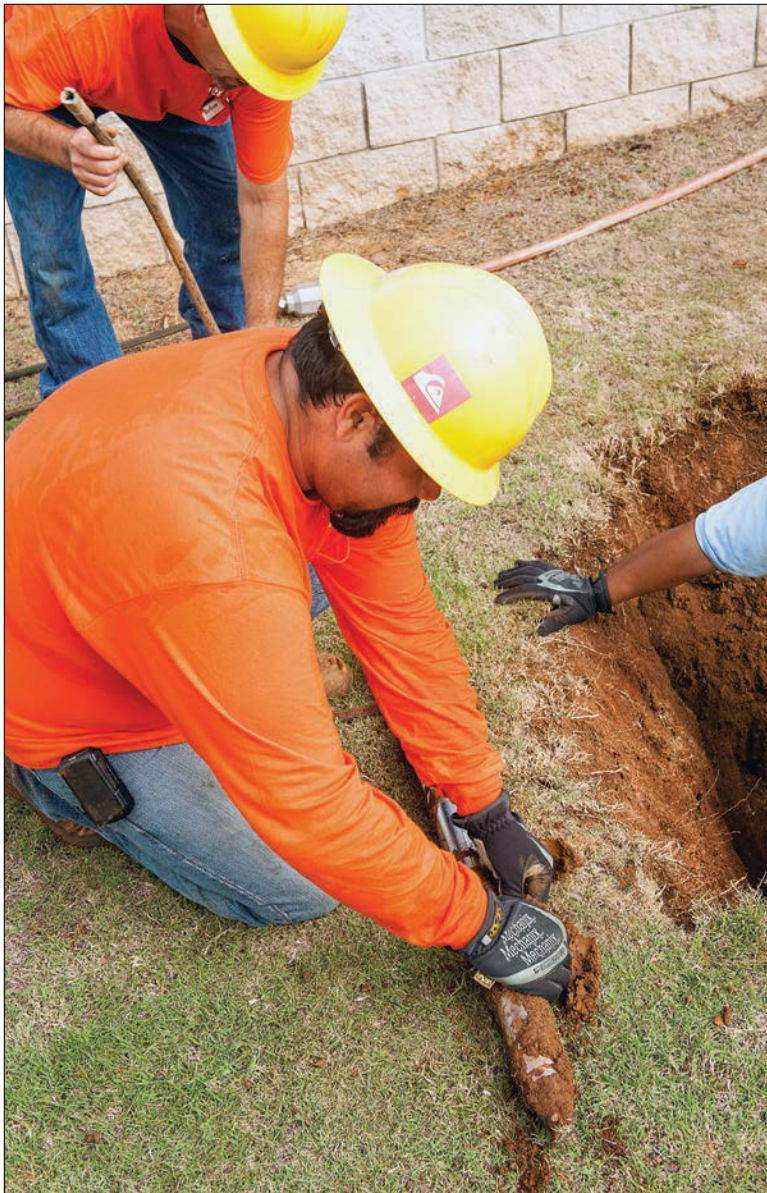
Jeffery Silva (foreground) and Corey Silva clean caked red Kauai dirt off a Grundomat horizontal boring tool (TT Technologies).
