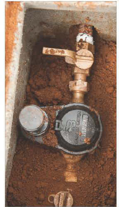
A newly installed water meter from Badger Meter.
