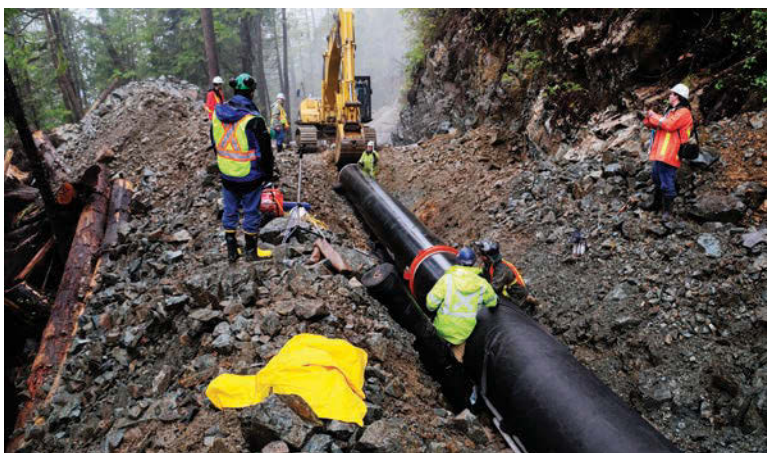
Inclement weather, difficult and uneven terrain, ground swell and landslides can create a variety of problems for installation crews, but grooved pipe's coupling system provides more flexibility at installation.
