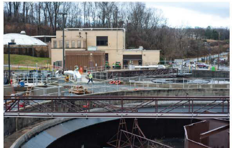
Upgrades have been made to the Lynchburg Regional Wastewater Treatment Plant in recent months, such as the secondary clarifiers. The headworks, primary clarifiers, aeration basins and return activation sludge system also were upgraded.
