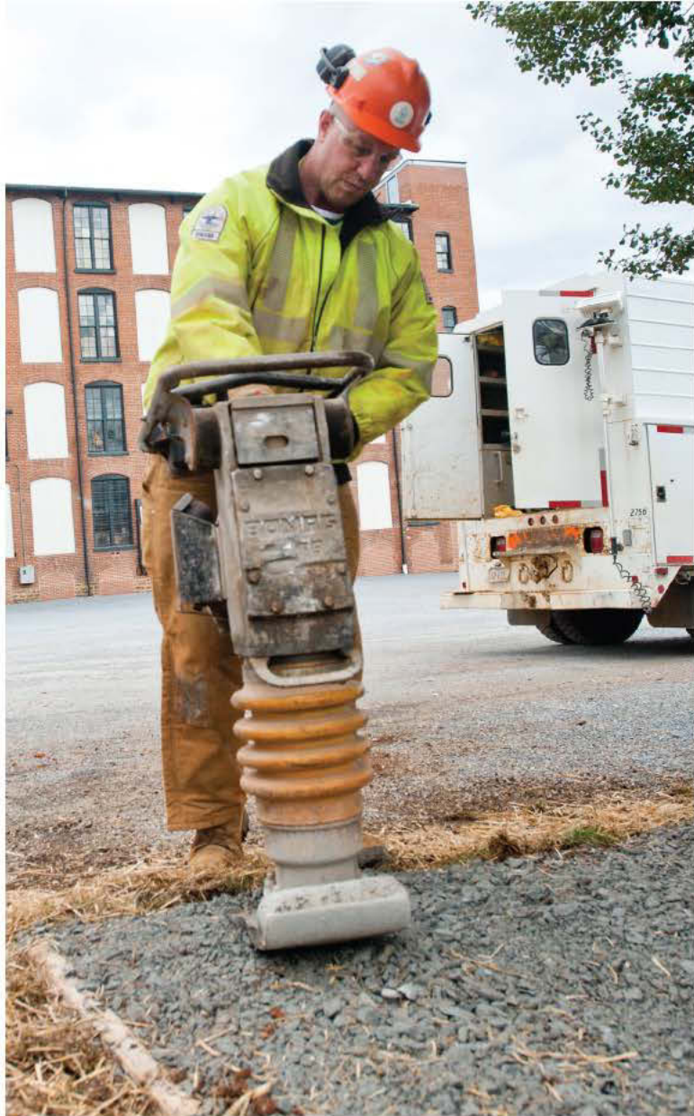
Scott Sablack, utility line tech 2, uses a tamper (BOMAG) to compact and flatten the surface after a water service renewal in Lynchburg.
