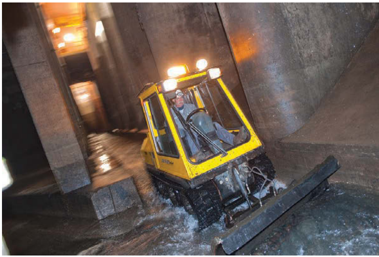
Pump mechanic Larry Mills operates a Bombardier SW48HY to squeegee debris off the floor of the intermediate structure of the underground concrete basin.
