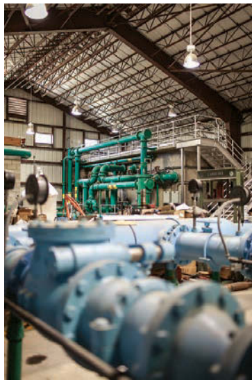
The Cedar Glen Water Treatment Plant doubles as the small community's offices and general storage facility.
