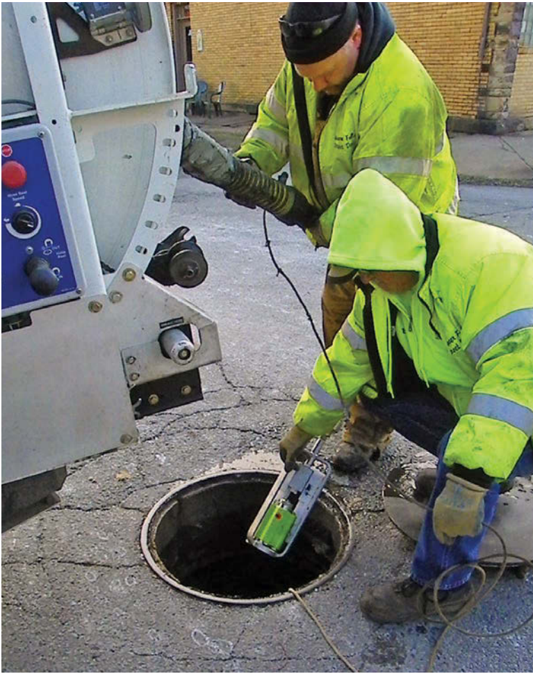
Beaver Falls Street Department crew members Bob Justisin (foreground) and Pat Burdine prepare to introduce the JetScan into the manhole.
