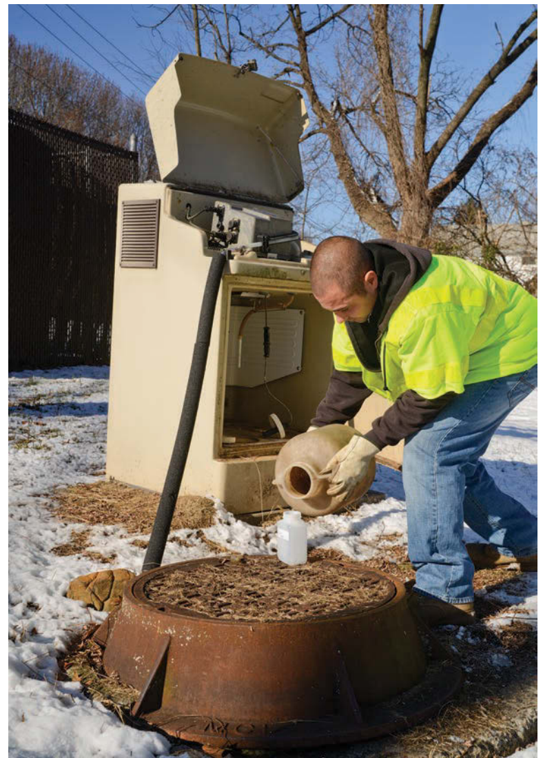
Steve Grosso takes a 24-hour composite sample at a meter chamber.
