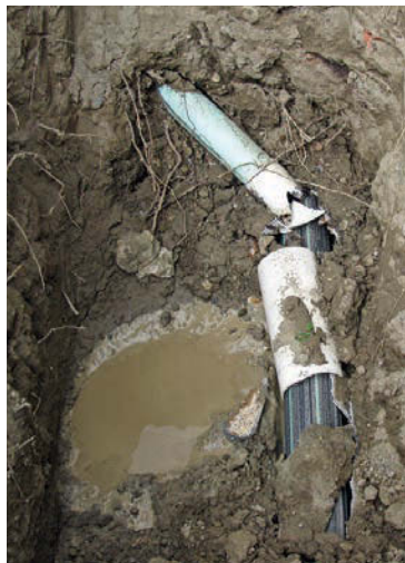
A new section of HDPE pipe is pulled through the existing PVC.
