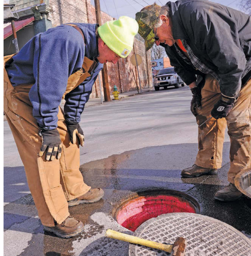
Town of Bell Buckle Wastewater Manager Randy Johnson, left, and Water Superintendent Ronnie Lockey look at a SpectraShield treated manhole.
