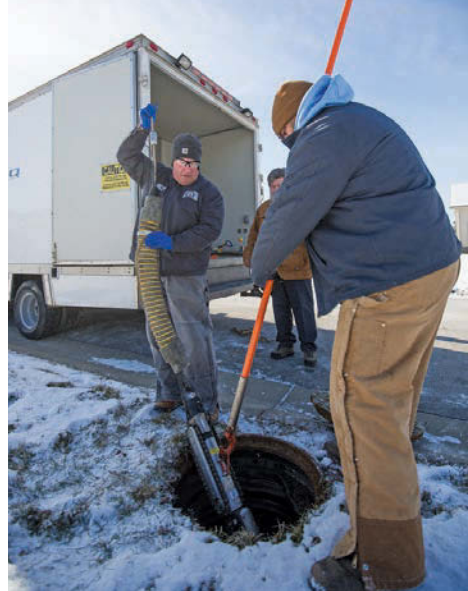
Pat Welch, left, and Rocky Price lower a CUES camera down the manhole for a sewer line inspection. RIGHT: A look at the control room in the CUES CCTV van.
