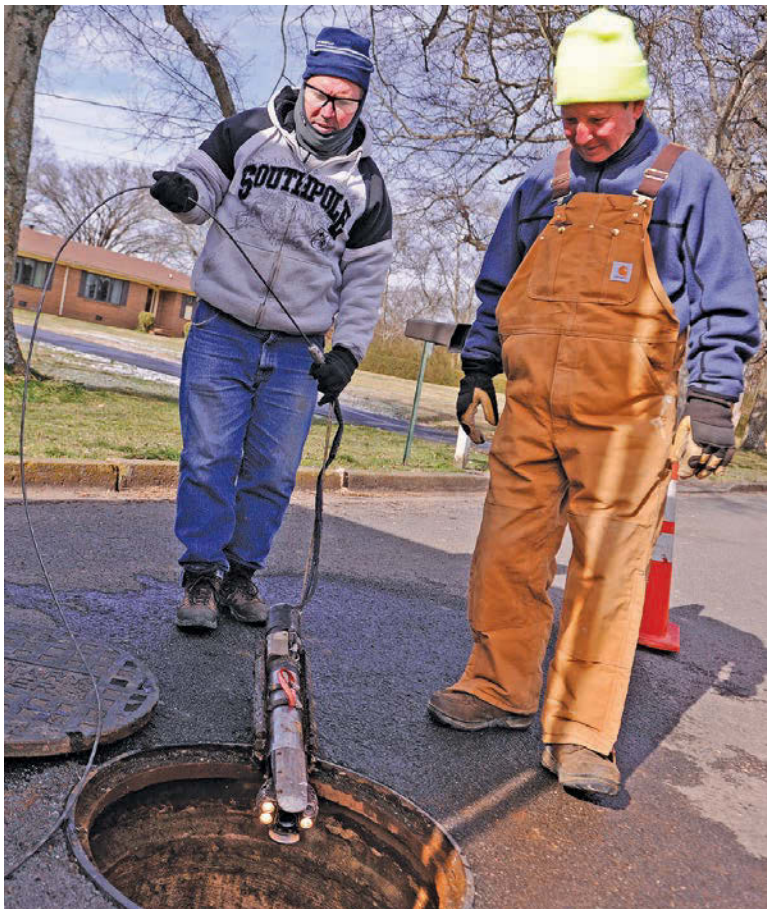
Town of Bell Buckle Wastewater Manager Randy Johnson, right, watches as a Compliance Enviro Systems worker retrieves a camera out of a manhole.
