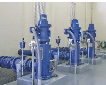
High service water pumps move water to the distributor at the Palm Bay Utilities Department.
