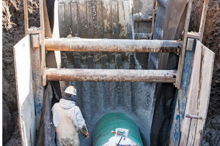
Gravel is brought in to backfill around the newly installed interceptor pipe.
