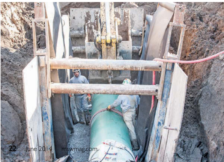
The Kissick Construction crew aligns a section of pipe deep in the Second Creek Interceptor trench.
