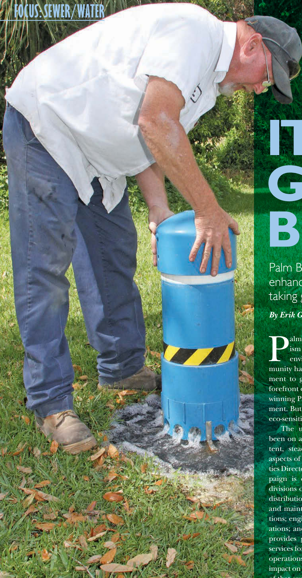
Jody Ballard, utility foreman, replaces the case of the automatic flushing device he made as it runs a cycle. (Photography by Keith Carson)
