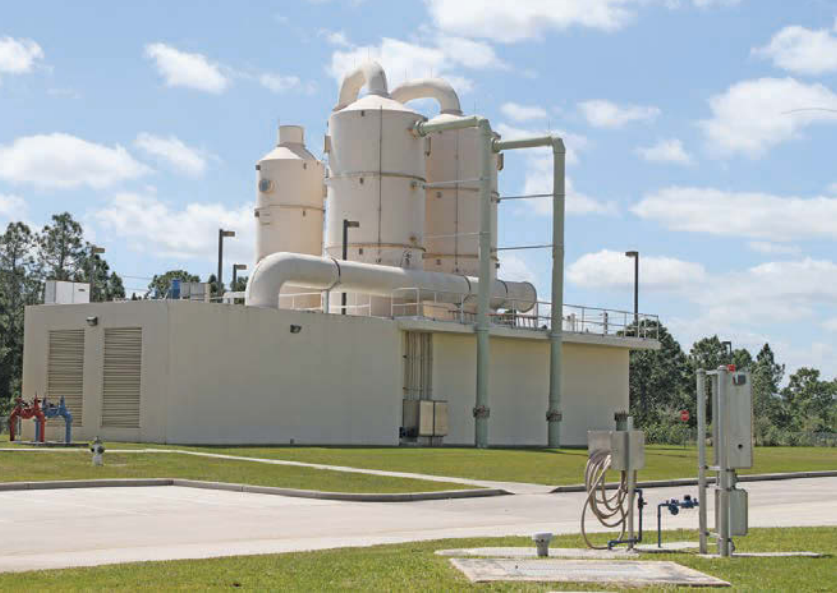
The degasifier at the Palm Bay Utilities Department takes the odor out of the water. Below: Palm Bay Utilities Department Director Dan Roberts stands above the department's reverse osmosis membranes.
