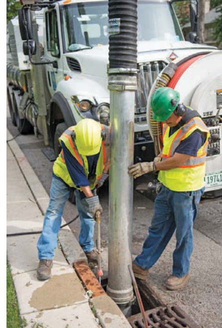
Danny Pingue (left) and Jaime Vega use a Vector jet/vac truck to clean a storm drain.
