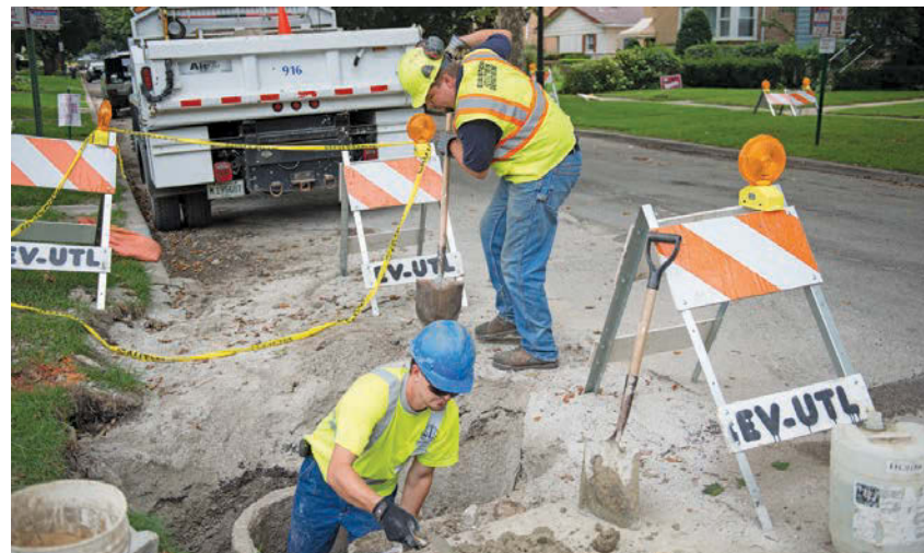
From top to bottom: Bob Bauer of the City of Evanston Utilities Department guides a camera through a mainline inspection using CUES equipment in the control room of the utility’s inspection van; Bernard Pamaran (left) and Bob Bauer lift the camera out of a manhole after the inspection; Danny Cullen, bottom, and Shawn Pestka make repairs to an inlet and catch basin along a residential street in Evanston.
