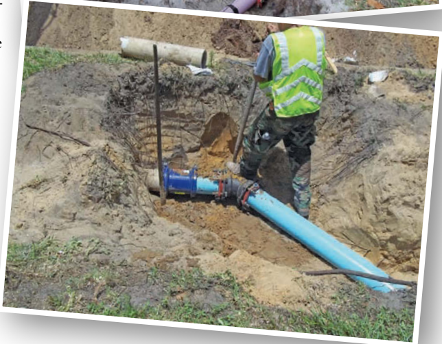
Crews from the City of Altamonte Springs Public Works and Utilities Department work on different pipe replacement projects in coordination with the Neighborhood Enhancement Program. (Photos courtesy City of Altamonte Springs)
