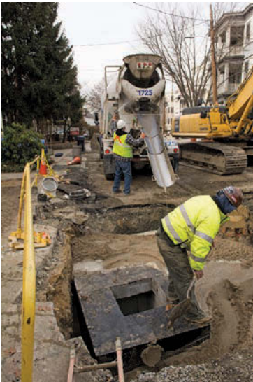
Construction on the Sewer Separation Project continues throughout the winter in Cambridge. Above left: Catherine Woodbury, engineering project coordinator for the Cambridge Department of Public Works at the Alewife Reservation Stormwater Wetland. Left: A mix of sand and a small amount of cement is used as fill and compaction material around a new sewer pipe.
