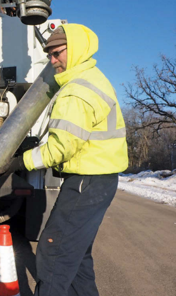
Public utilities service operator Joe Kachtinske attaches a vacuum tube to the boom of an Aquatech jet/vac truck while Keith Ruprecht stands at the truck's control panel.
