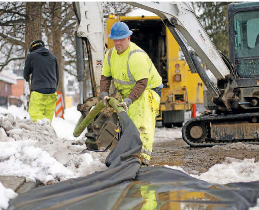
Top: Columbus Division of Water employee Tom Strejcek (in hole) works to fix a broken mainline at a home on Highland Street in Columbus, Ohio. Above: Jeff Boals pulls back a vacuum hose after repairing the broken waterline.
