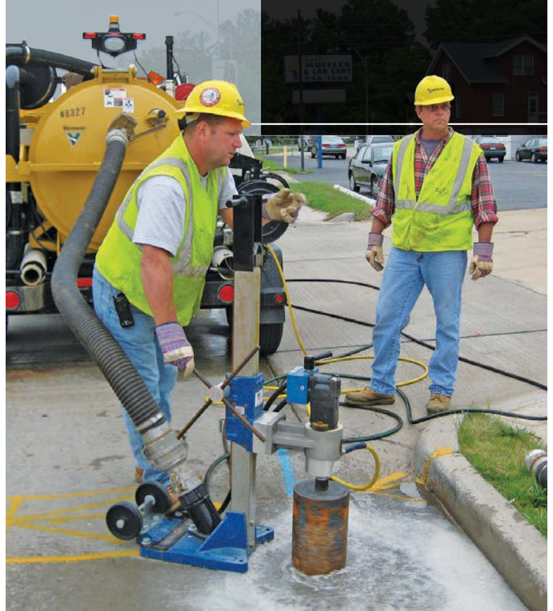
Workers use a core saw to open a hole in the street surface for a precise hydroexcavation job.
