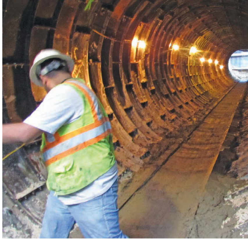
Left: When complete, the Tarrant Regional Water District's new water supply line will stretch across 150 miles of Texas countryside and connect the utility to four additional water sources. Above: A Tarrant Regional Water District construction crew member walks through the framework of a section of the new pipeline.
