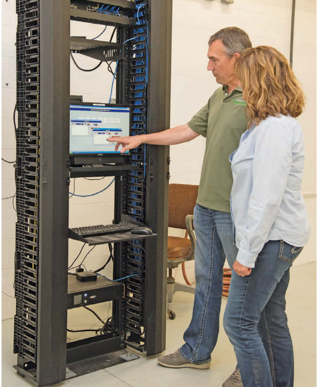
Technology Director Bruce Patterson and GIS specialist Carol Ellison check a monitoring system at the city’s water department.
