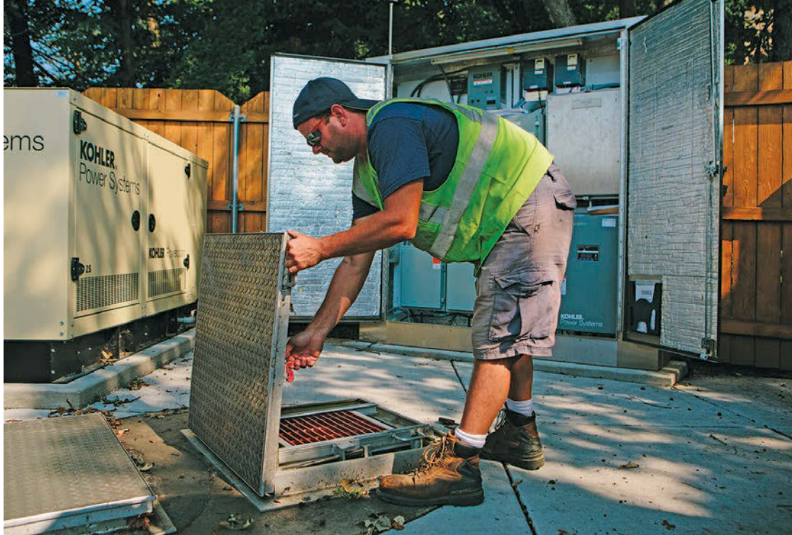
Utility technician Jamie Antich checks the Flow-Technics monitoring and control system at the Royce Road lift station in Naperville.
