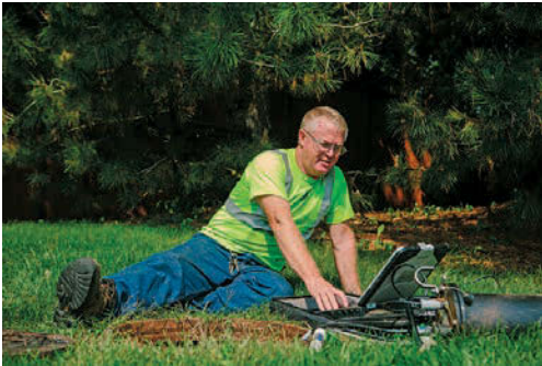
Top: Utility technician Wally Thome remotely drives and monitors an OZIII camera while inspecting a sewer line from the control room of the CUES TV truck. Bottom: Technician Terald Brue checks on a Triton Flow Shark (ADS Environmental Services) used to monitor flow conditions including depth, speed and temperature.
