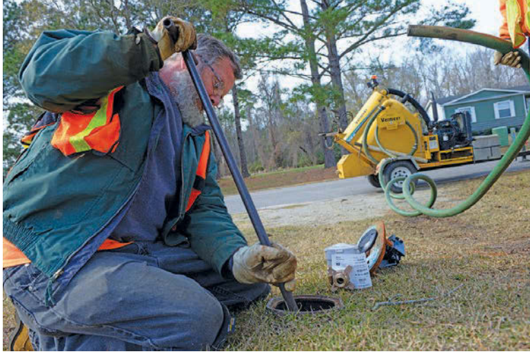
Meter technician Bill Schmidt preps a meter box for installation of a new water meter outfitted with a Sensus Smart Point transmitter.
