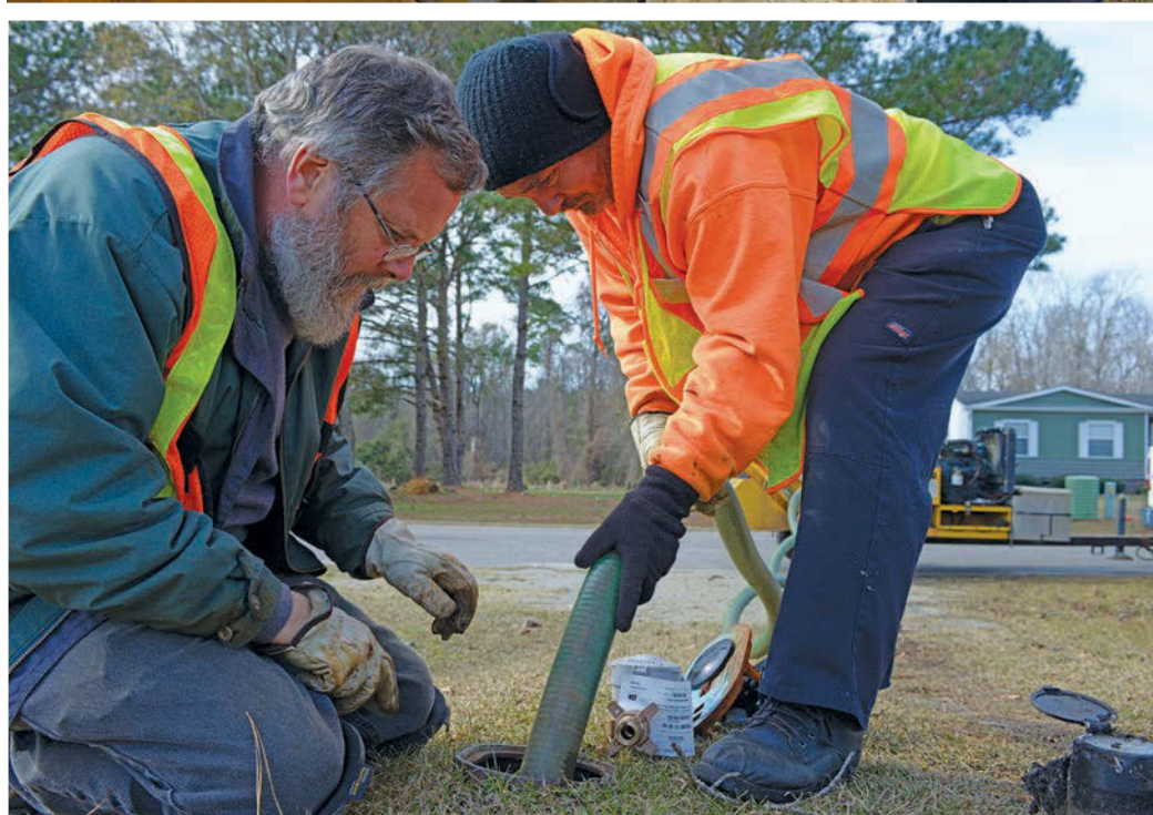
Meter technician Walter Trulove (top) wraps up the vacuum hose on a Vermeer FM 150 SDT after cleaning out a meter box for a new meter installation (above) with technician Bill Schmidt.
