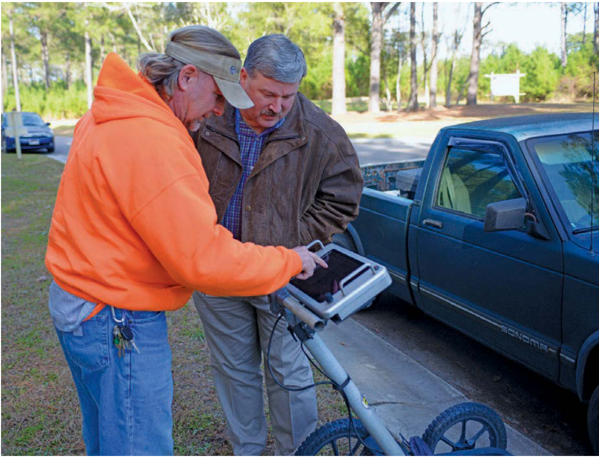
Brunswick County Utility Foreman Robert Horn (left) discusses results of scans from the MALA ground-penetrating radar with Water Distribution Superintendent Bob Tweedy.
